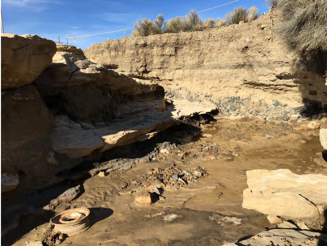
5. EXISTING JETTY EXPOSED IN THE EROSIONAL FLOW PATHWAY, PARALLEL TO JETTY
