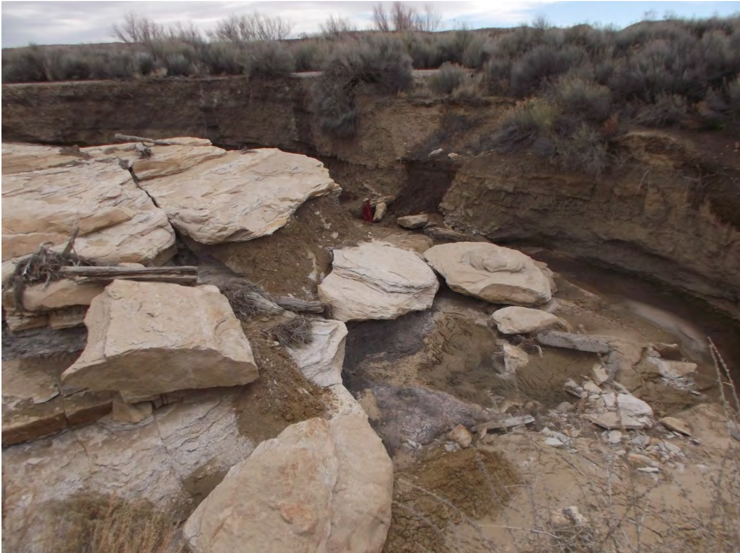
Photo I.7-3: Drainage Cut Approximately 150 Feet Downstream of the Rock Jetty
