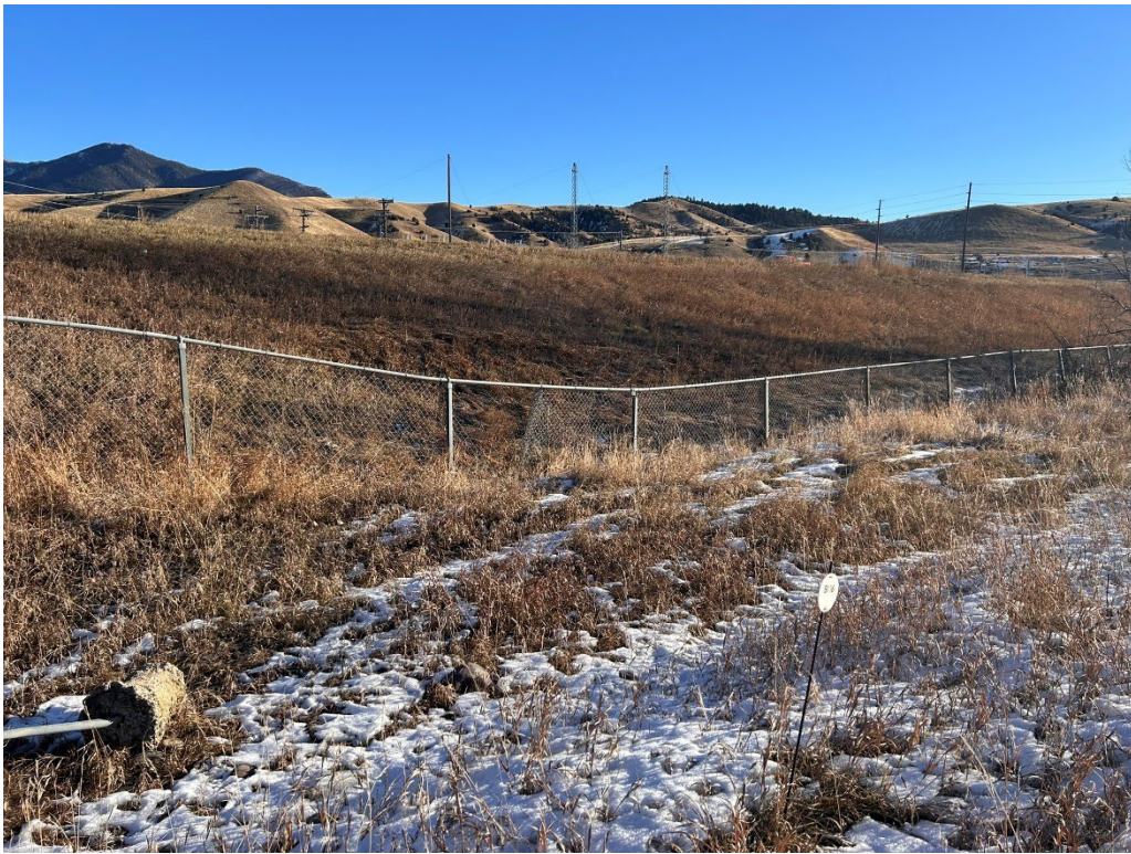
Hole in the fenceline
