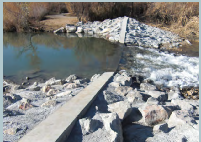
After: The replacement dam is a steel-reinforced boulder structure with low-flow channels that direct the water toward the center of the river to avoid riverbank erosion. The dam was also designed to allow for safe boat passage and portage for canoeists and kayakers.
