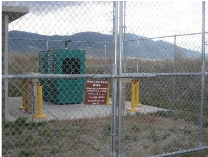
BPSOU: locked gate
