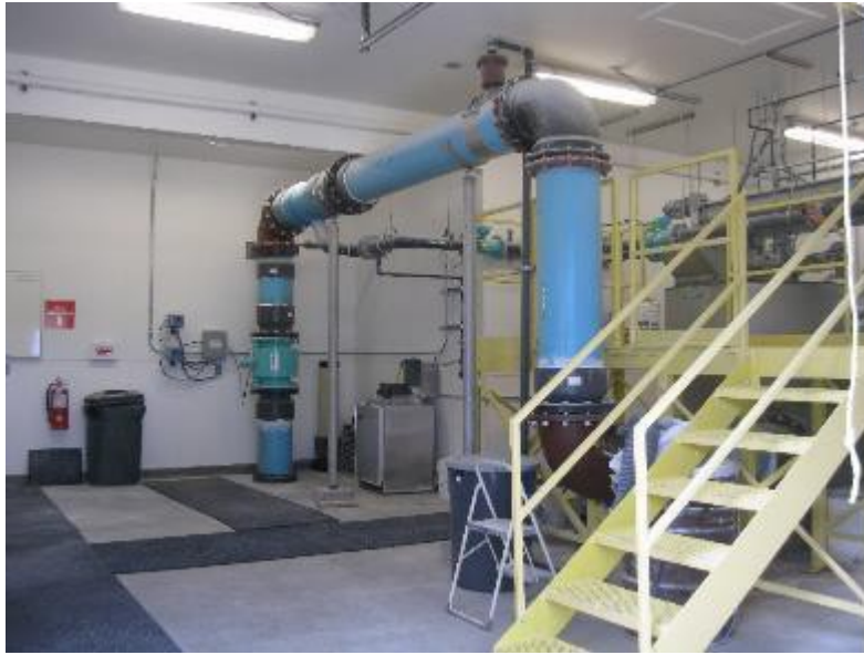
BPSOU: Butte Treatment Lagoons Chemical Addition Building – everything is new except stairs and platform
