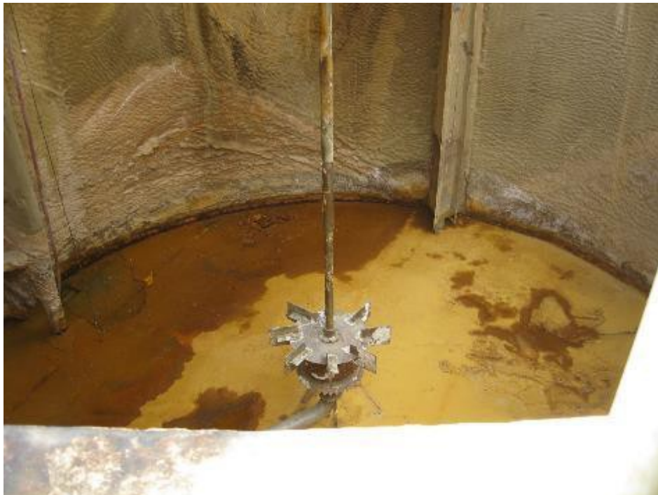
BMFOU: Crack in reactor
