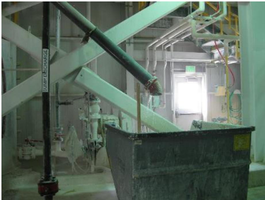
BMFOU: Lime receiving room
