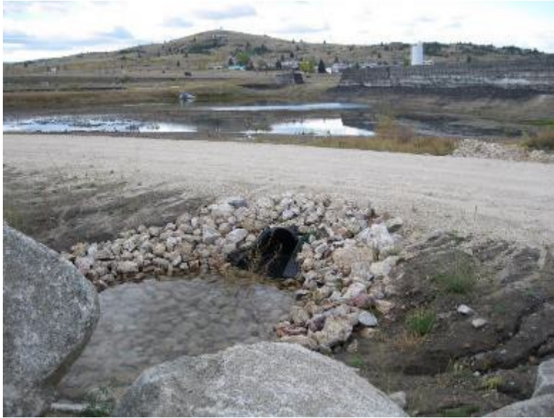
BPSOU: discharge out of drying bed
