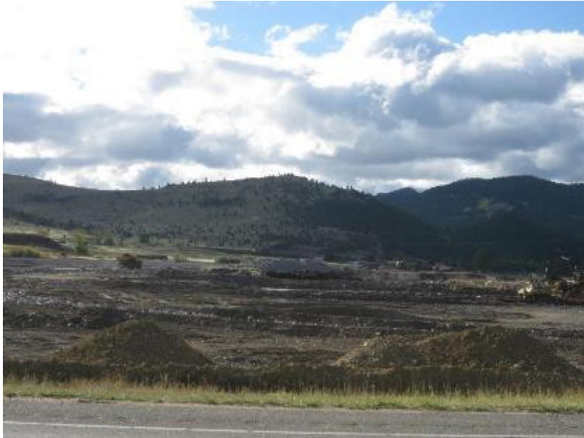
SSTOU: View of sediment pond construction (subarea 3) from bridge. Formerly full of tailings
