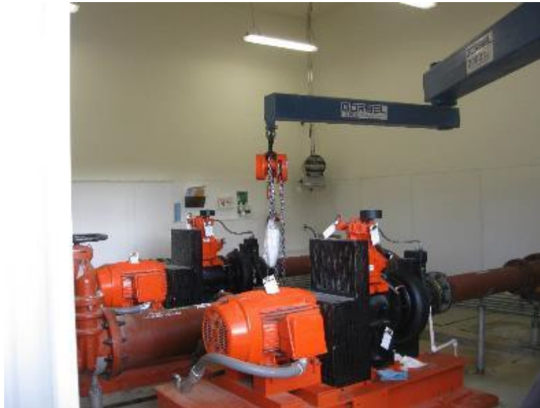
BPSOU: two pumps for D-4
