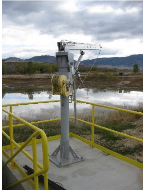
BPSOU: hoist at D4
