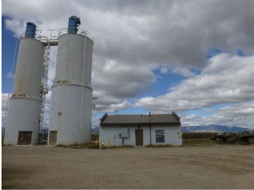
Warm Springs Ponds: Lime treatment silos
