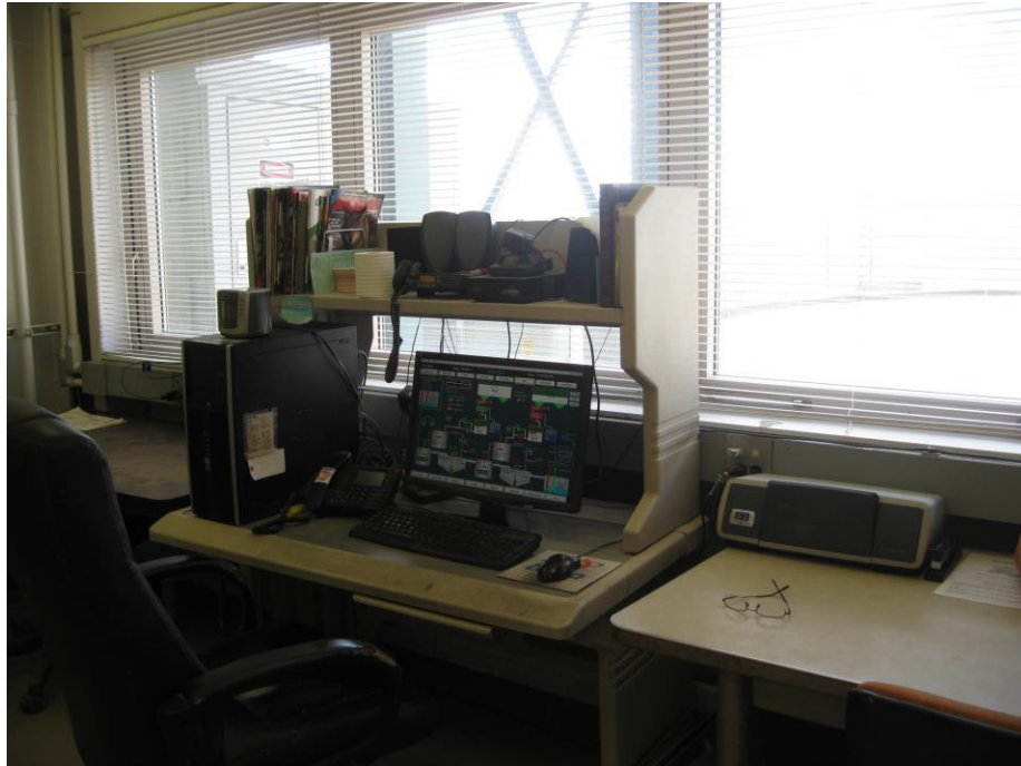
BMFOU: Treatment Plant Control Room
