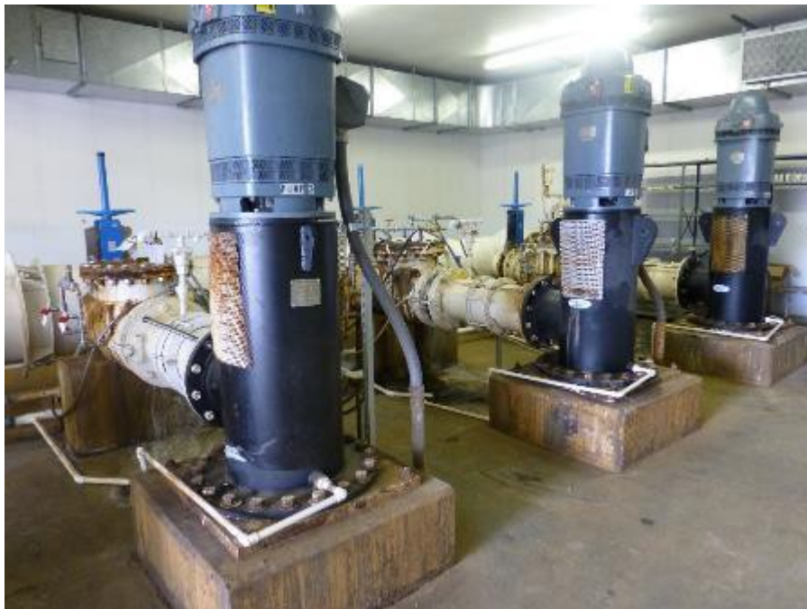
Warm Springs Ponds: Water level pumps
