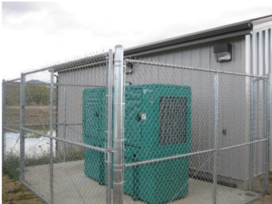
BPSOU: backup power generator next to D4
