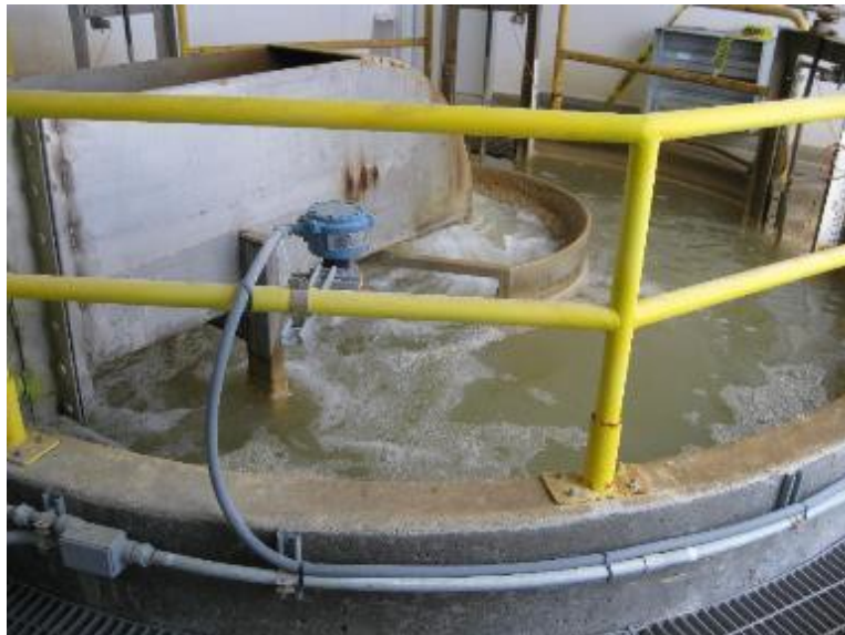
BPSOU: distribution tank
