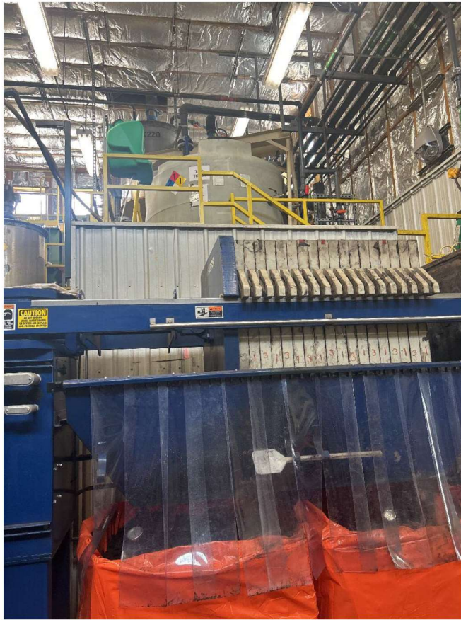
Interior of the WTP
