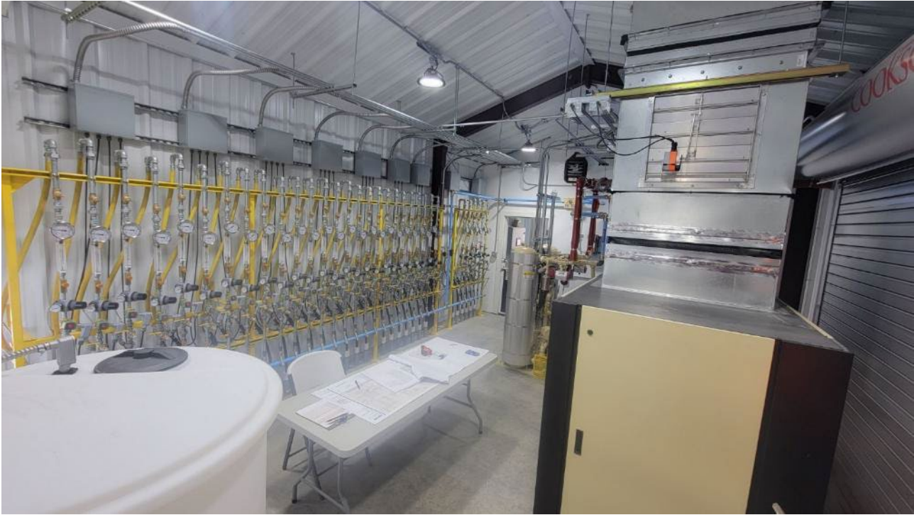
Photograph 22: Area 2 ISB compressed air system..
