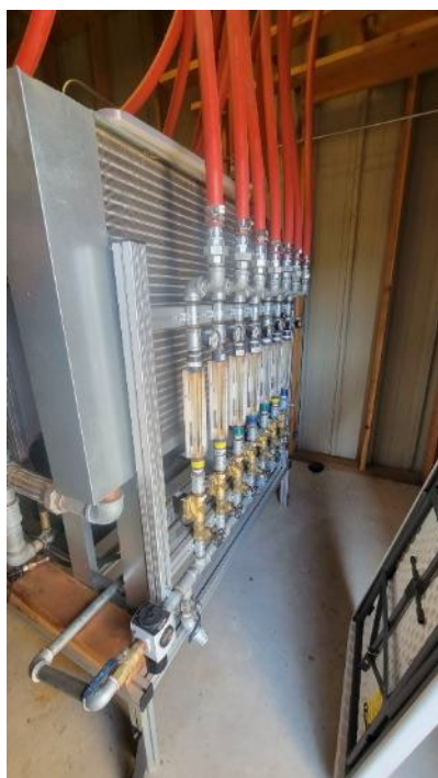
Photograph 19: Area 1 ISB – pilot scale manifold. To be used for the for Remedial Action system
