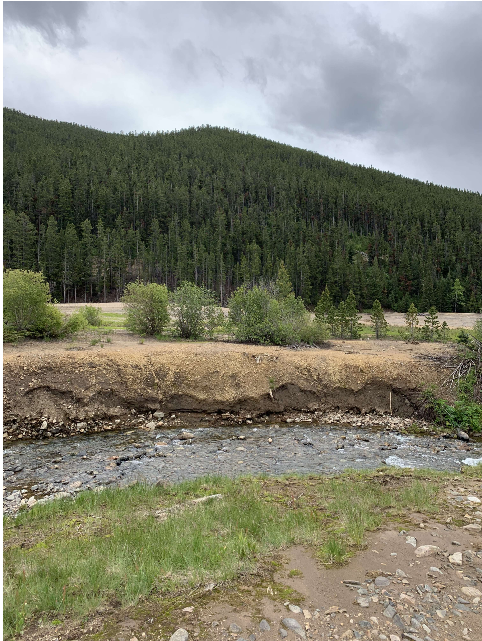
Figure 8: Photograph taken on June 21, 2023, showing the undercutting of the Lower Tailings Impoundment
