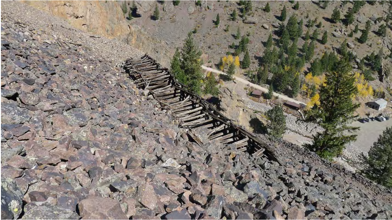
Photo No. 45: Detail of unfilled cells of lower cribbing wall at Lower Bachelor waste rock dump. Commodore surface plant below at creek side. Camera facing northeast.
