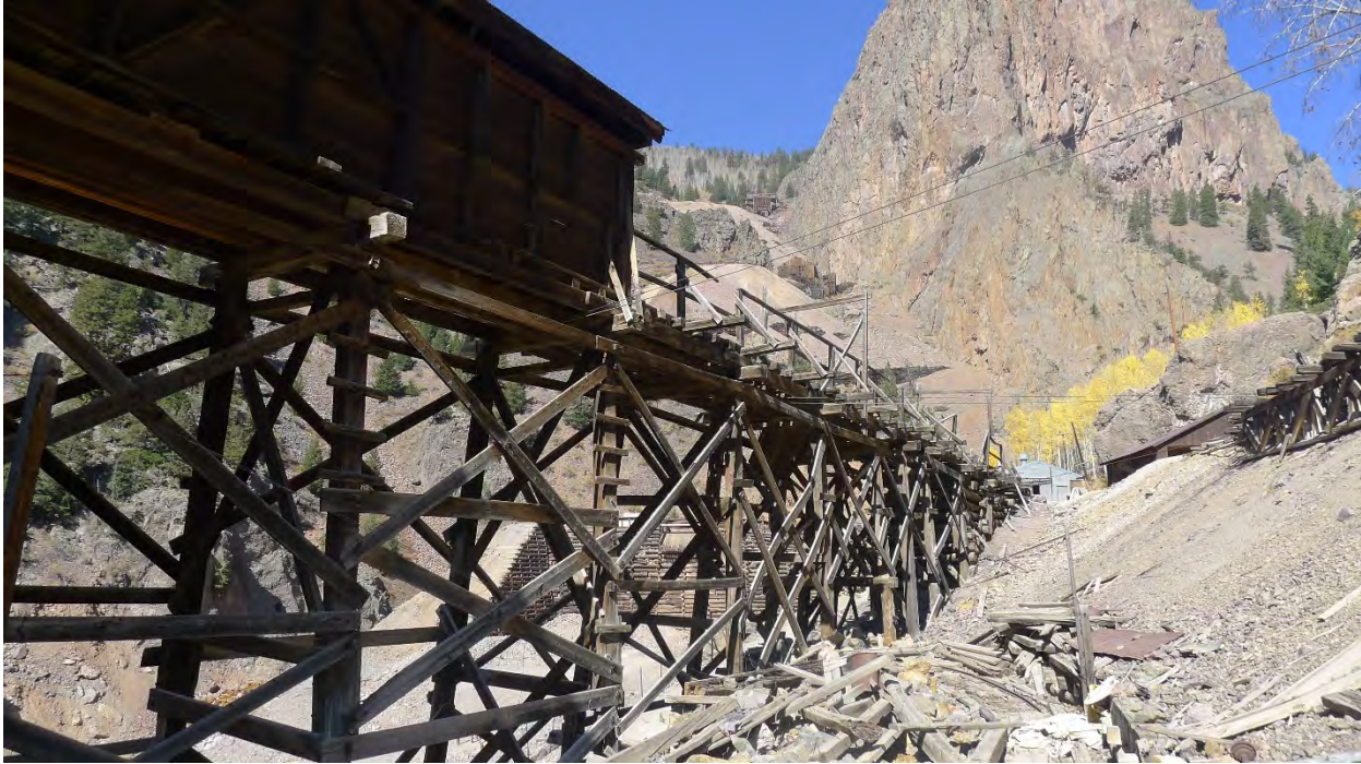
Photo No. 21: East side of trestle of Commodore ore sorting house; snow shed at left. Camera facing west.
