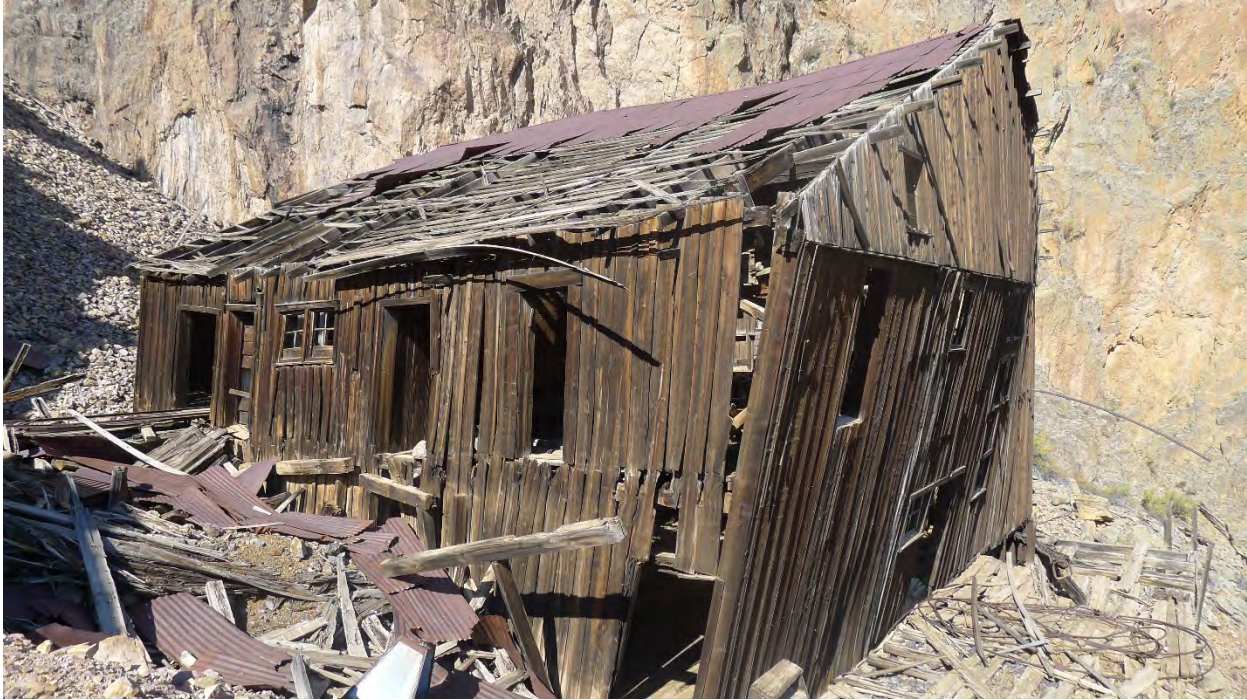
Photo No. 57: East and south sides of Lower Bachelor ore sorting house and aerial tramway terminal (Resource 29). Camera facing north.
