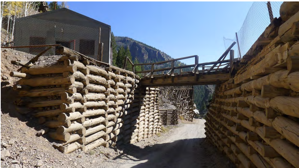
Photo No. 28: View of rail bridge (Resource 9) from road below, with cribbing walls of southeast and south waste rock dumps at either side. Camera facing south.
