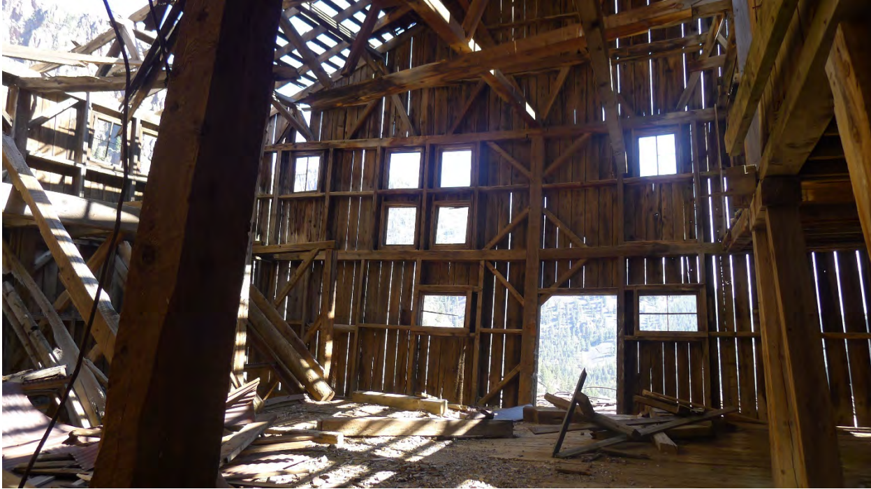
Photo No. 63: Interior of Lower Bachelor ore sorting house. Camera facing southeast.
