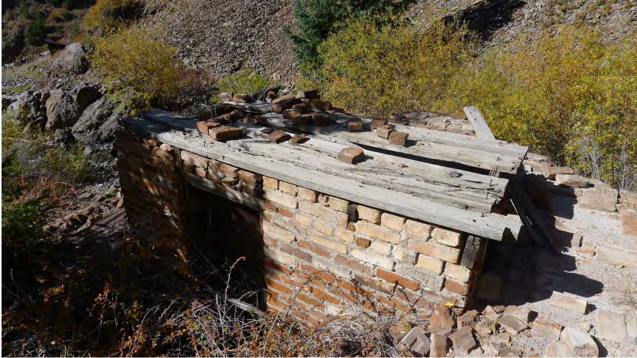
Photo No. 39: Detail of boiler setting remnant at powerhouse ruins. Camera facing west.
