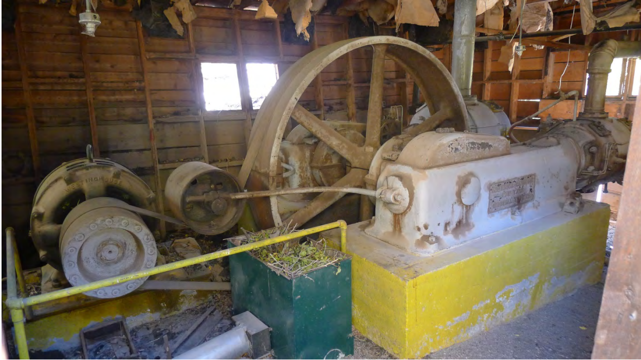
Photo No. 37: Interior of compressor house (Resource 17), showing the belt-driven duplex Ingersoll-Rand Imperial Type 10 compressor. Camera facing east.
