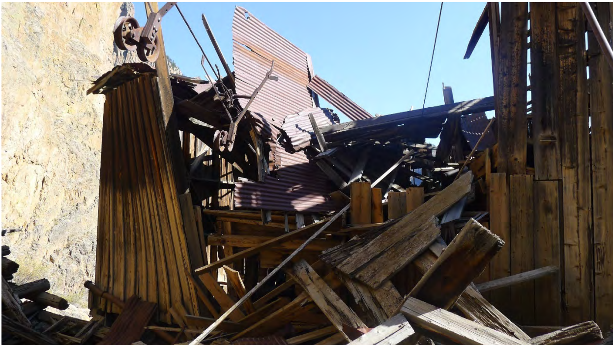
Photo No. 62: Detail of west side of north extension of Lower Bachelor ore sorting house. Note ore bucket hangers still suspended on aerial tram cables. Camera facing southeast.
