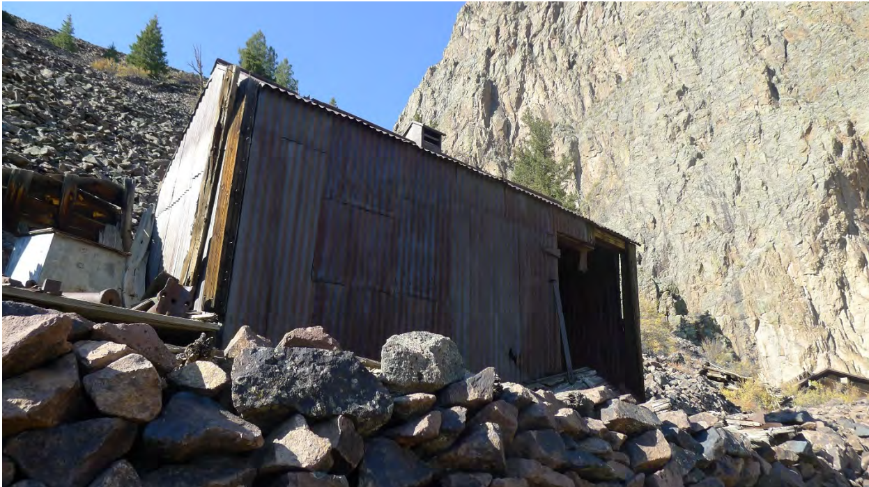
Photo No. 48: South and east sides of dynamite thaw house (Resource 24). Camera facing northwest.
