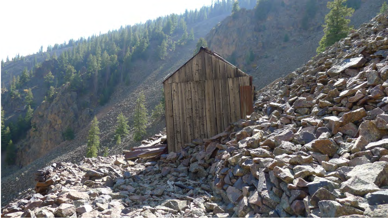
Photo No. 49: North side of dynamite thaw house (Resource 24). Camera facing southwest.
