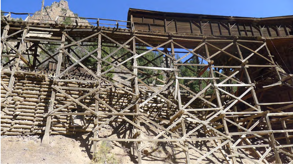
Photo No. 19: West side of trestle of Commodore ore sorting house; snow shed at top. Camera facing northeast.
