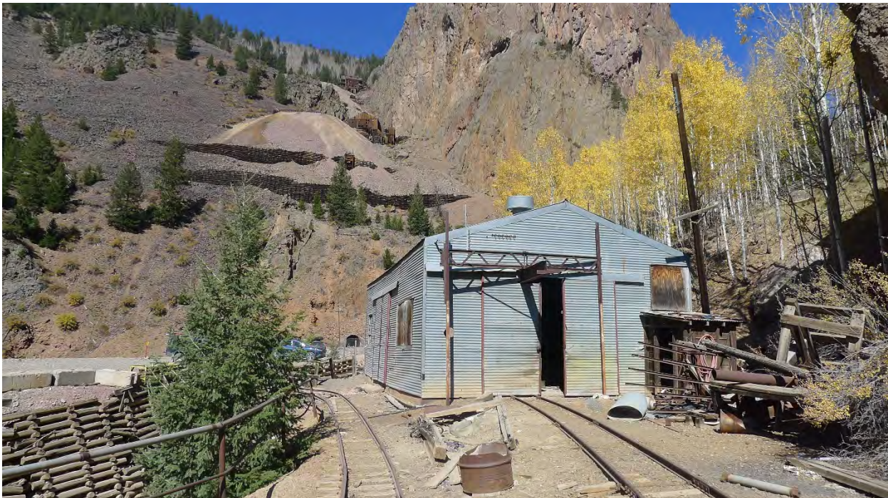
Photo No. 26: South side of shop building (Resource 8). Bachelor Mountain in distance. Camera facing northwest.
