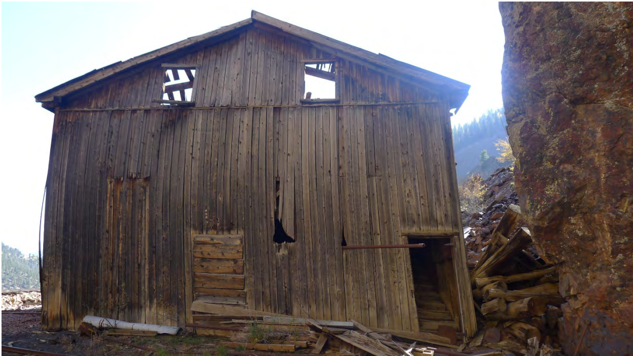
Photo No. 56: North side of shop (Resource 28), with wall of bedrock outcrop at right. Camera facing south.
