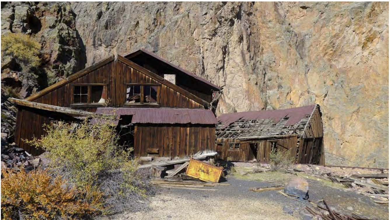
Lower Bachelor Shop (Resource #28) at left, and Lower Bachelor Ore Sorting House and Aerial Tramway Terminal (Resource #29) beyond at right. Camera facing north.
