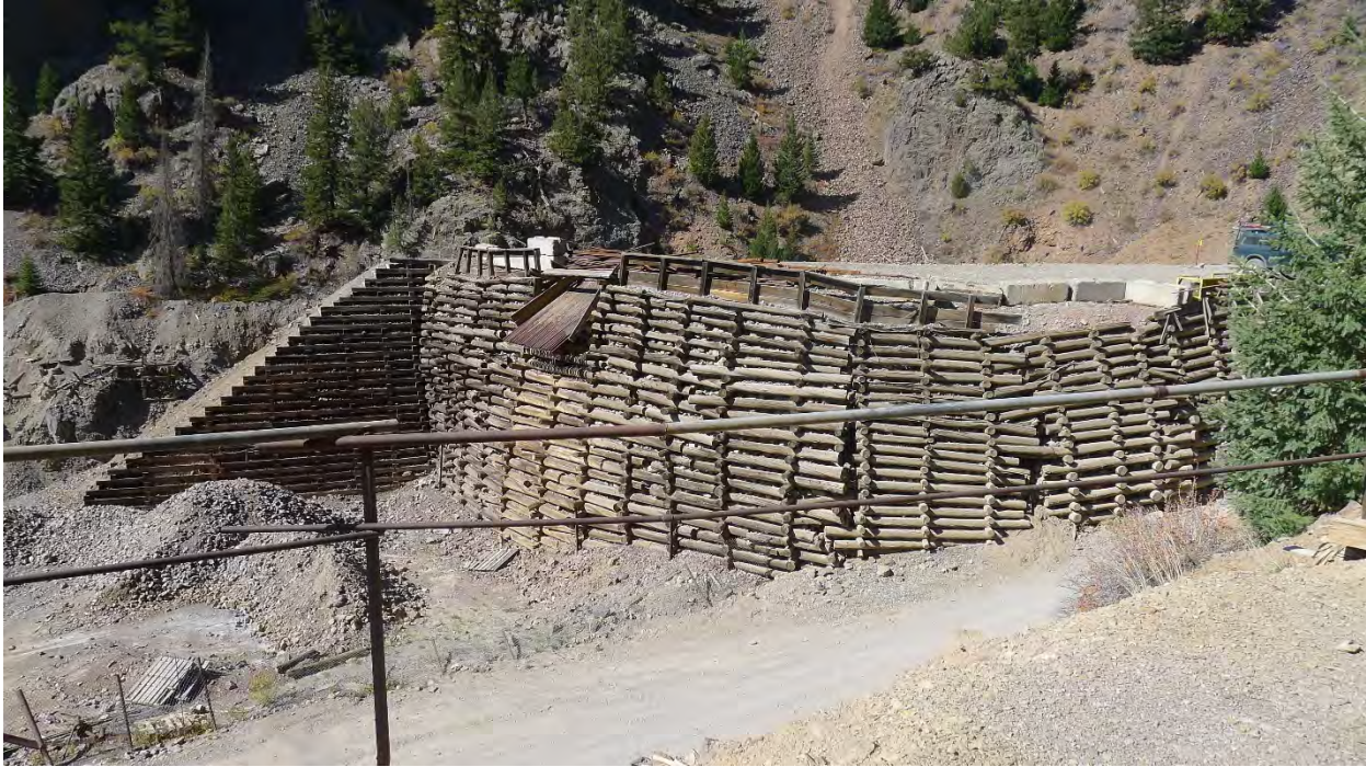
Photo No. 29: View of top of remaining section south waste rock dump and cribbing wall with ore chute (Site Feature 2). Camera facing west.
