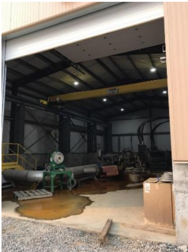
Capture system pump house
