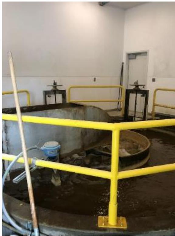
Lime treatment at Butte Treatment Lagoons
