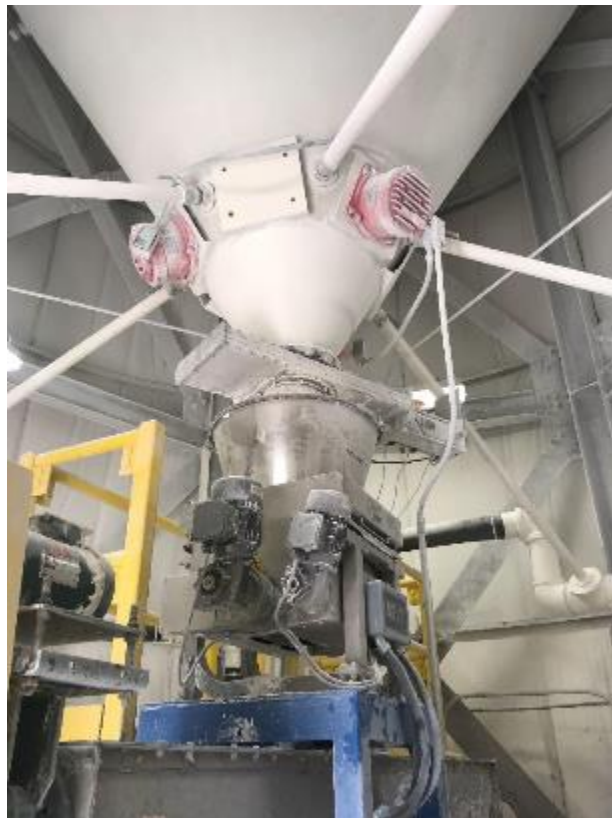
Lime treatment silo
