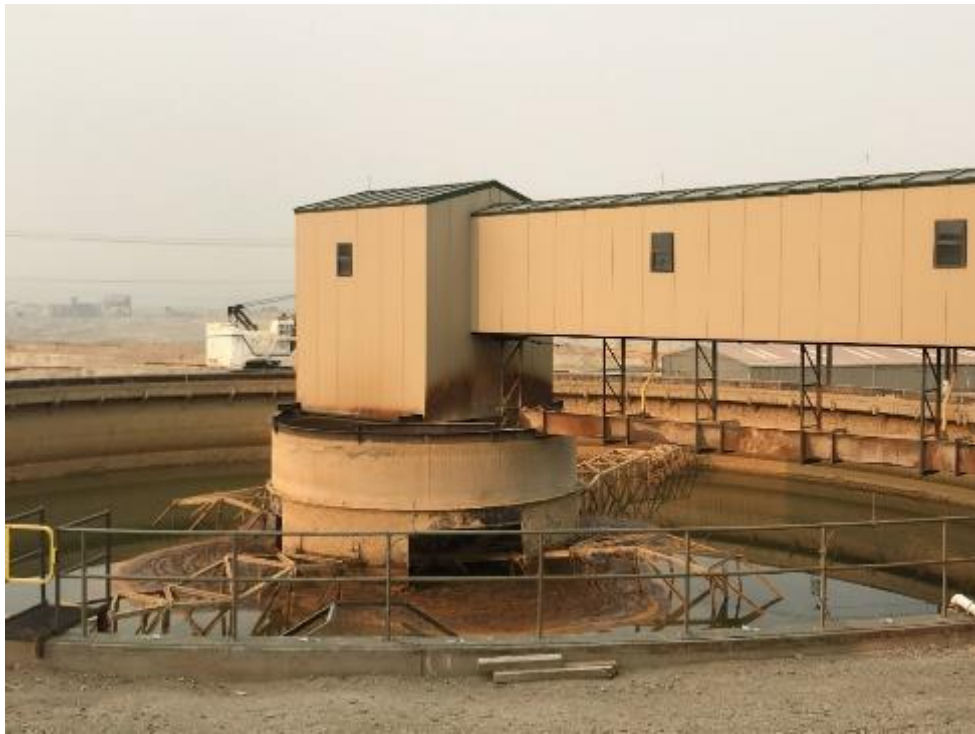
Sludge accumulation at HsBWTP
