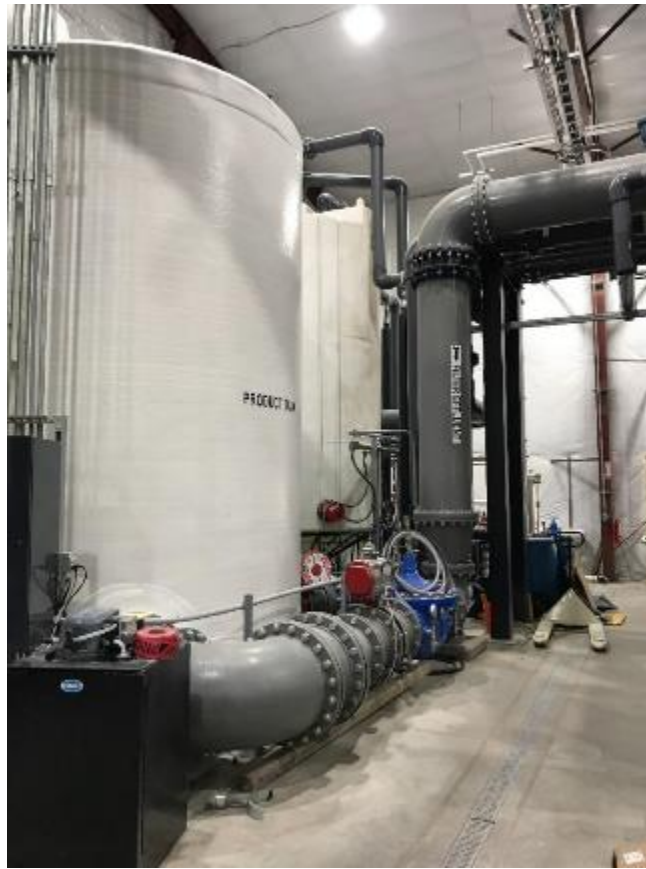
Product tank and effluent filter in Polishing Plant
