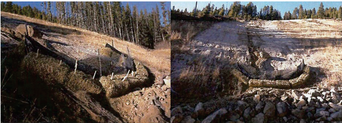
Figure 4: Reinforced silt fencing, straw bales, and wattles temporarily used to prevent sediment from reaching No Name Creek (Photos taken in 2016).
