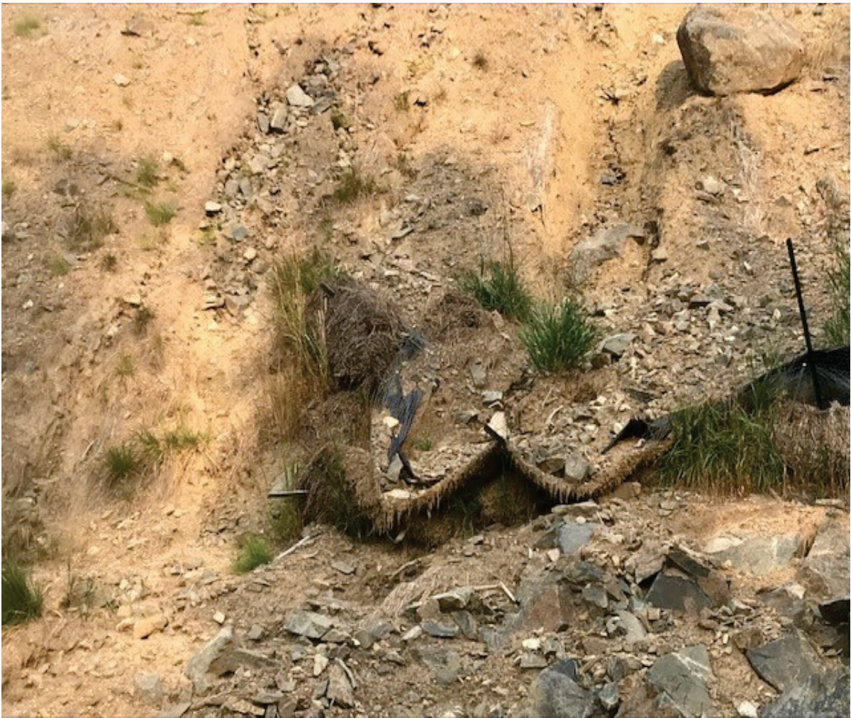
Figure 3: Displaced wattles and initiation of gully erosion at the base of the impoundment erosion control.
