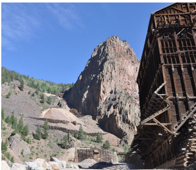
Commodore Ore House on right with cribbing and Commodore 3 and 4 visible up the slope to the left.
