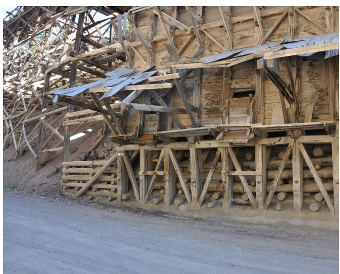
Deteriorating condition of the Ore House roof.
