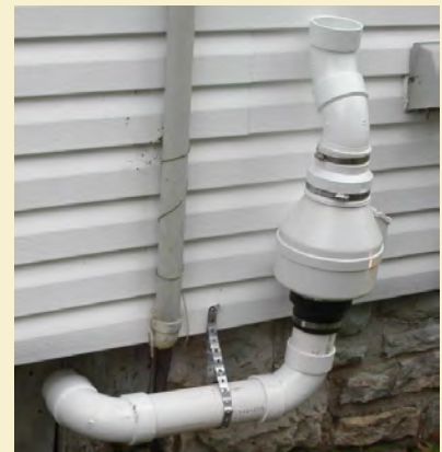
One of the residential ventilation systems installed near the site.
