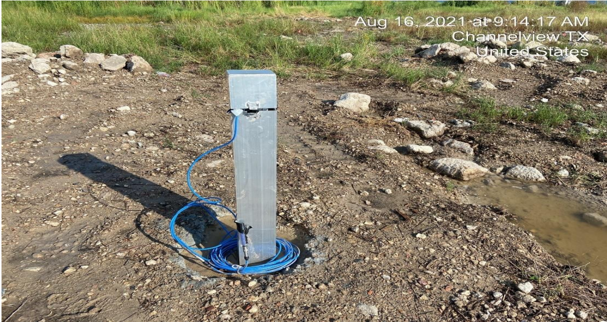
Photo 15 Transducer installed at location SJMW-016.
