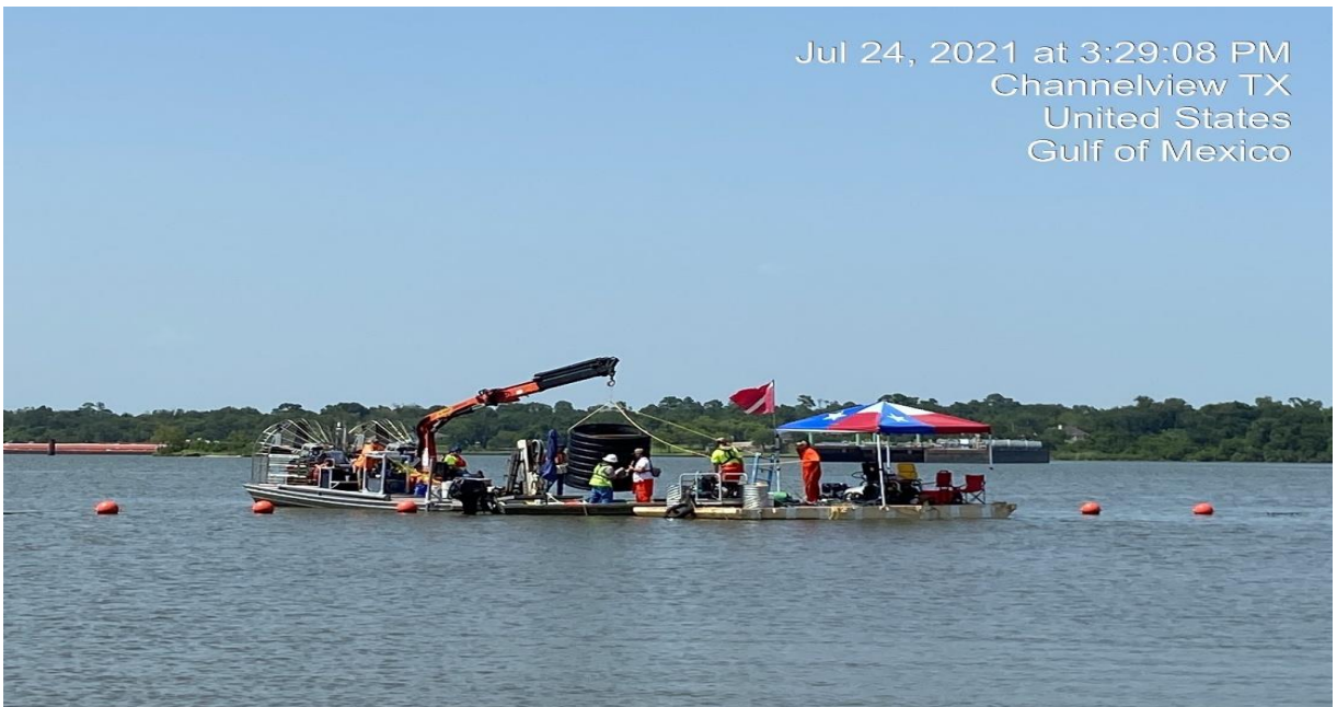
Photo 8 Airboat and dive crews installing a large culvert to assist in clearing rock at boring location SJSB100.
