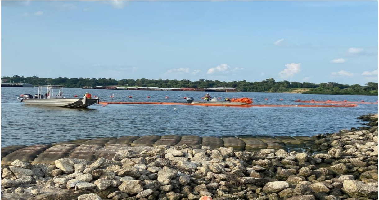
Photo 17 View from land, subcontractor crew installing turbidity curtain near boring location SJSB103.
