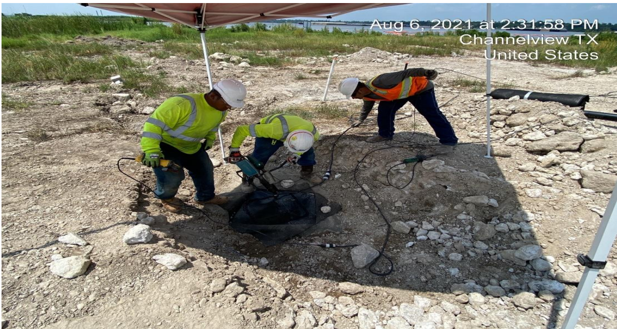
Photo 12 Subcontractor welding a patch on the geomembrane liner following drilling activities at boring location SJSB078.
