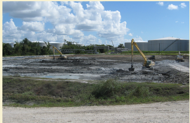
Solidification of sediments in the settling basin in October 2014.
