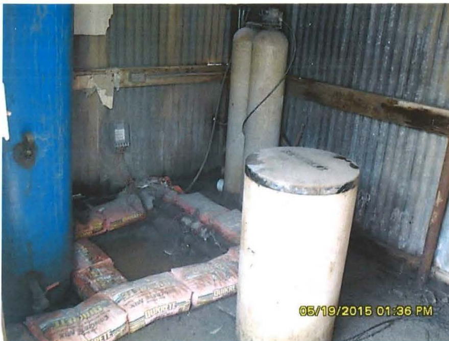
Figure 3 - Onsite water well with sandbags as a temporary emergency measure to prevent further migration of hazardous substances entering the wellbore.
