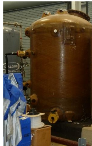
Figure 4. Liquid creosote collection tank.
