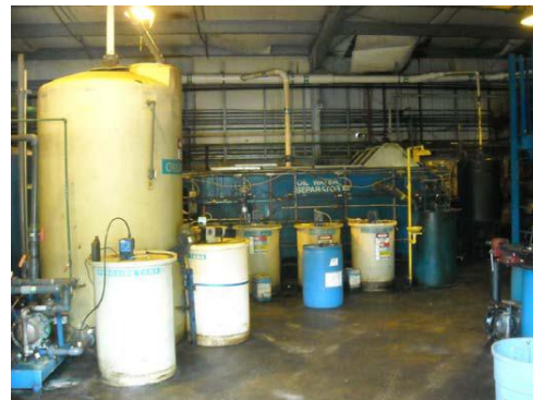
Figure 7. Oil/water separator inside the site's treatment system facility.
