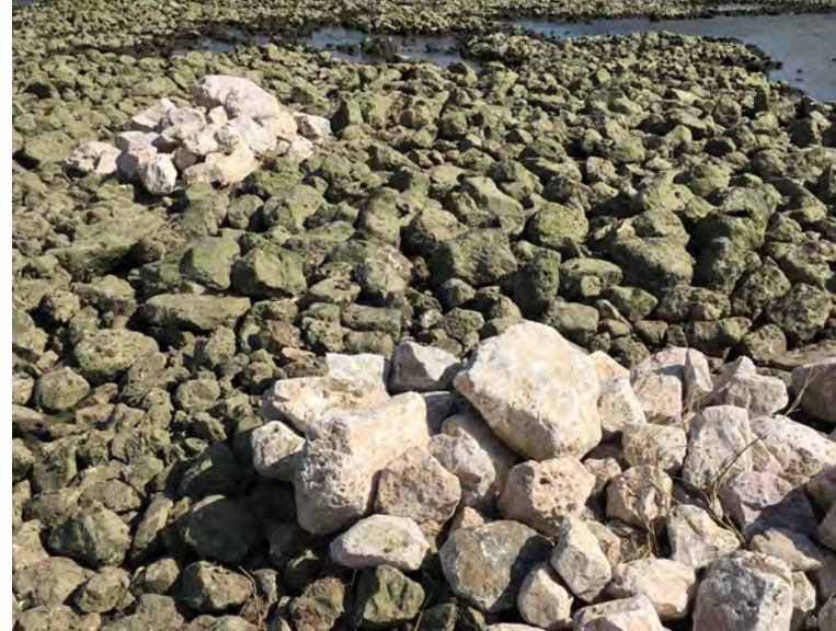
Photograph 6: Example of previously visible geotextile areas in the eastern cell, after the completion of maintenance, on February 26, 2020
