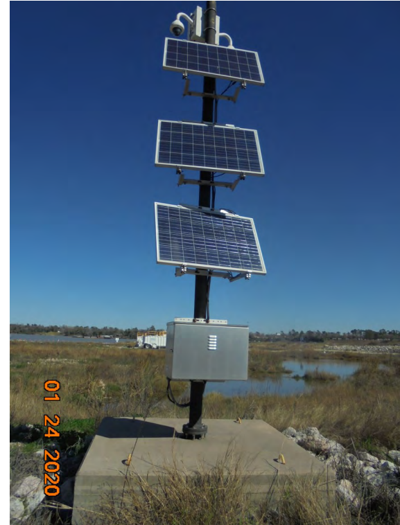
Photograph 22: View of security camera apparatus on southern berm (western cell) (view northeast)
