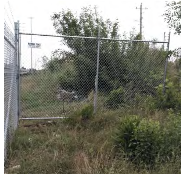
Photograph 12: View of installed fence extension south of I-10 on west bank, on April 8, 2020 (view east)
