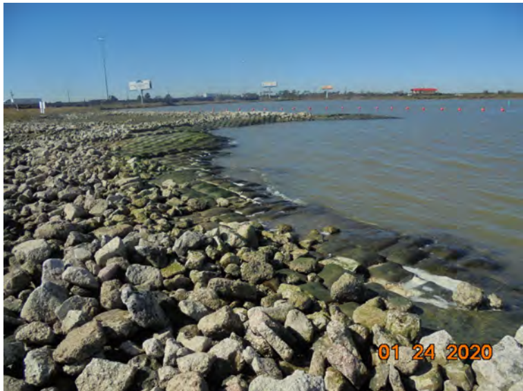
Photograph 7: View of the western cell, articulated concrete block mat (ACBM) northwest slope enhancement, and perimeter buoy system (view southwest)
