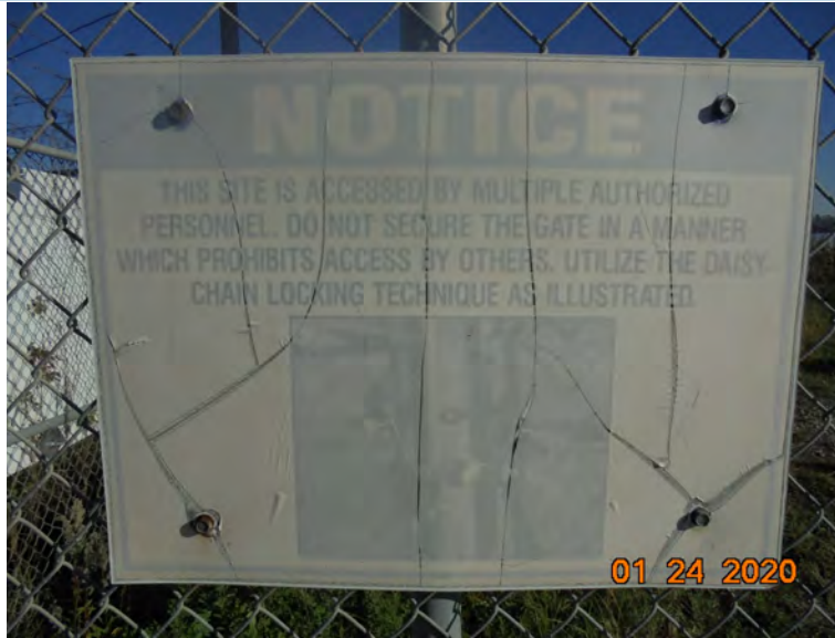
Photograph 9: View of daisy chain sign to be replaced. Note this is an informational sign, not an EPA-required sign.
