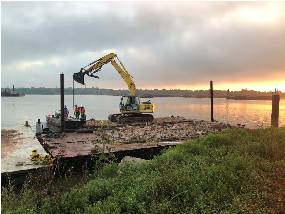
Photograph 1 – Barges loaded with Dynamic Excavator and rock at San Jacinto River Fleet property.
