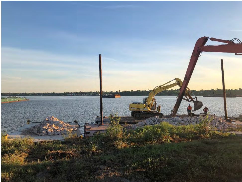
Photograph 1 – Rock and equipment being loaded onto barges at San Jacinto River Fleet property.
