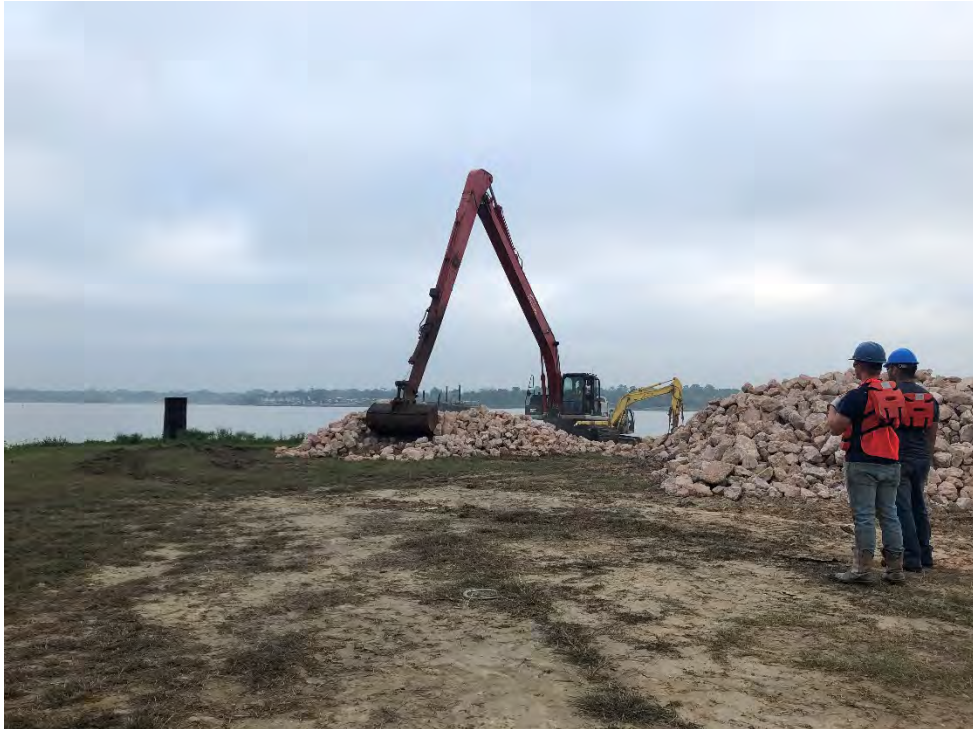
Photograph 1 – Rock being loaded with Long Front Excavator at San Jacinto River Fleet property.
