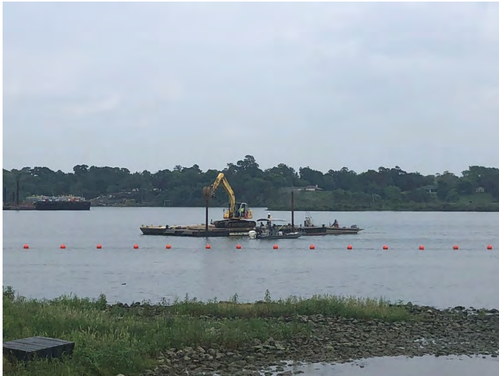
Photograph 1 – Rock placement corrections being conducted at Placement Areas 2 and 3 with assistance from surveyors.
