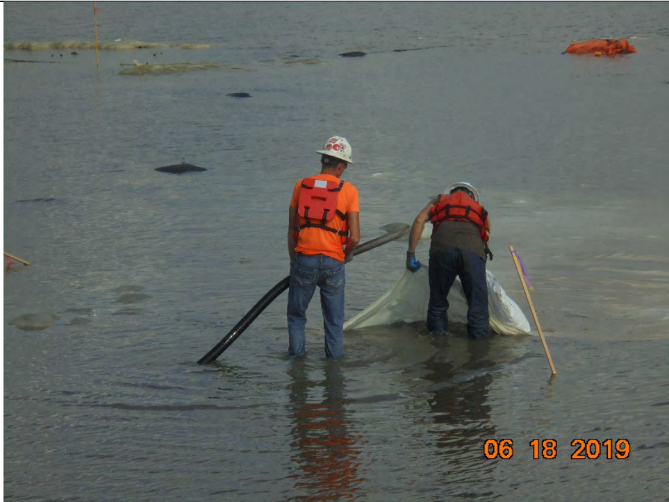
Photo 5 – CCI preparing to insert the grout hose into an ACBM form during grouting operations
