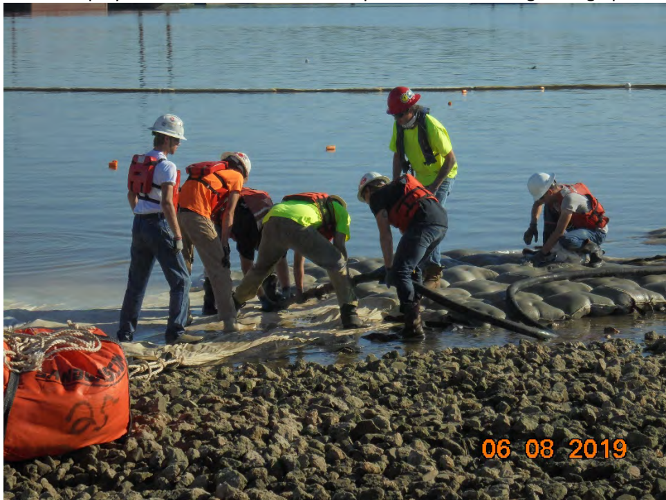
Photo 3 – Insertion of the grout hose into an ACBM form during grout pumping operations
