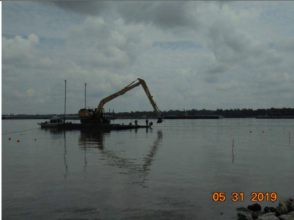
Photo 4 – Barge-mounted excavator pulling a rope attached to its bucket to unroll underwater roll of ACBM form and geotextile fabric
