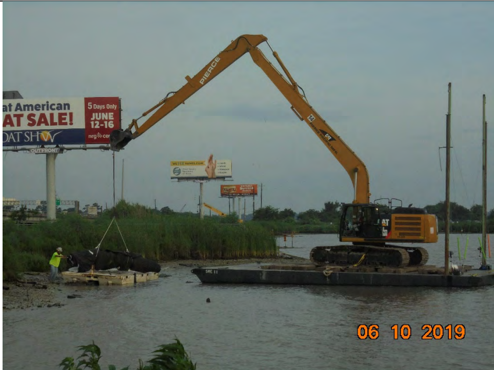
Photo 5 – Barge loading of ACBM form for transport and deployment at the installation site
