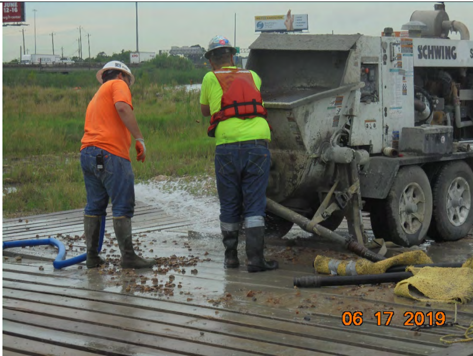
Photo 5 – Removal of observed coarse aggregate from rejected delivery trucks from the screen of the grout pump
