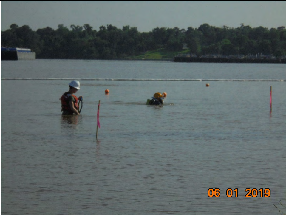
Photo 2 – Diver entering water to perform ACBM panel zippering, as CCI provides assistance with air hose
