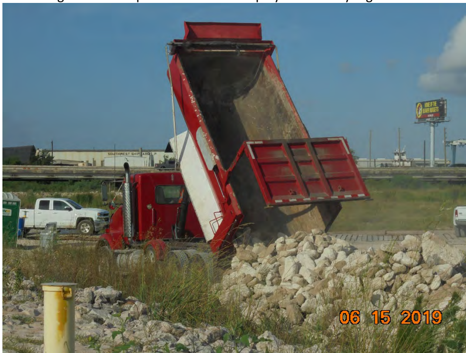
Photo 2 – Delivery of riprap for armoring the southern edge of the installed ACBM
