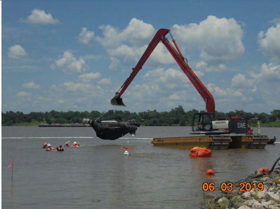
Photo 5 – Roll of ACBM and geotextile fabric being placed in the water for unrolling and positioning
