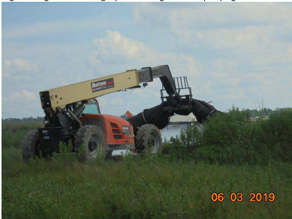
Photo 4 – Roll of ACBM and geotextile fabric being loaded onto barge for transport to the installation site
