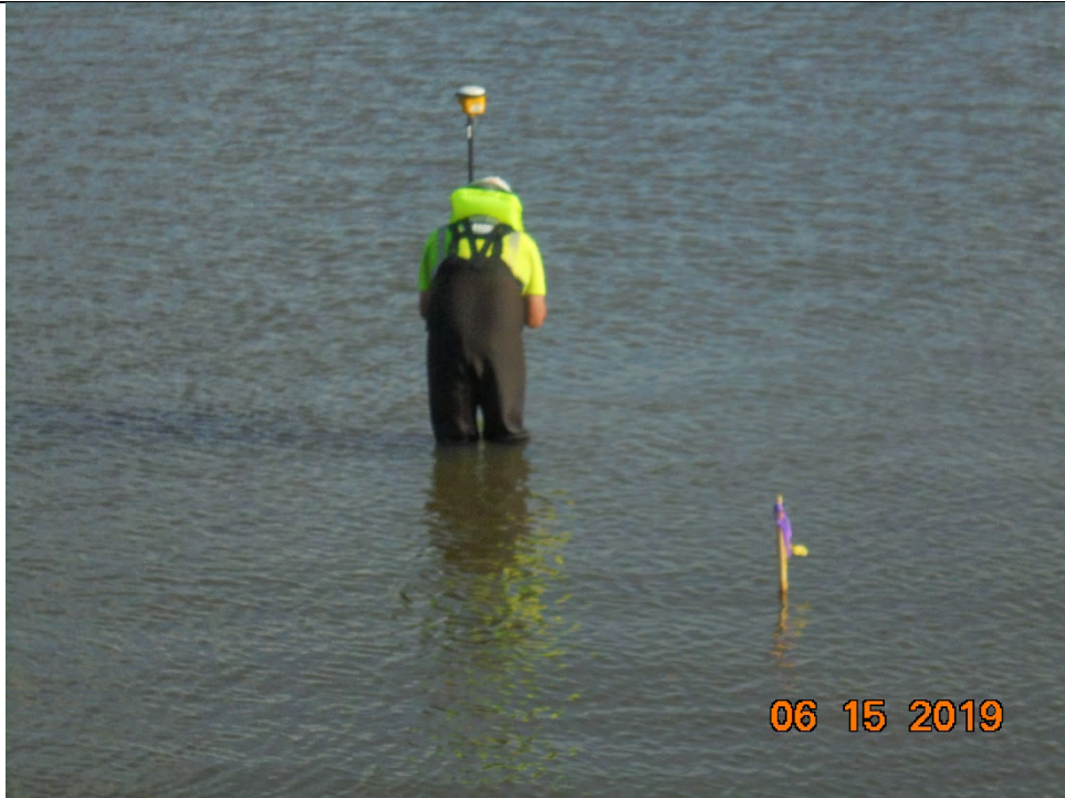
Photo 3 – Stakeout of limits for riprap placement along southern edge of installed ACBM
