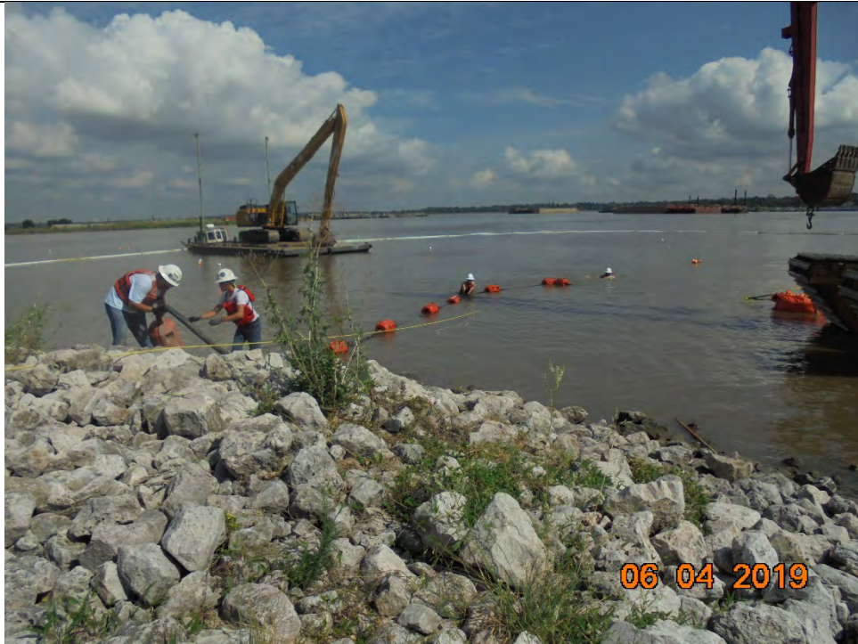
Photo 3 – Setup of grout hose at the ACBM installation site in preparation for grout pumping
