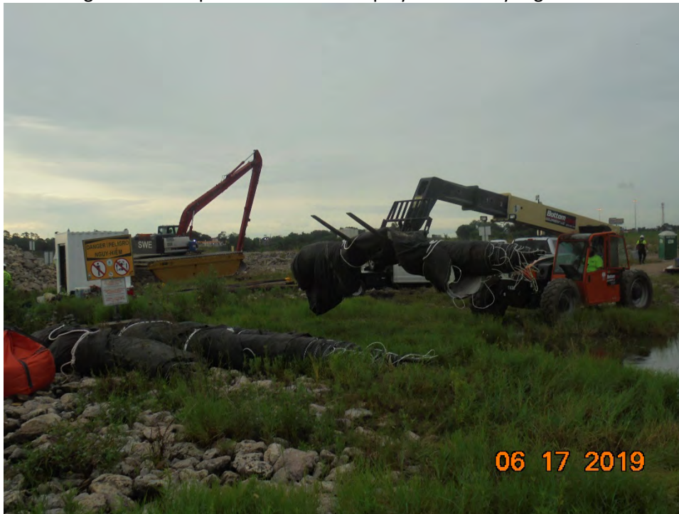
Photo 2 – Staging of ACBM forms near the shoreline of the installation site for deployment
