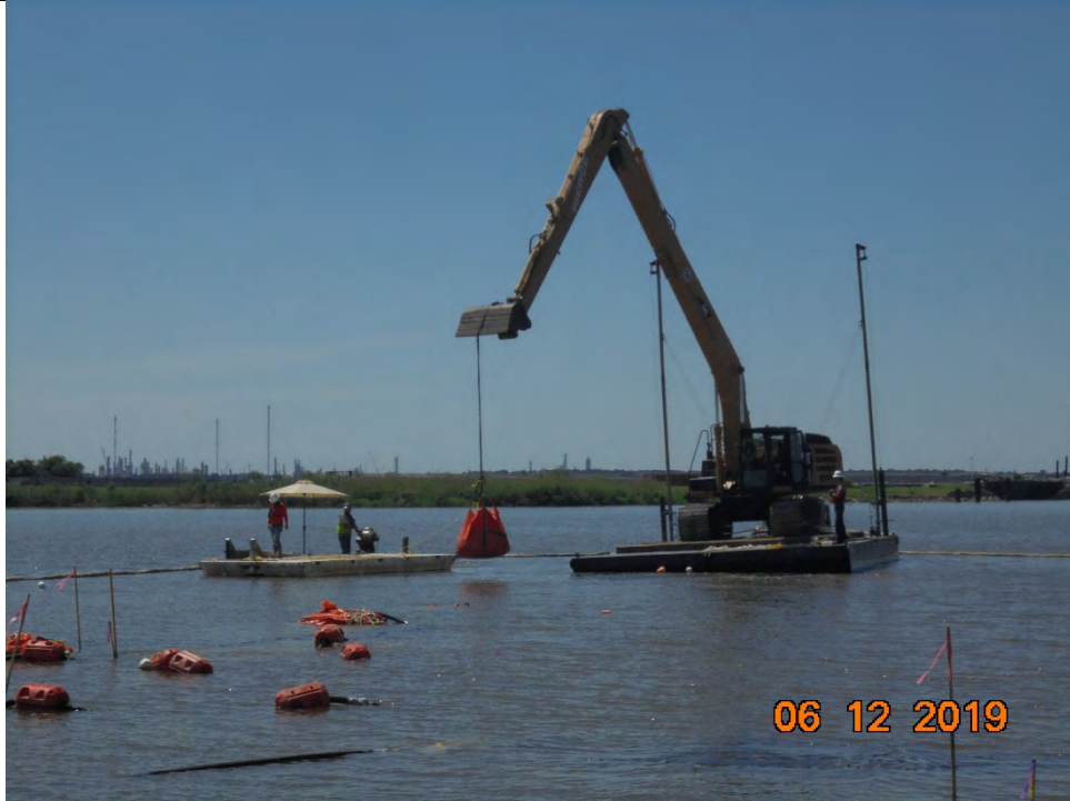
Photo 5 – Sandbags being lowered into the water as anchoring points during ACBM deployment operations
