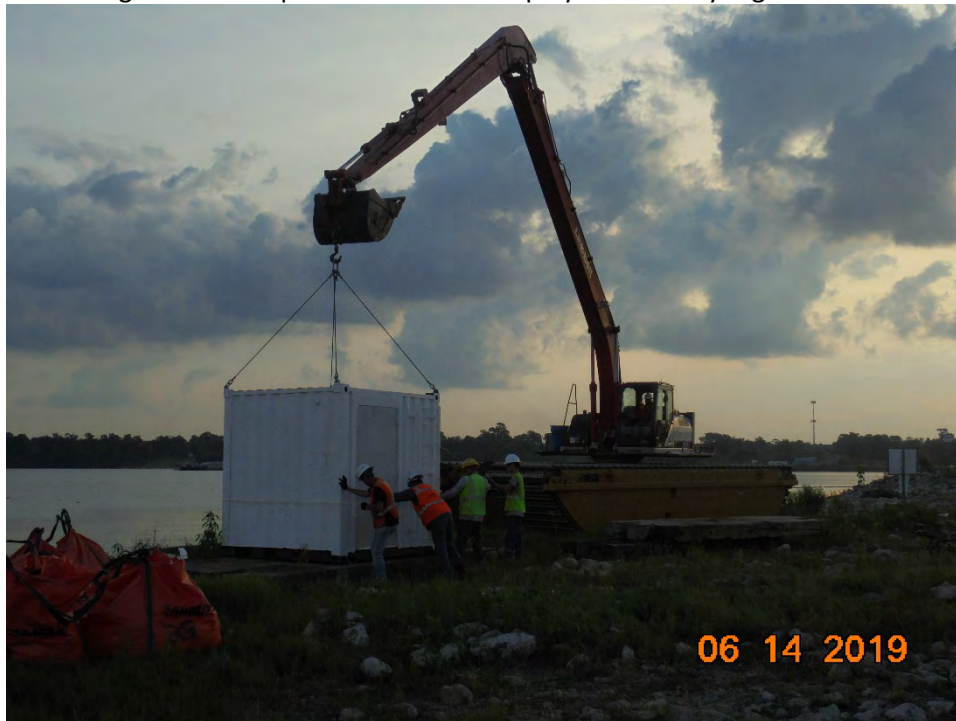
Photo 2 – Relocation of dive shack near the installation site of 400-series ACBM panels
