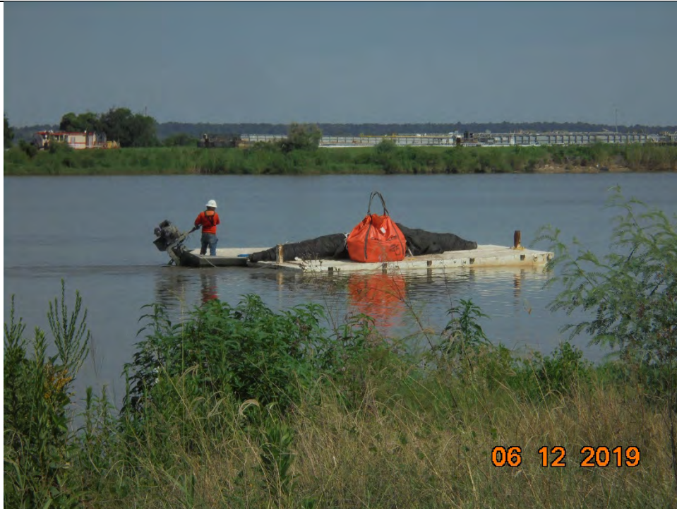
Photo 3 – ACBM form 305 and anchoring sandbags being transported by barge to the installation site for deployment
