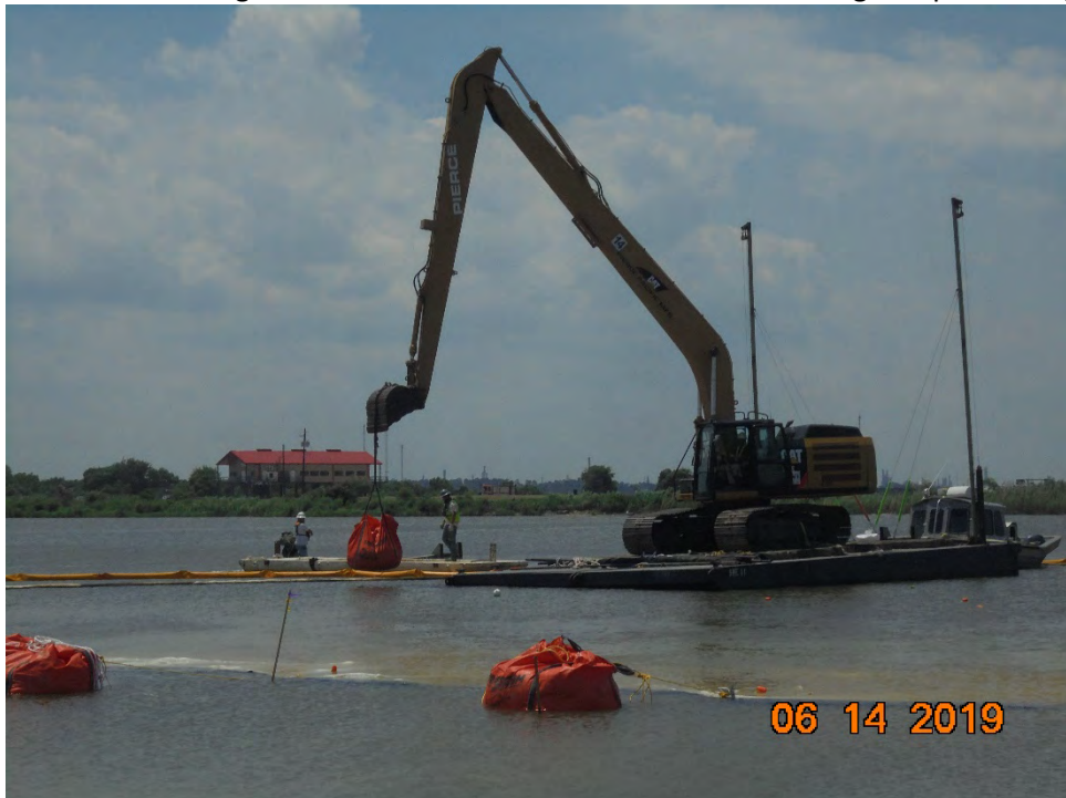
Photo 6 – Barge-mounted excavator placing anchoring sandbags into the water for deployed ACBM forms
