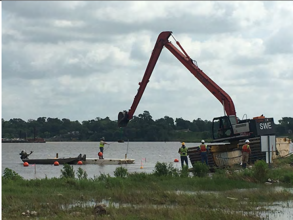
Photo 4 – Temporary removal of perimeter buoy segment for construction access to ACBM installation site
