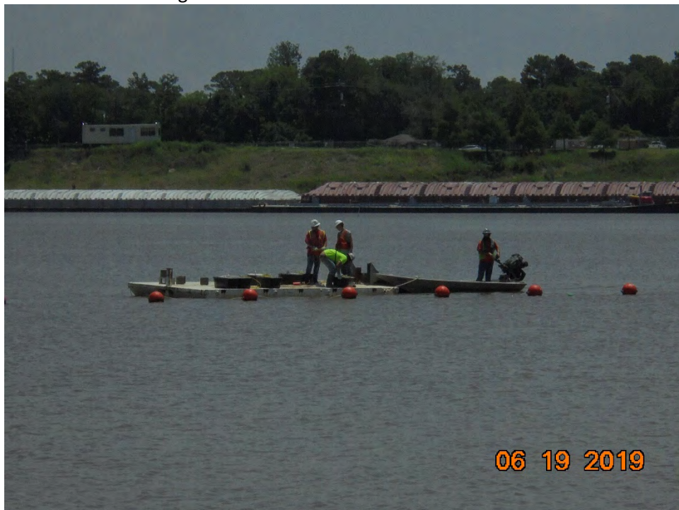
Photo 5 – Installation of additional anchors along the perimeter buoy system on the east side of the Central Berm
