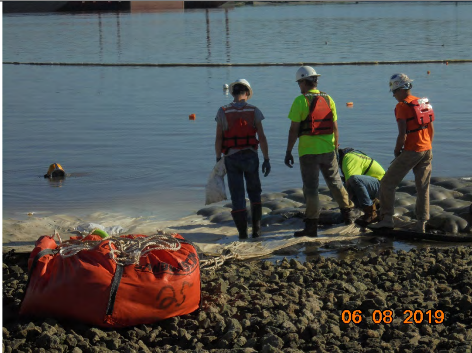
Photo 4 – Grouting of ACBM form from the shoreline, as dive crew monitors filling of underwater portion of the form
