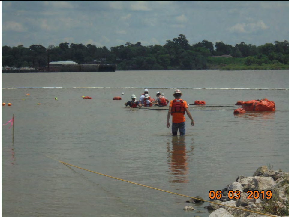
Photo 3 – Segment of grout hose being replaced during a break in pumping after a leak was observed
