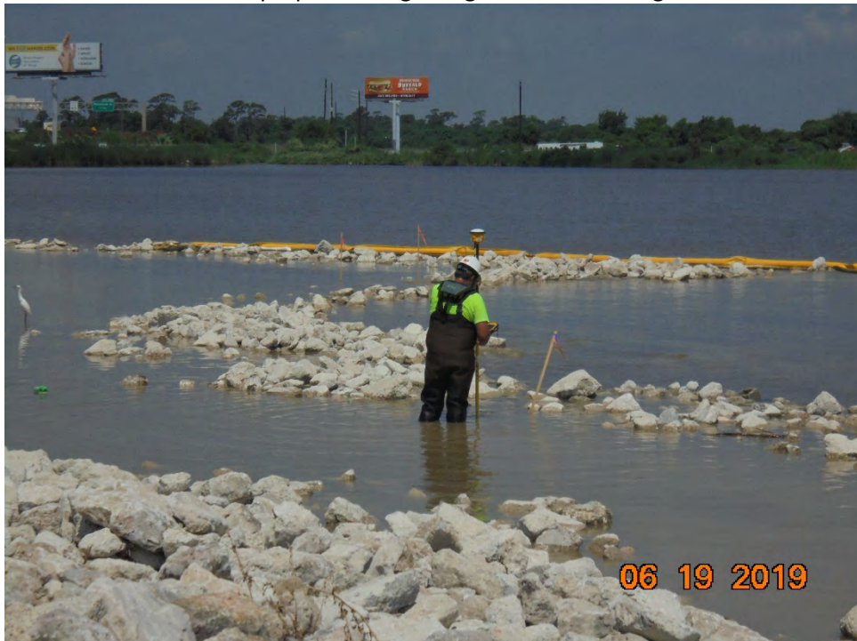
Photo 3 – Surveying of riprap armor extents along the southern edge of installed ACBM
