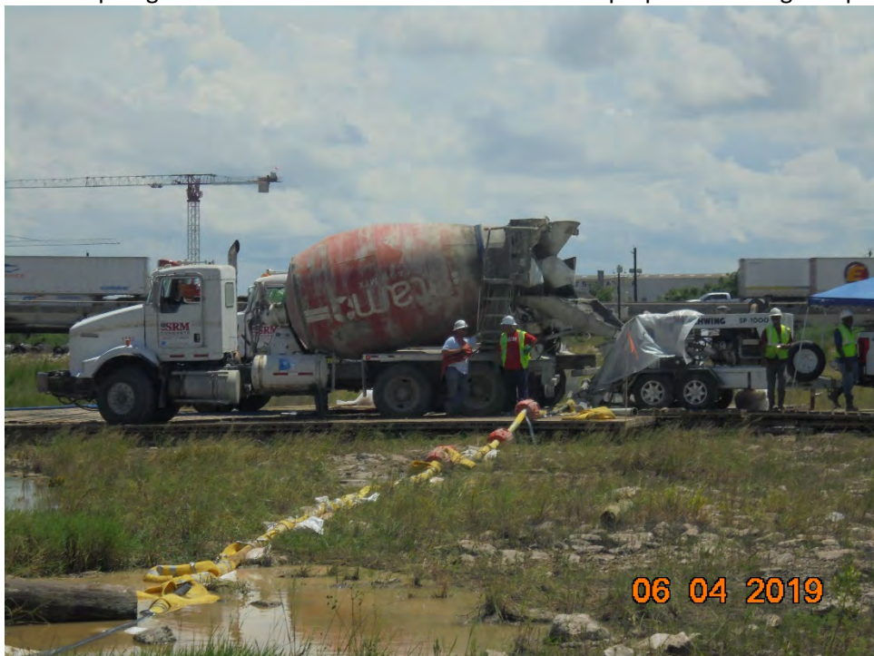
Photo 4 – Concrete being offloaded from delivery trucks into grout pump during ACBM panel grouting
