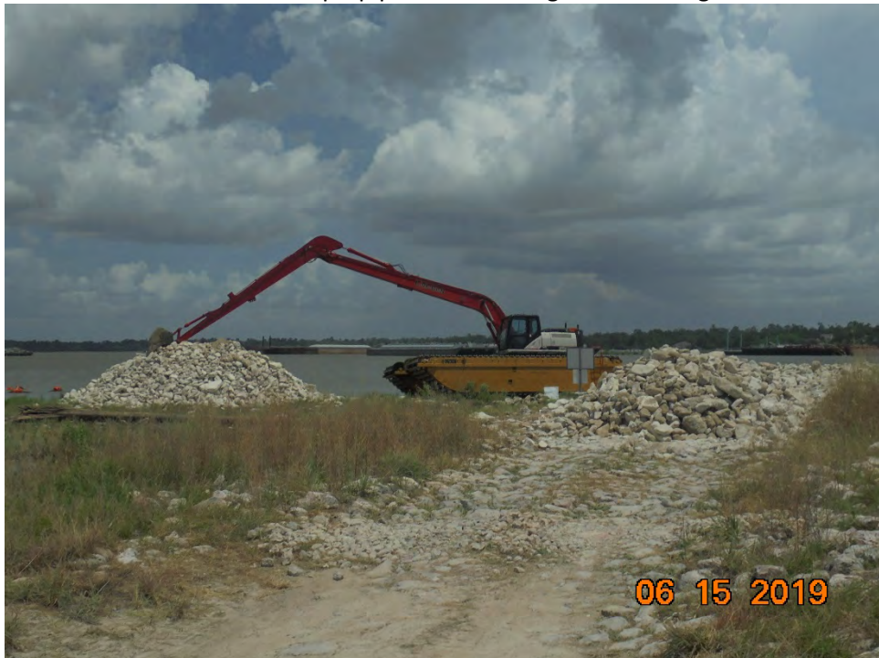
Photo 4 – Stockpiles of riprap staged near the shoreline of the ACBM installation site
