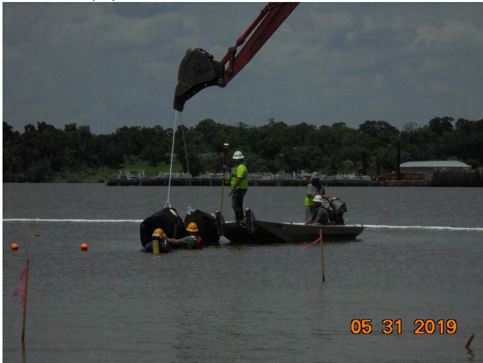
Photo 3– Marsh buggy placing roll of ACBM form and geotextile fabric into the water for unrolling and positioning
