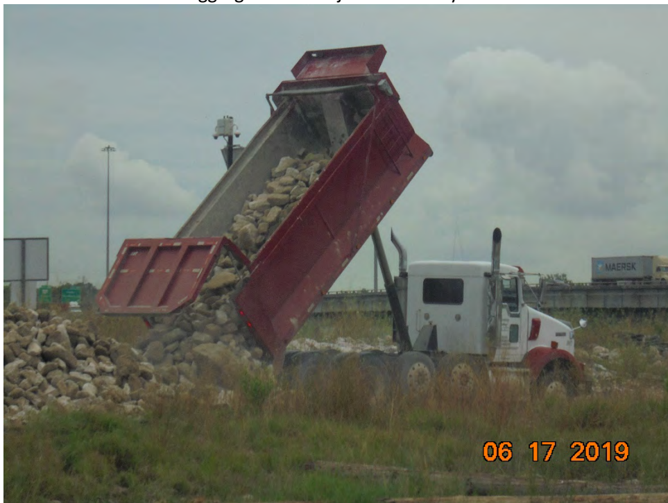
Photo 6 – Delivery of riprap for armoring the southern edge of the installed ACBM
