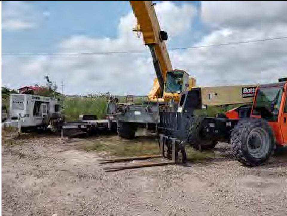
Photo 4 – Small fork lift, and 4phase grout pump. (Crane belongs to bridge contractor).
