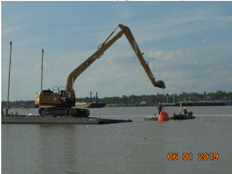
Photo 5 – SWE excavator lowering sandbags into the water to anchor ACBM forms in place
