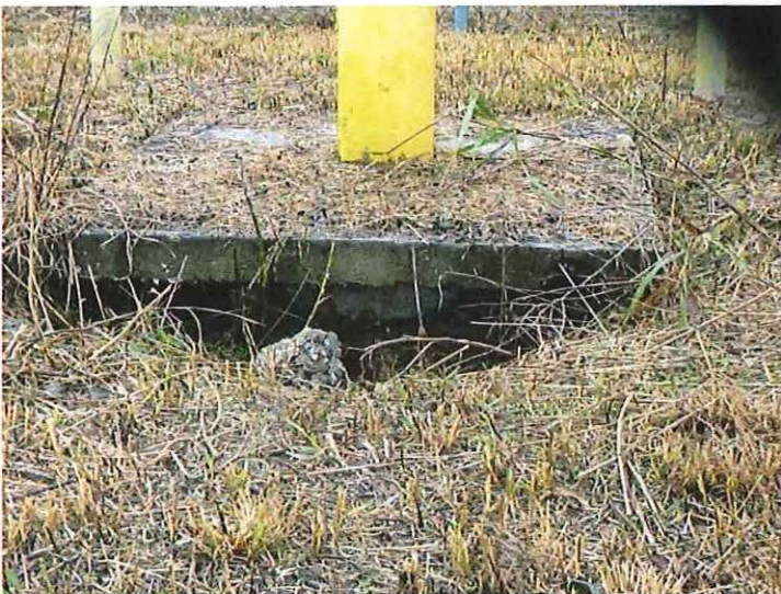
Soil erosion under concrete pad for MA-06
