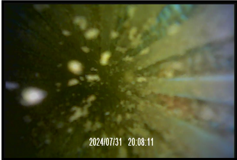
PS10A – sediment along screen loosened by camera drag
