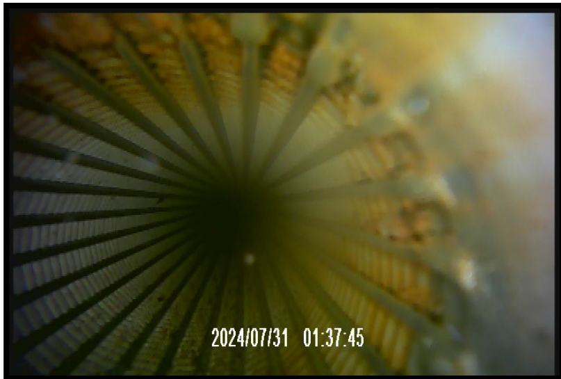
MW402S – some rust near top of screen
