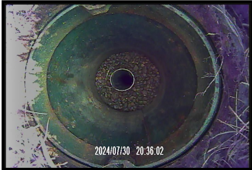
MW401S – well in the flush mount
