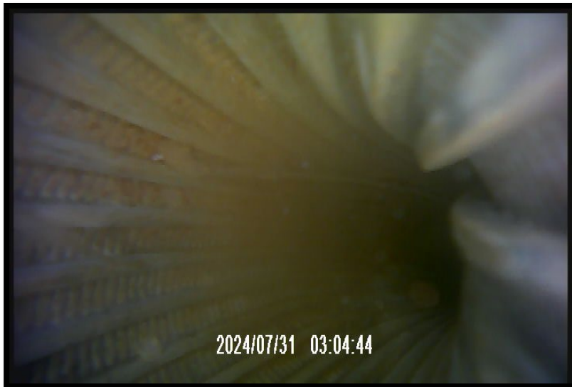
PS4 – clear bend in screen, camera could not pass
