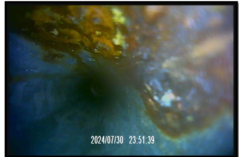
COP3 – heavy rusting above water table
