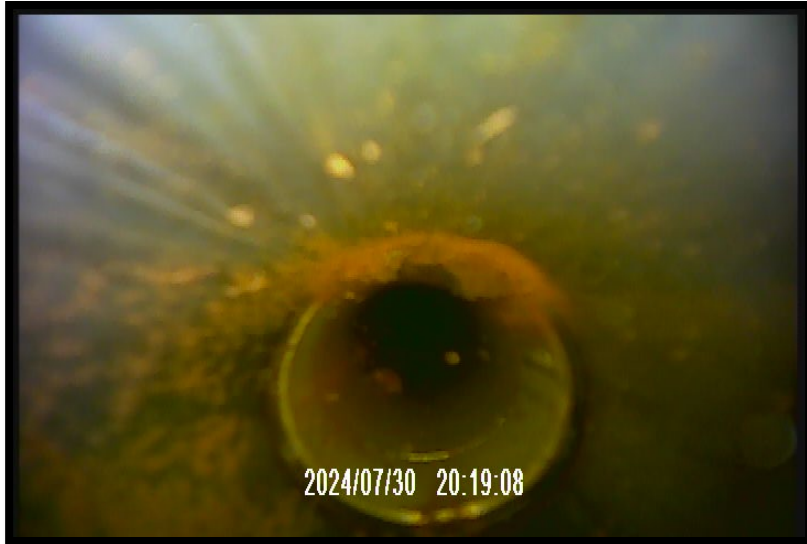
MW401D – sediment buildup around joint
