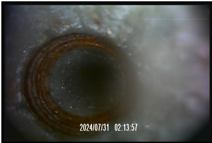
PS6 – rusty joint
