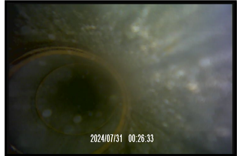
MW205DR – off center, joint below water table
