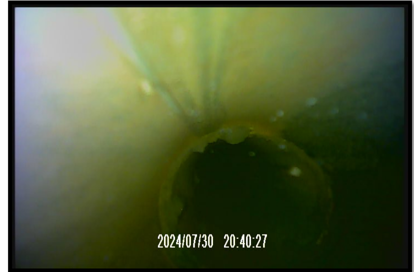
MW401S – some buildup around joint
