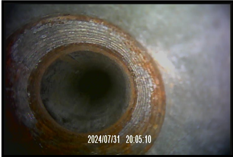
PS10A – rusty joint
