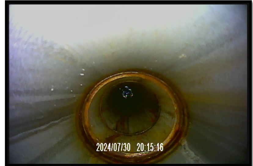
MW401D – Rusting around joint
