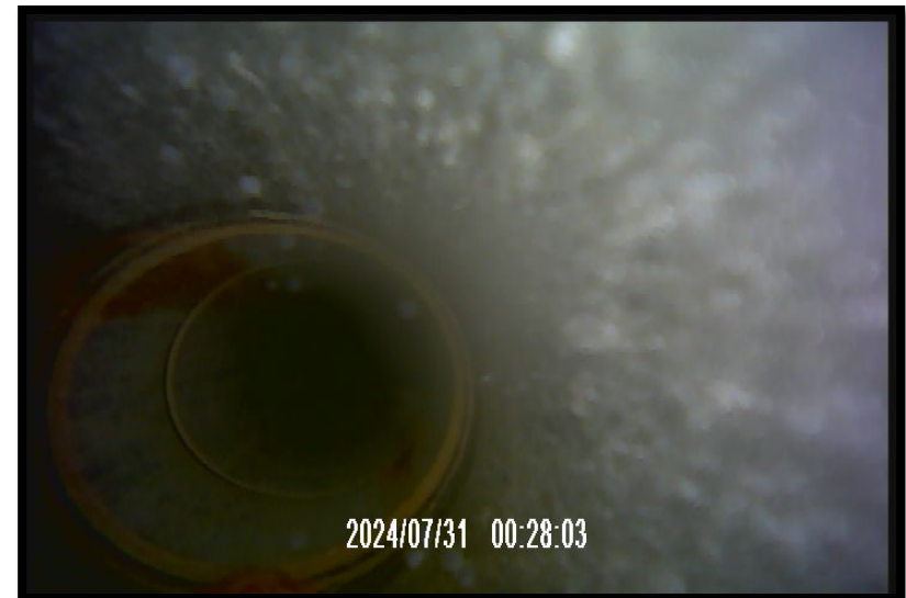
MW205DR - off center, joint below water table
