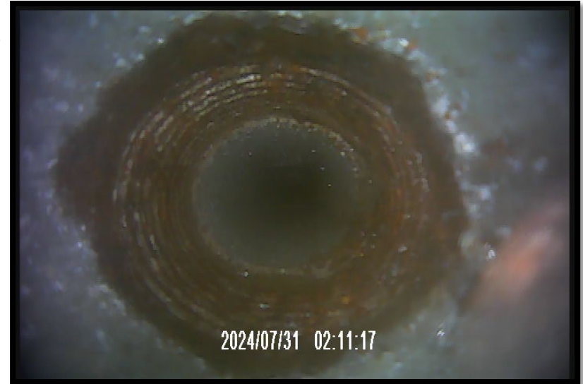
PS6 – rusty joint
