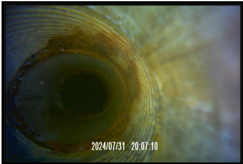
PS10A – rusty joint
