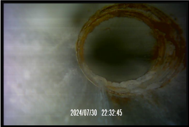
PS105D – joint, camera cut out approx. 60 ft.
