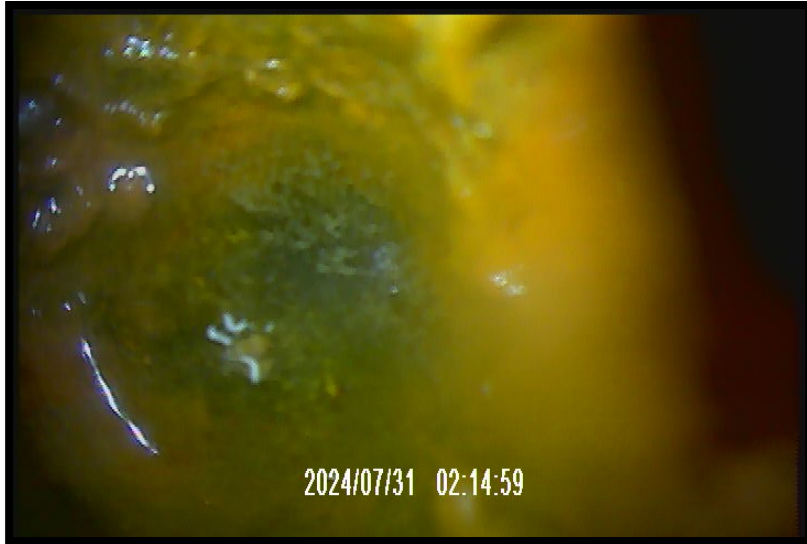
PS6 – buildup around a joint
