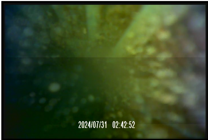
PSBS – screen appears lightly rusted and silty
