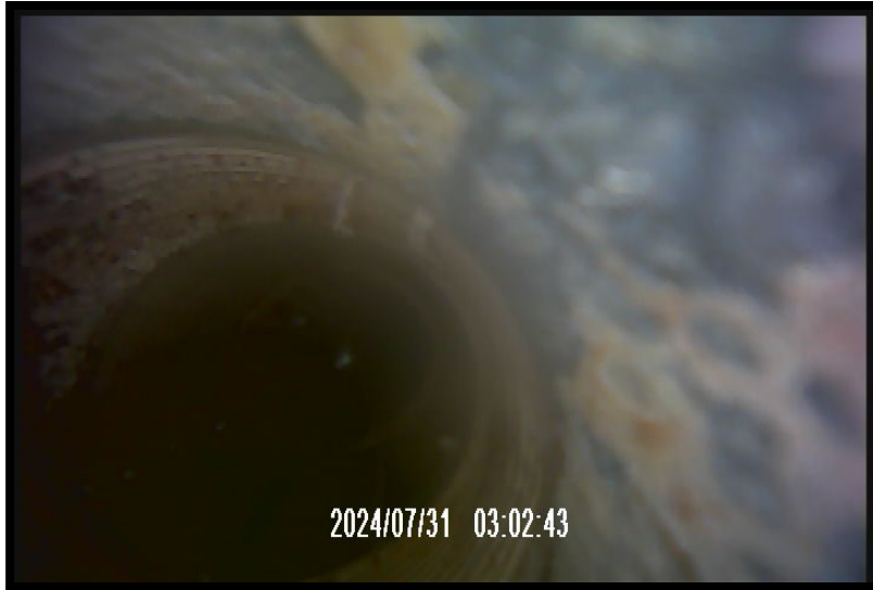
PS4 – rusting near joint
