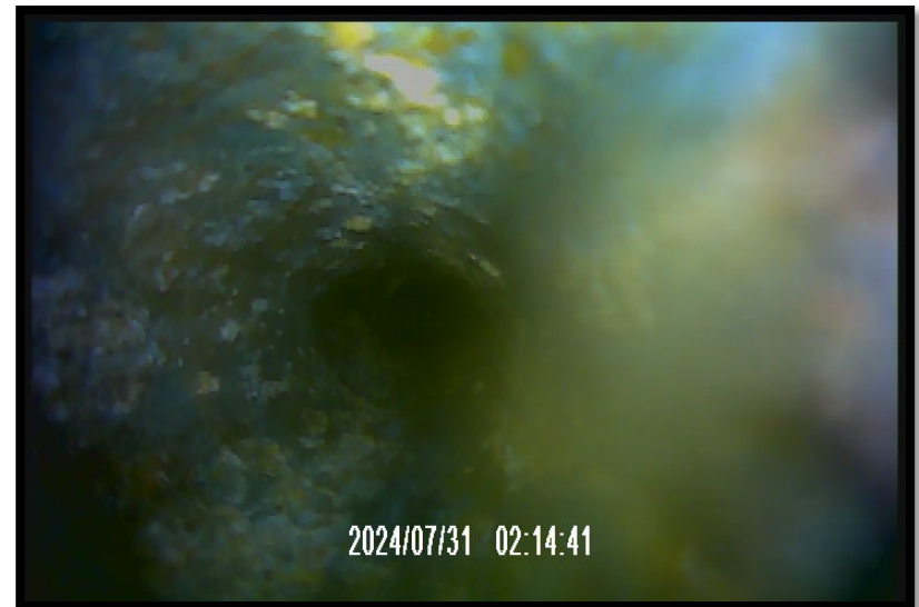
PS6 – casing slight degraded
