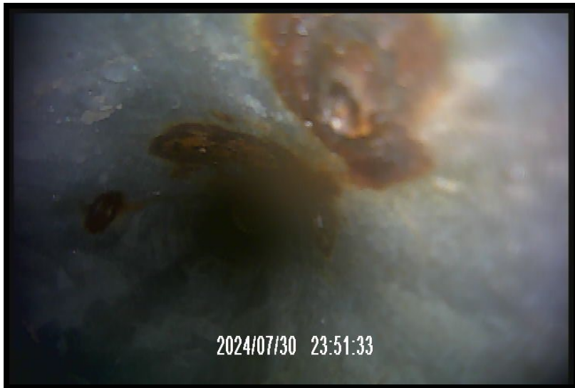
COP3 – rust feature that may be a hole
