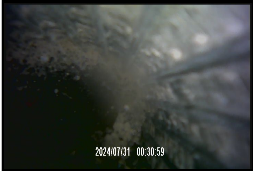
MW205DR – Sediment being knocked off screen by camera, screen in good condition otherwise
