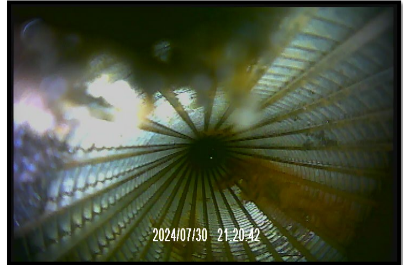
COP5R – little rust lower right side
