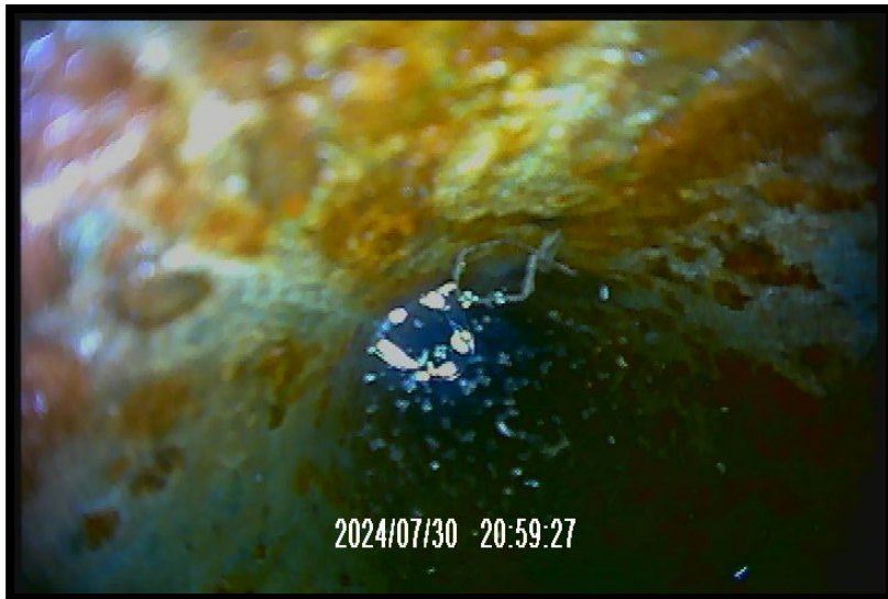
COP1 – heavy rust above water table
