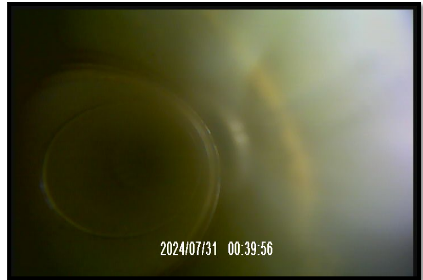
MW205SR – poor visibility, joint
