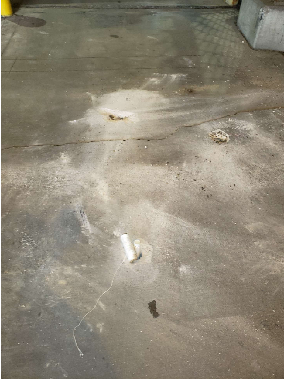
Figure 4: Holes C' (C'X) (upper), C (CX) (right), and C'' (with pipe and spool) (looking north)
