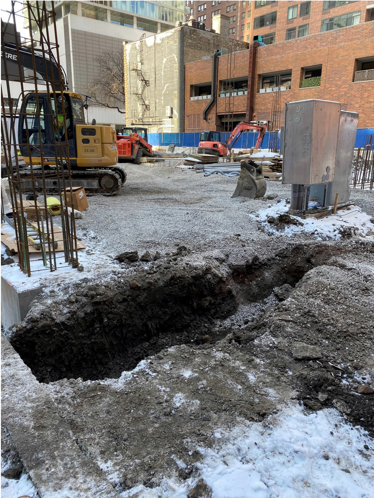
PICTURE 5: WEST-FACING VIEW OF COMPLETED EXCAVATION OF SECTION 6 AT 210-225 E. GRAND AVE.
