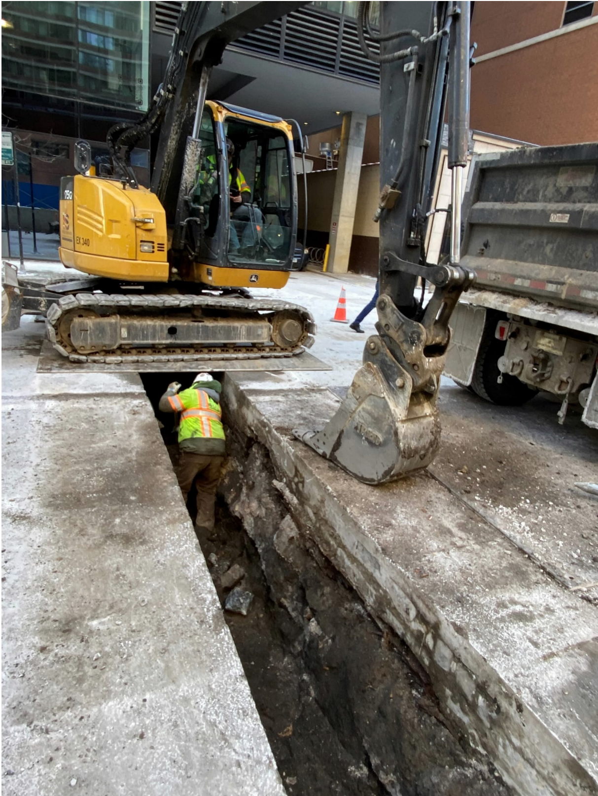
PICTURE 2: SOUTH-FACING VIEW OF COMPLETED EXCAVATION OF SECTION 3 AT 210-225 E. GRAND AVE.
