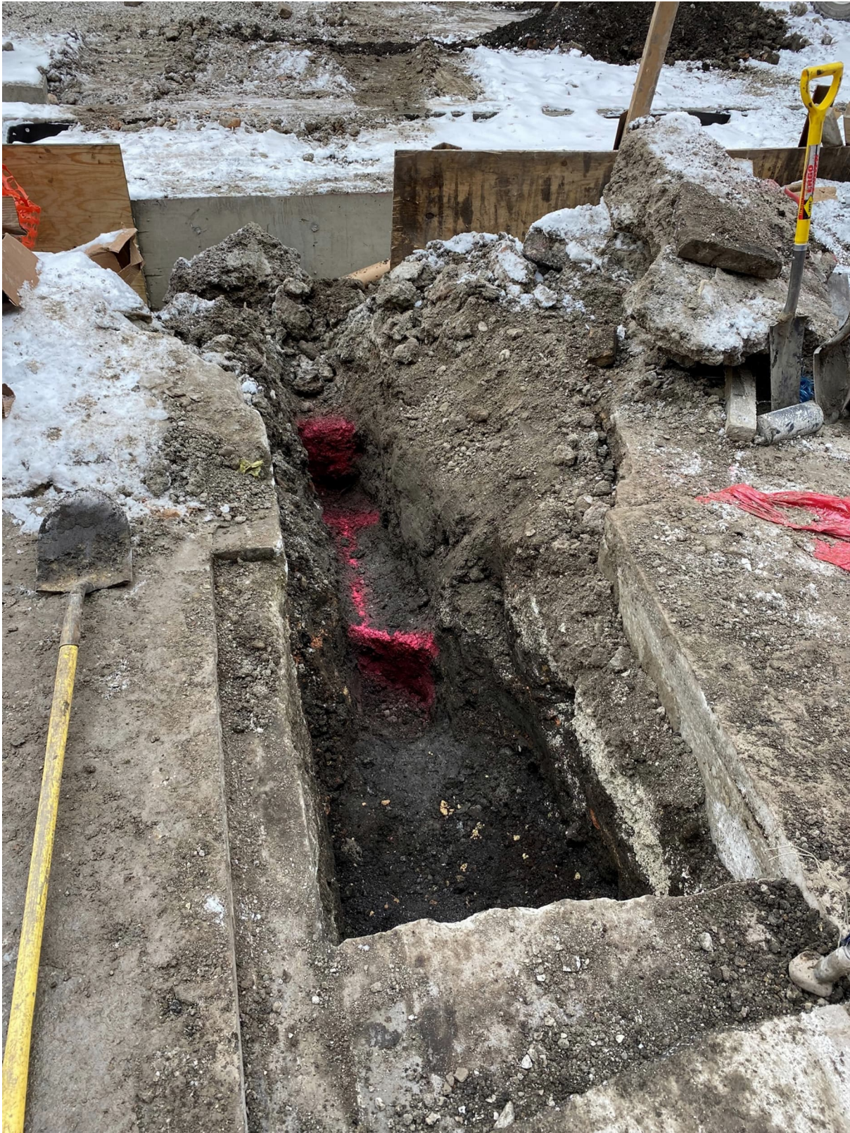
PICTURE 4: NORTH-FACING VIEW OF COMPLETED EXCAVATION OF SECTION 5 AT 210-225 E. GRAND AVE.
