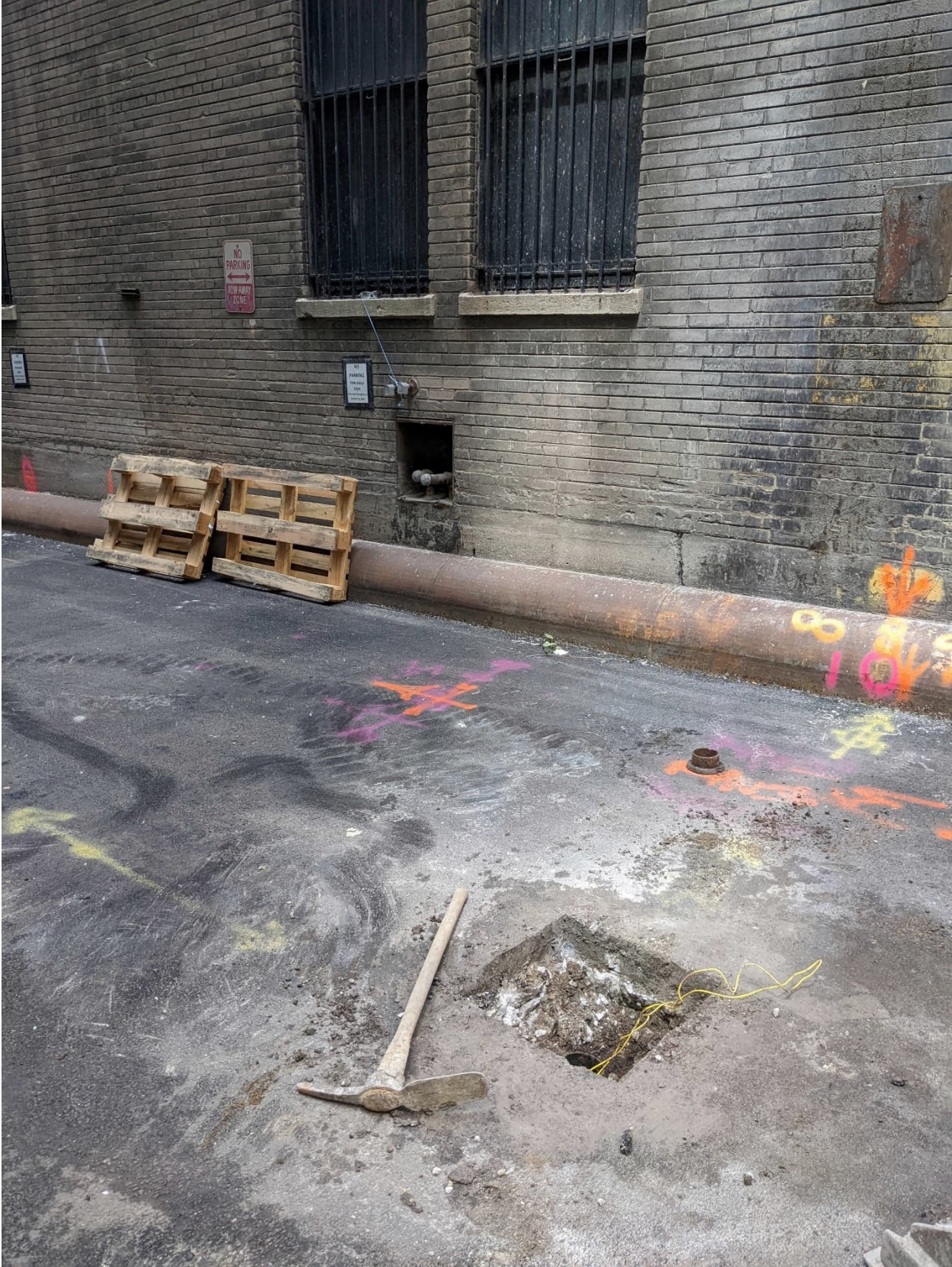
PICTURE 1: VIEW OF THE COMPLETED DAMAGED VALVE REPLACEMENT EXCAVATION AT 301-311 N MACCHESNEY COURT
