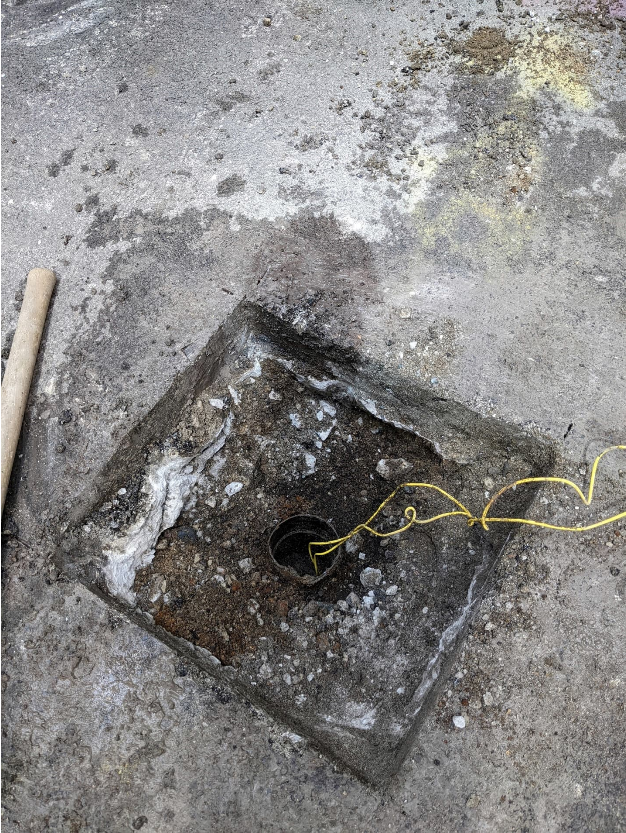
PICTURE 2: VIEW OF THE COMPLETED DAMAGED VALVE REPLACEMENT EXCAVATION AT 301-311 N MACCHESNEY COURT (CLOSE)
