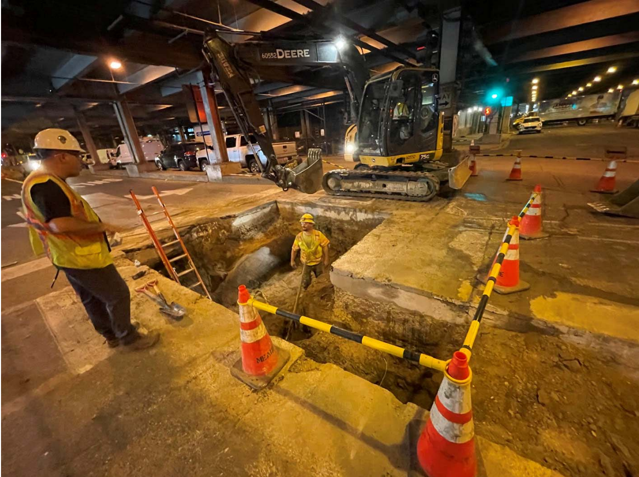
PICTURE 3: VIEW OF THE COMPLETED EXCAVATION ON LOWER MICHIGAN AVE TO ACCESS GAS MAIN LOOKING SOUTHEAST (JUNE 21, 2022)
