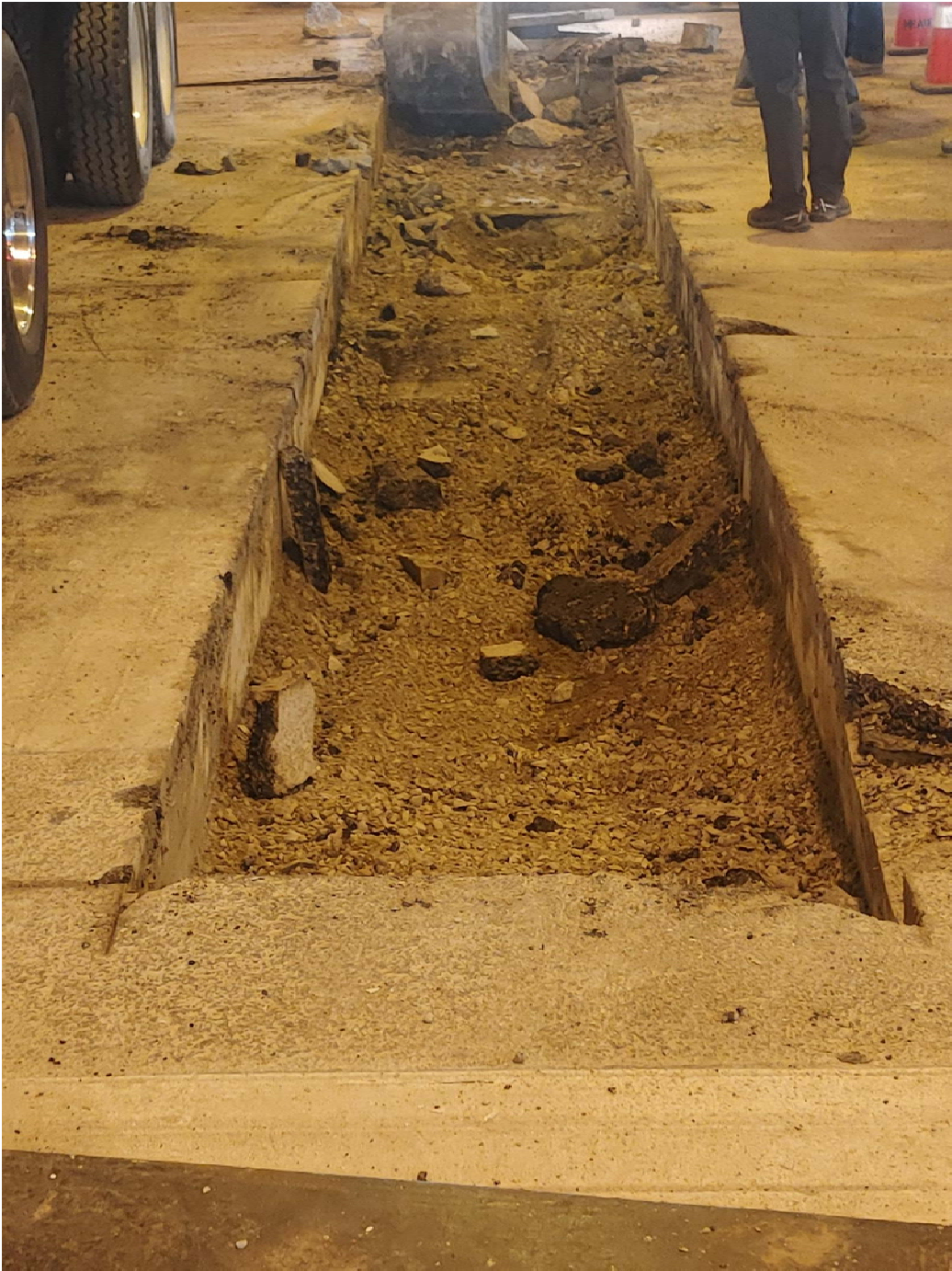
PICTURE 1: VIEW OF THE TRENCH LOOKING SOUTH DOWN LOWER MICHIGAN AVENUE AFTER CONCRETE REMOVAL (MAY 17, 2022)
