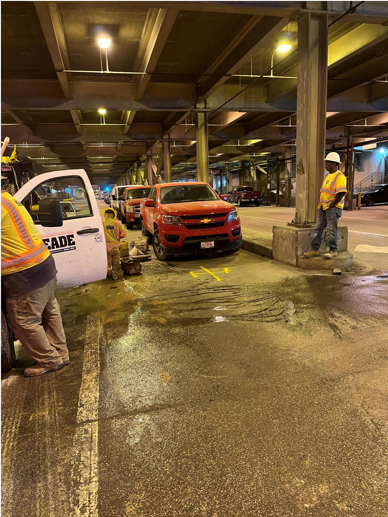
PICTURE 1: VIEW OF THE COMPLETED CORROSION PROTECTION EXCAVATION AT 325 N MICHIGAN AVE LOOKING SOUTH
