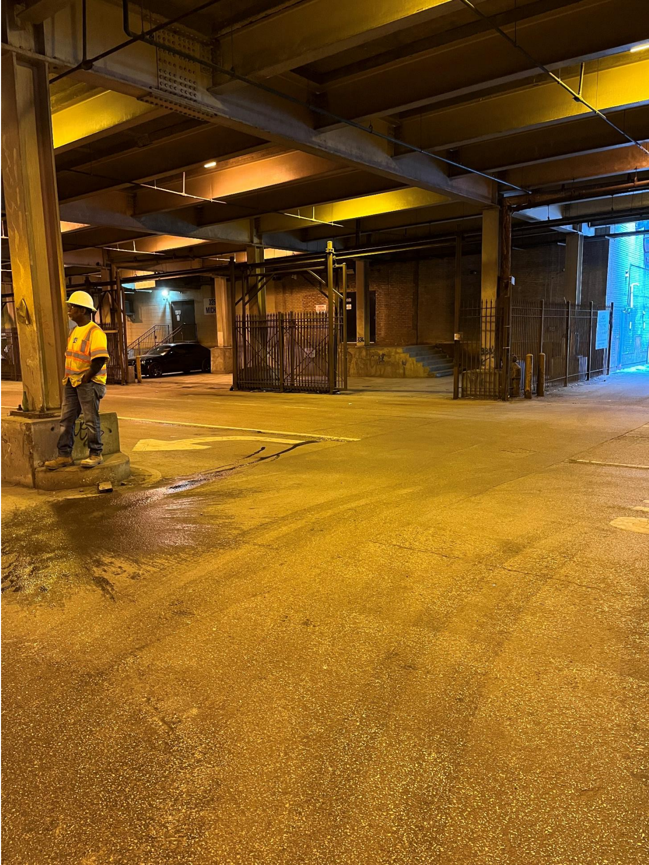
PICTURE 2: VIEW OF THE COMPLETED CORROSION PROTECTION EXCAVATION AT 325 N MICHIGAN AVE LOOKING SOUTHWEST
