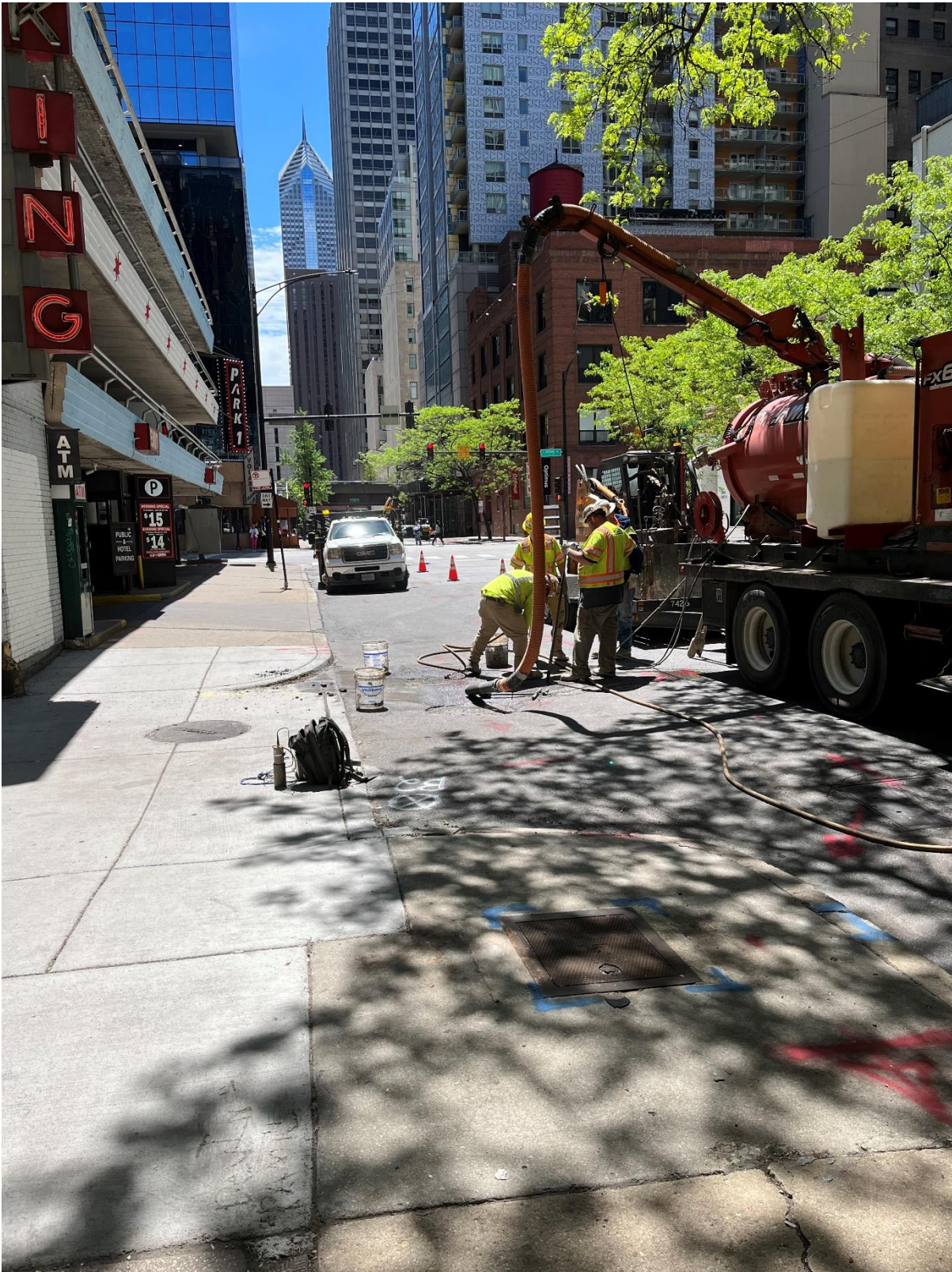
PICTURE 3: VIEW OF THE COMPLETED CORROSION PROTECTION EXCAVATION AT 550 N ST CLAIR LOOKING SOUTH
