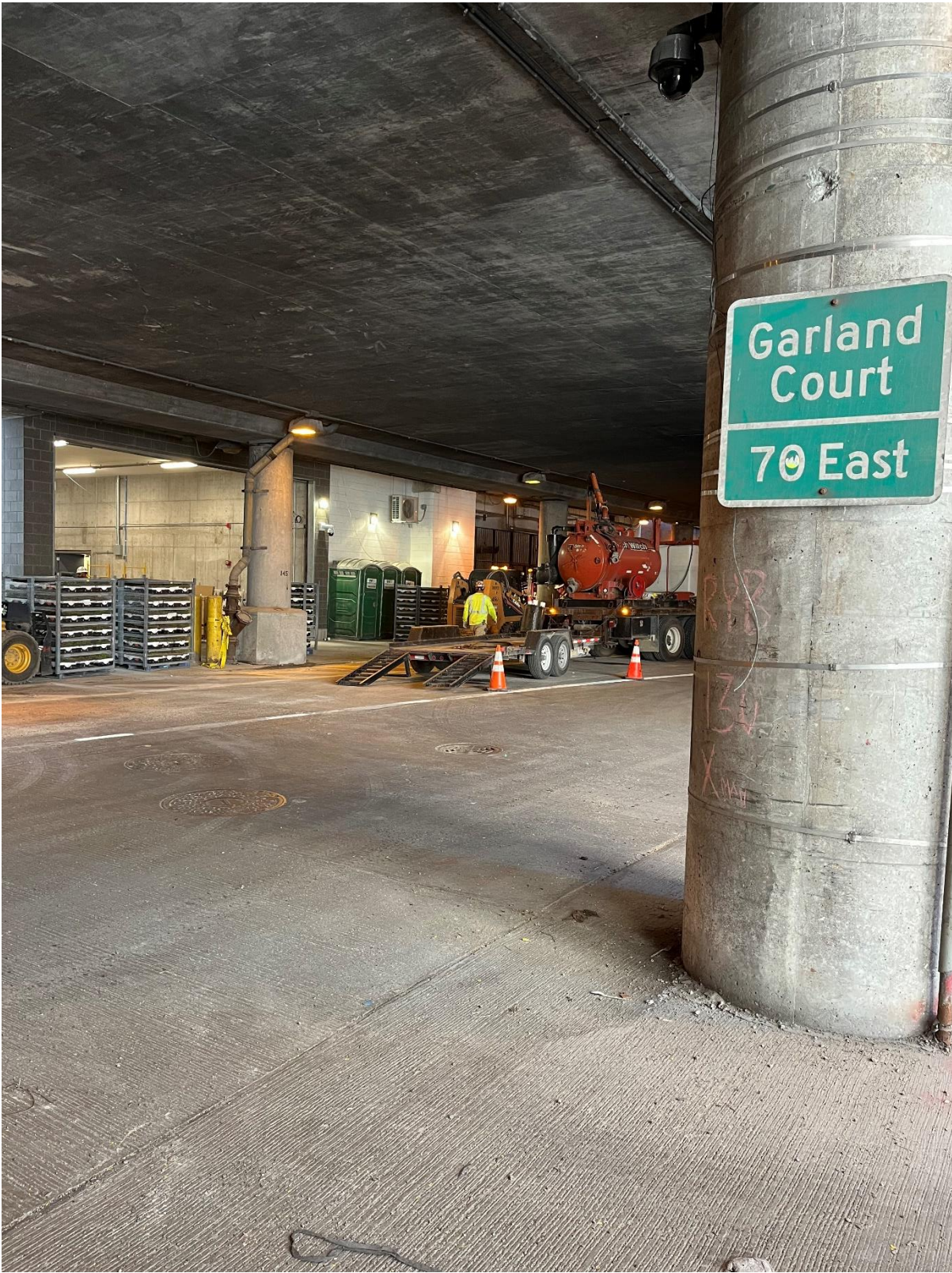
PICTURE 5: VIEW OF THE COMPLETED CORROSION PROTECTION EXCAVATION AT 74-78 E LOWER WACKER PLACE LOOKING NORTH EAST
