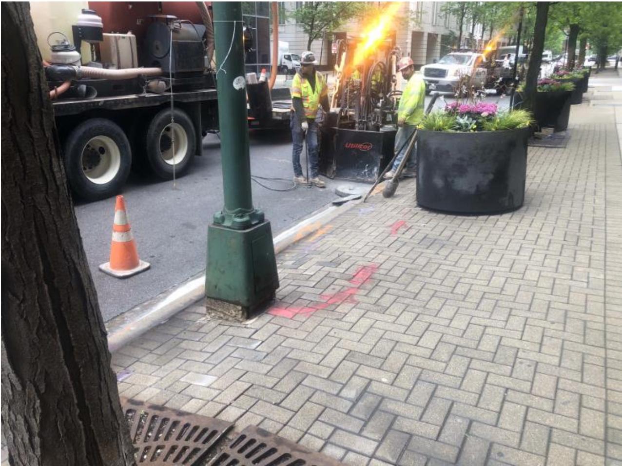
PICTURE 7: VIEW OF THE COMPLETED CORROSION PROTECTION EXCAVATION AT 100 EAST ERIE ST
