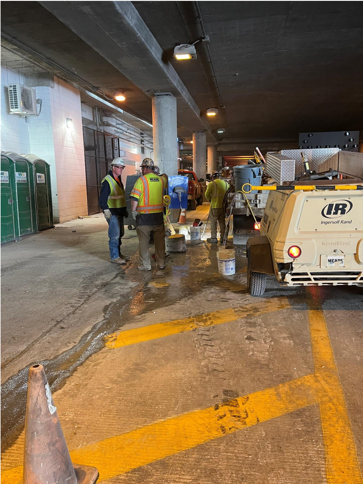
PICTURE 4: VIEW OF THE COMPLETED CORROSION PROTECTION EXCAVATION AT 74-78 E LOWER WACKER PLACE LOOKING EAST
