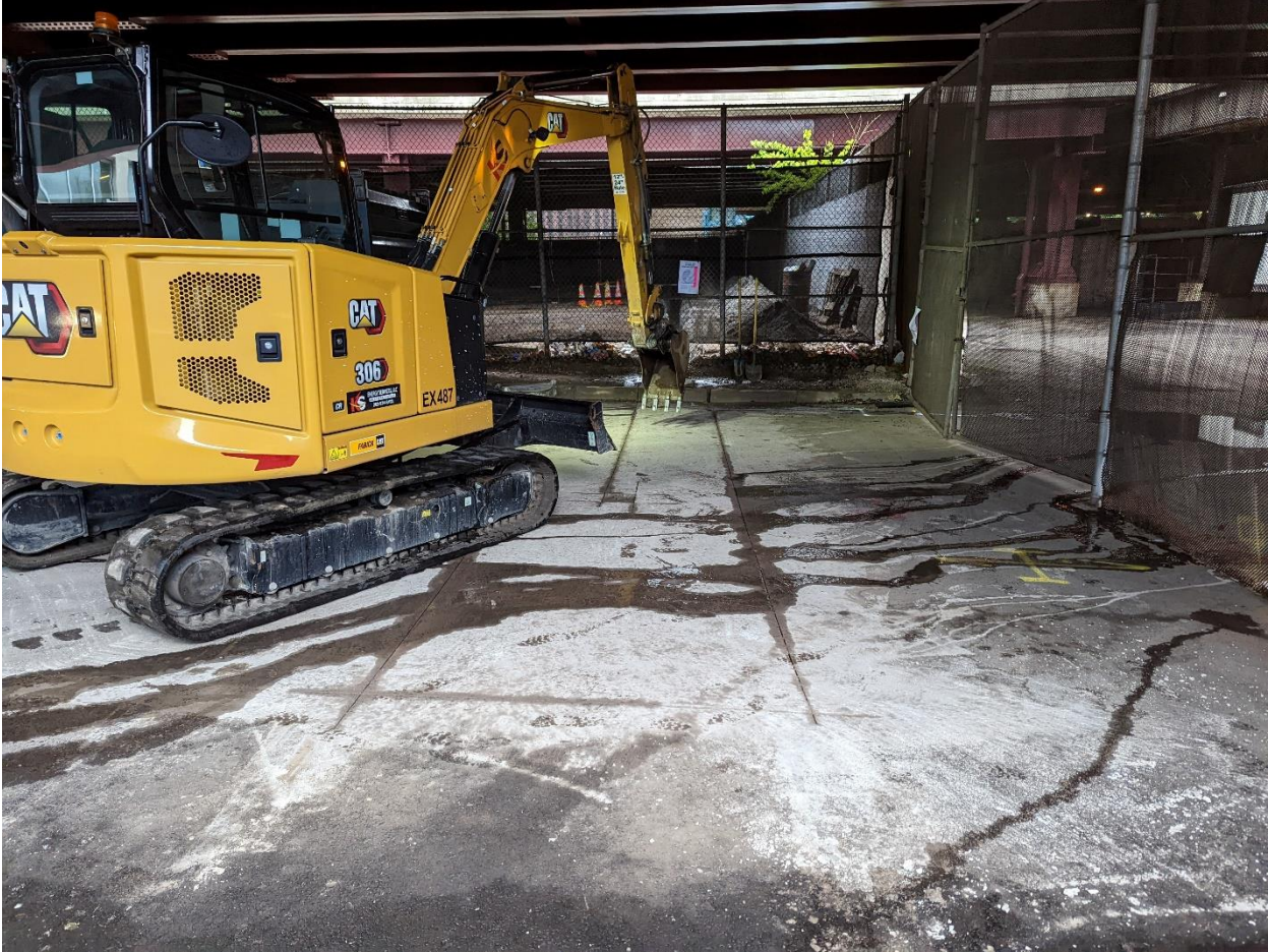
PICTURE 3: VIEW OF THE UNION JOINT AREA OF THE EXCAVATION AT 485 EAST CHICAGO RIVERWALK
