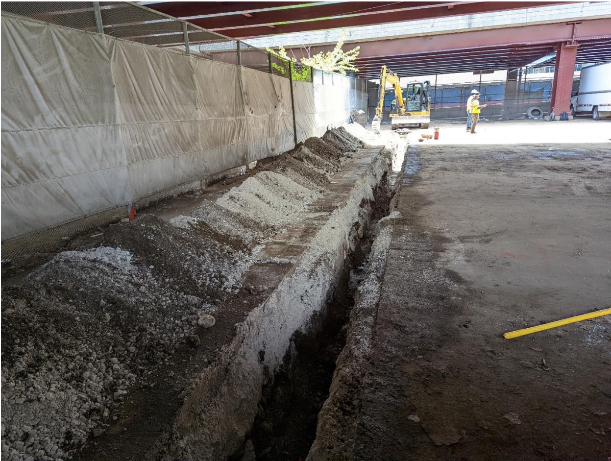
PICTURE 2: VIEW OF THE COMPLETED CORROSION PROTECTION EXCAVATION AT 485 EAST CHICAGO RIVERWALK
