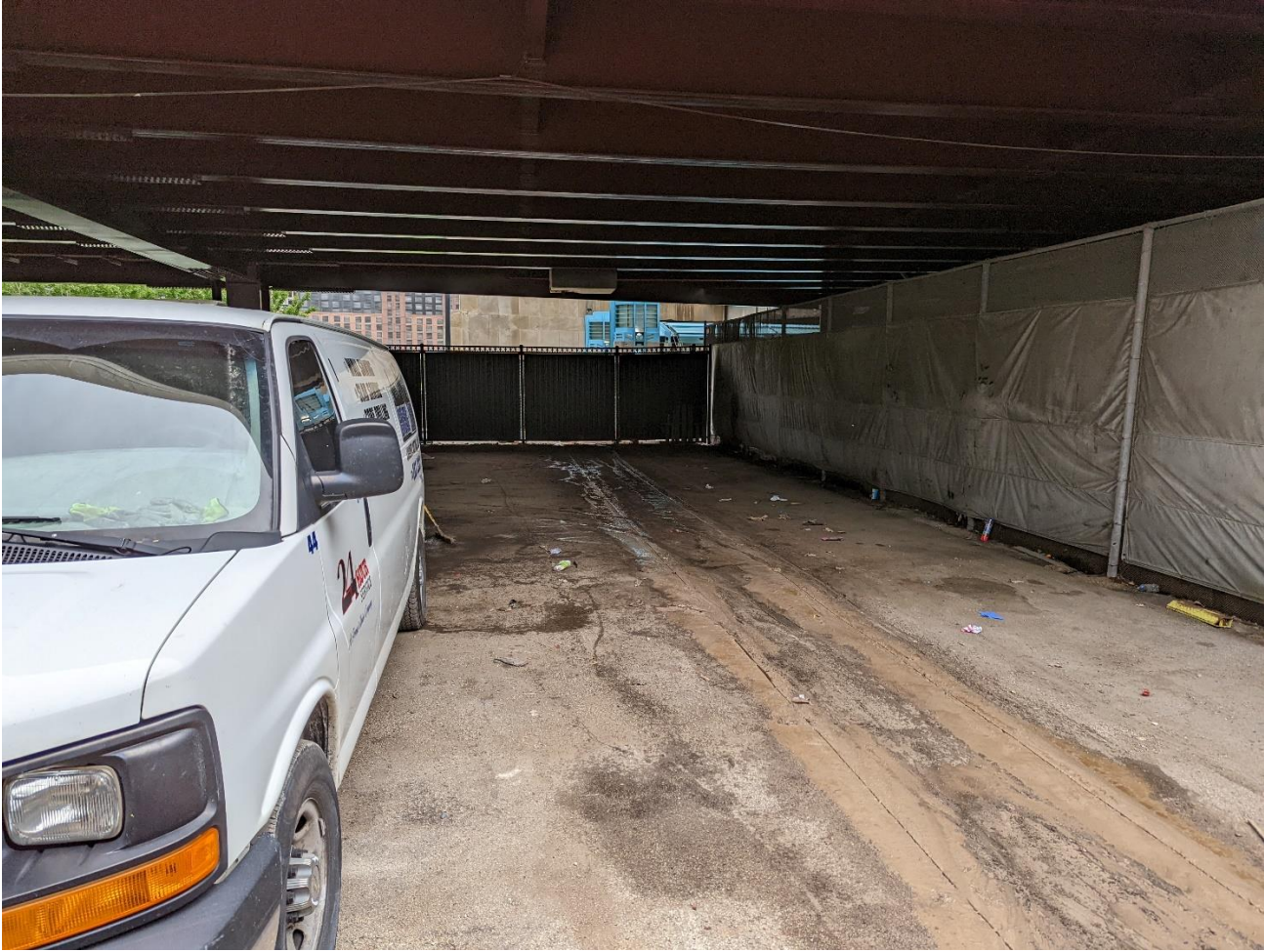
PICTURE 1: VIEW OF THE CUT TRENCH AREA PRIOR TO EXCAVATION AT 485 EAST CHICAGO RIVERWALK
