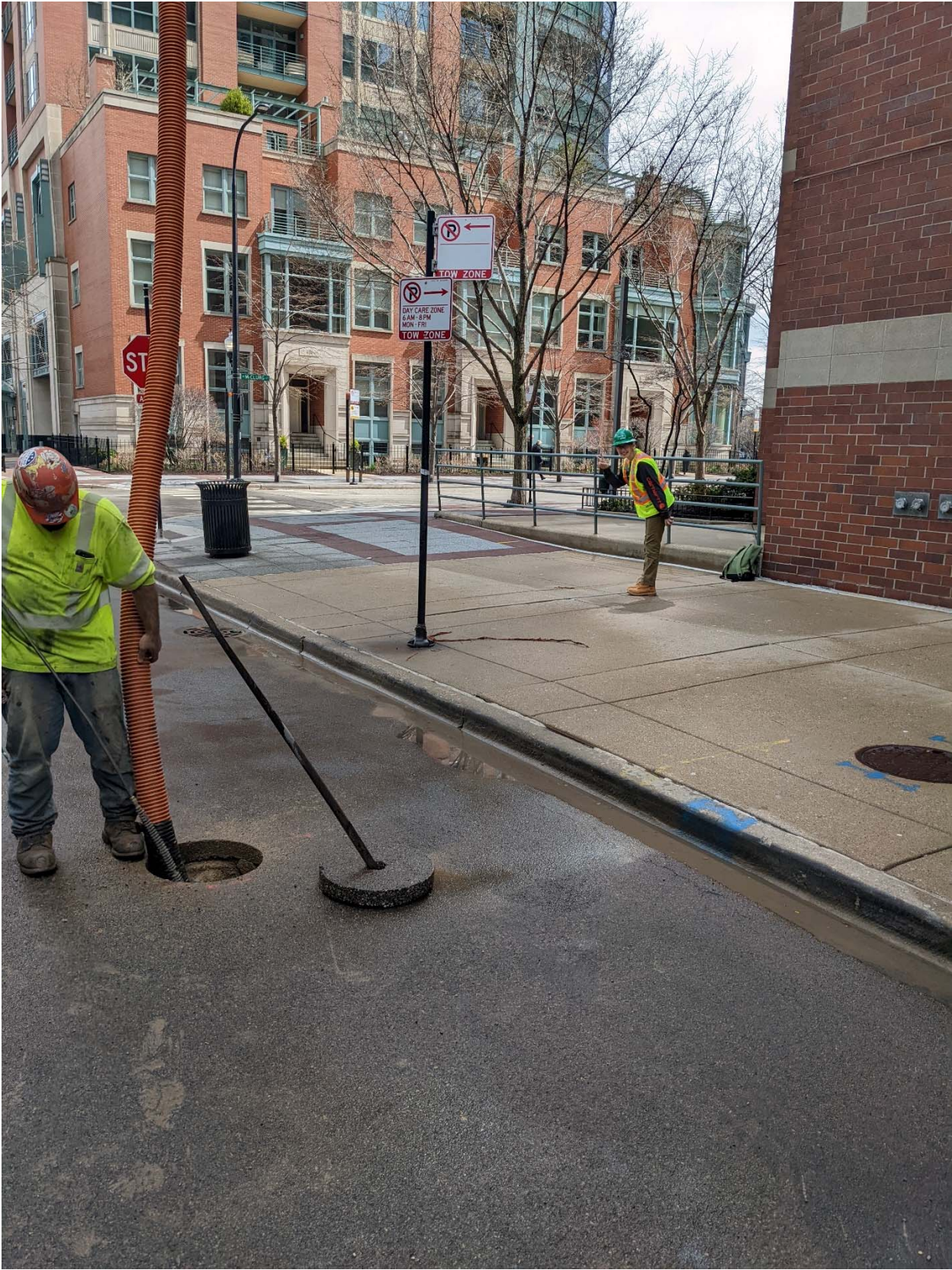
PICTURE 3: VIEW OF THE COMPLETED CORROSION PROTECTION EXCAVATION 1 AT 358-59 E NORTH WATER ST.
