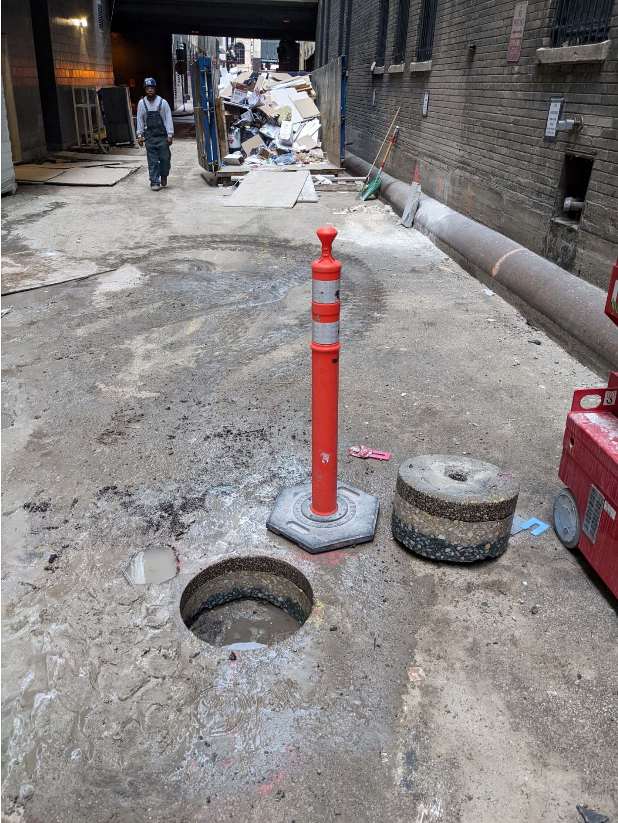
PICTURE 1: VIEW OF THE COMPLETED CORROSION PROTECTION EXCAVATION AT 301-06 N MICHIGAN AVE
