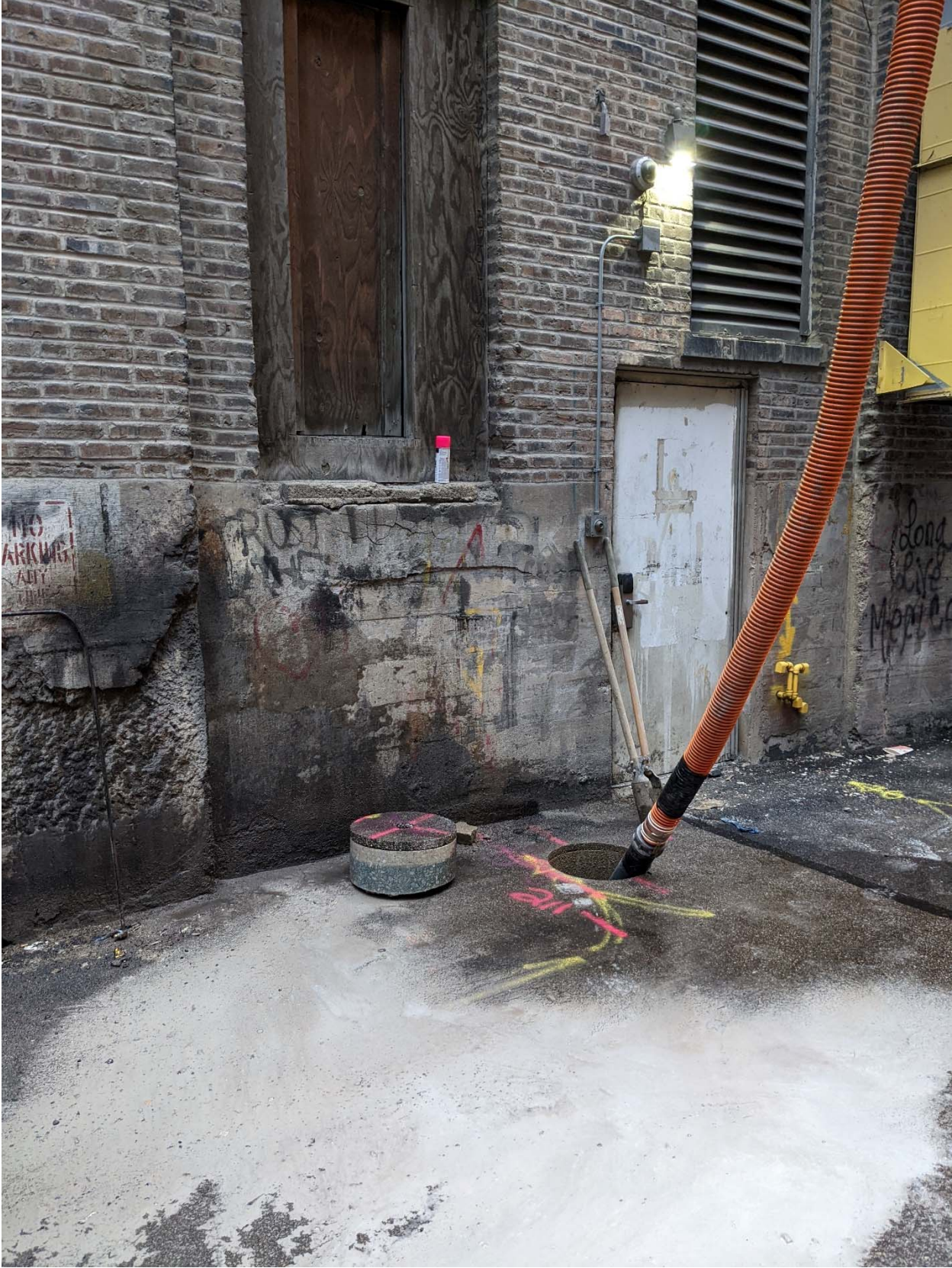
PICTURE 2: VIEW OF THE COMPLETED CORROSION PROTECTION EXCAVATION AT 320-25 N MACCHESNEY CT.
