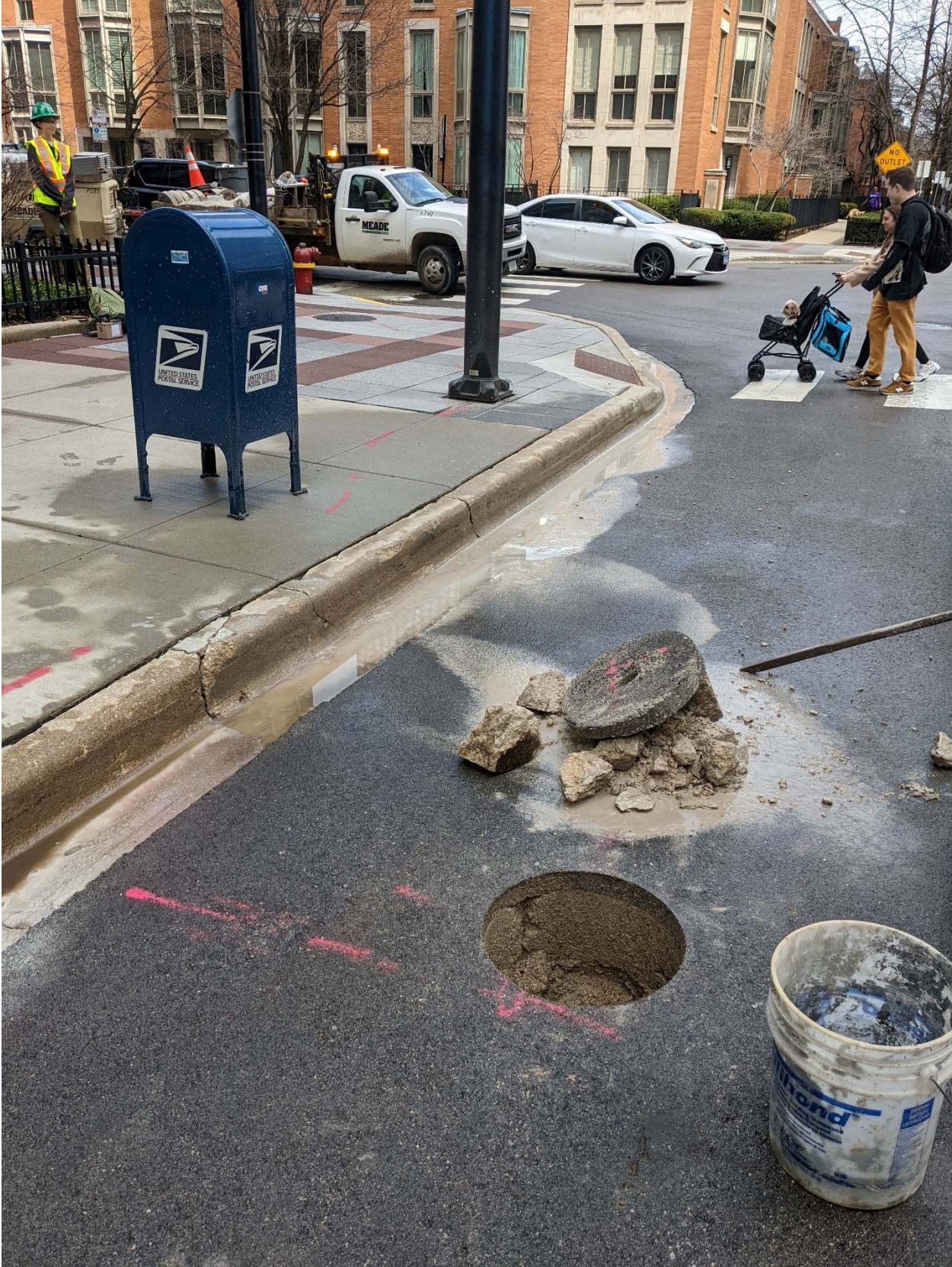
PICTURE 4: VIEW OF THE COMPLETED CORROSION PROTECTION EXCAVATION 2 AT 358-59 E NORTH WATER ST.
