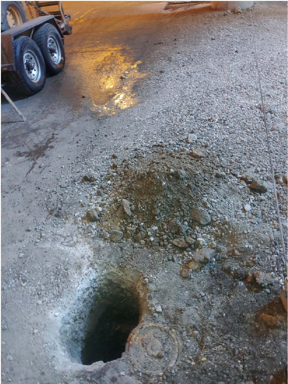
PICTURE 1: VIEW OF THE COMPLETED CORROSION PROTECTION EXCAVATION AT 150-53 N. FIELD BLVD.
