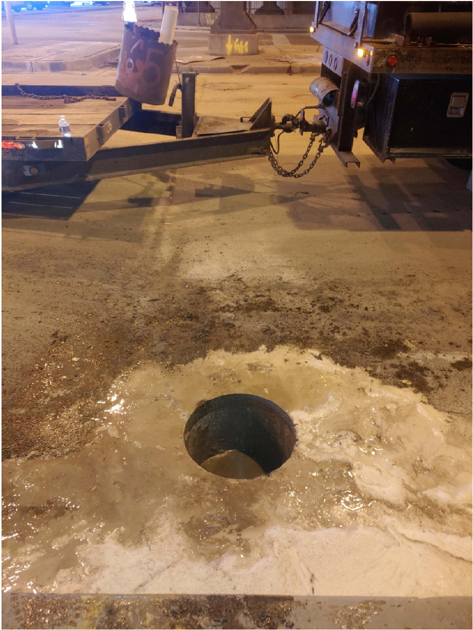
PICTURE 2: VIEW OF THE COMPLETED CORROSION PROTECTION EXCAVATION AT 236-48 N. COLUMBUS DR.
