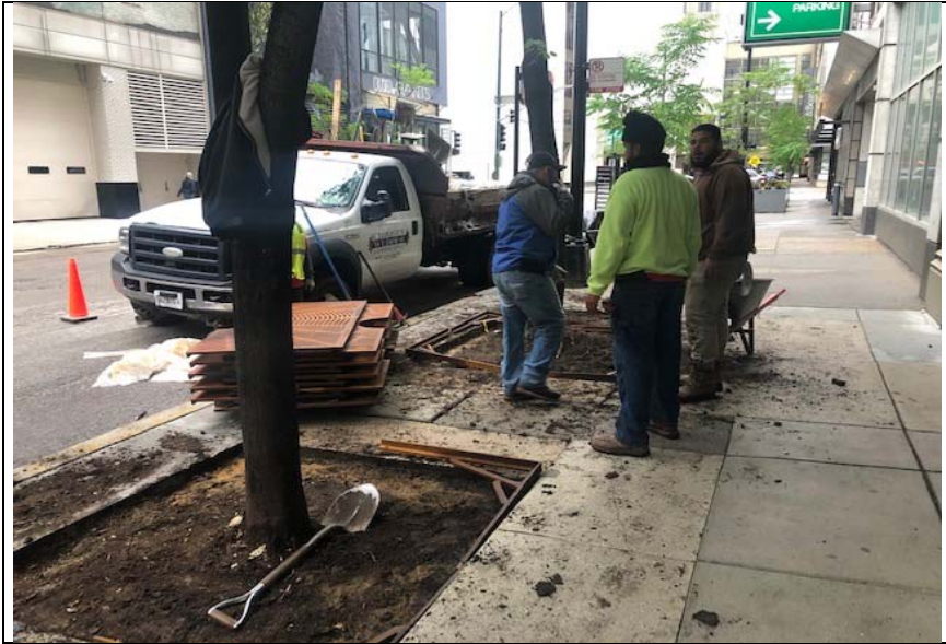
Photo 1: Looking south as workers excavate soils in Planter Areas #1 and #2 after screening. 5/28/21
