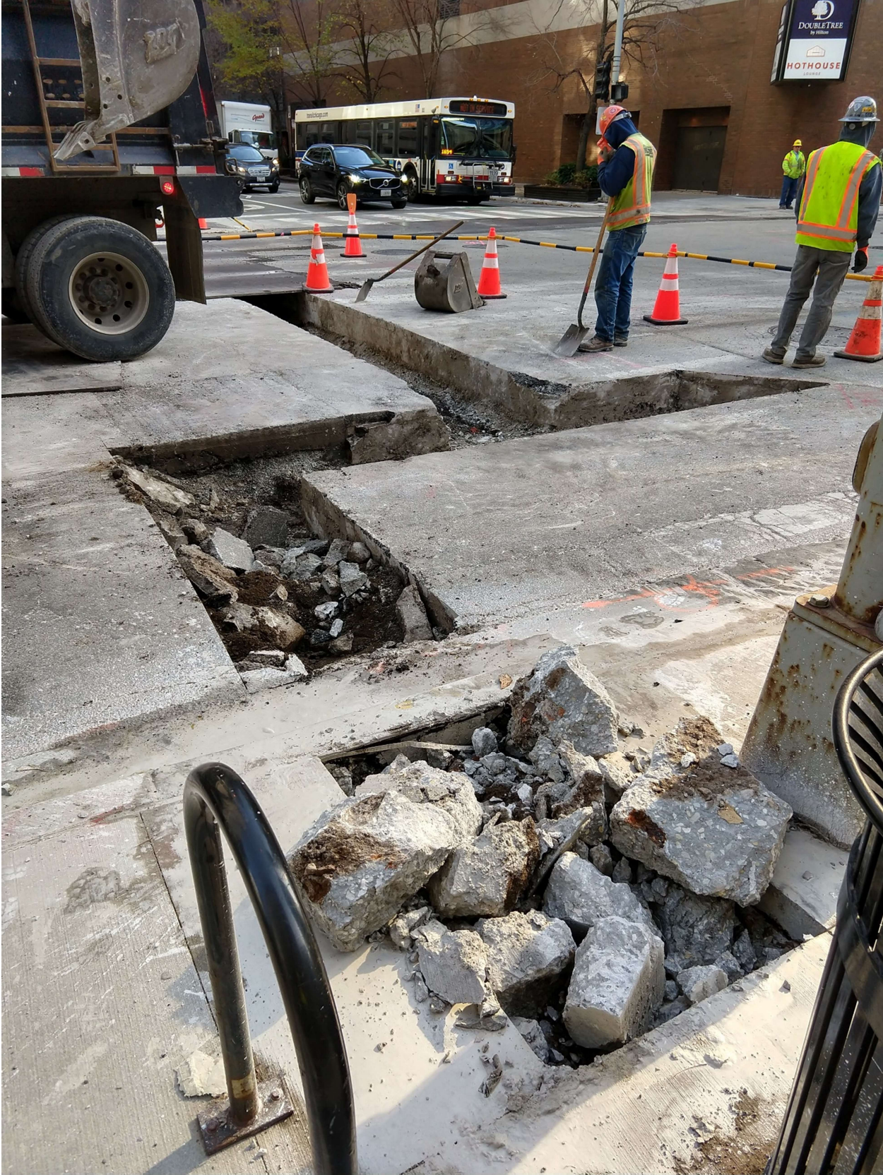
PICTURE 1: VIEW OF THE EXCAVATION AT INTERSECTION OF FARIBANKS CT. AND ONTARIO ST., LOOKING SOUTHEAST.
