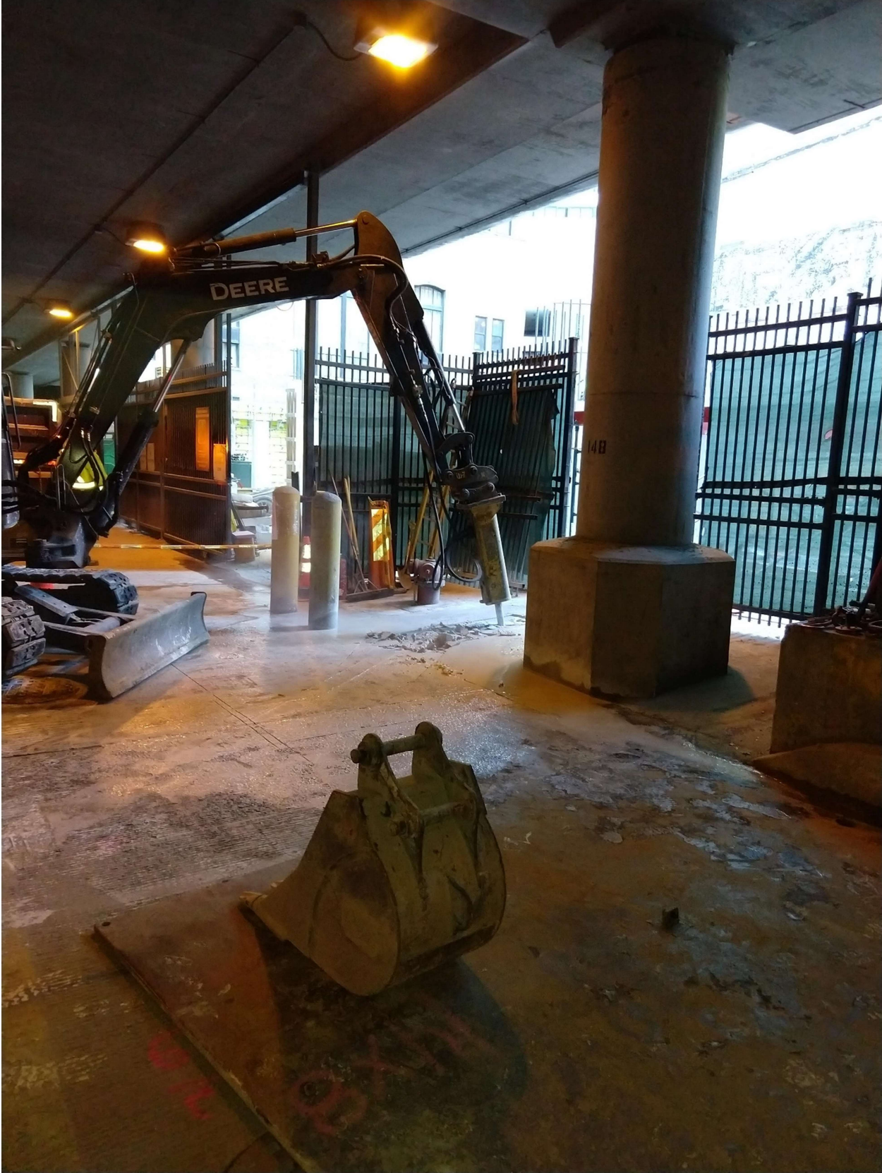
PICTURE 1: VIEW OF THE EXCAVATION AT 80 E. LOWER WACKER PLACE, LOOKING NORTHWEST FROM LOWER MICHIGAN AVENUE.
