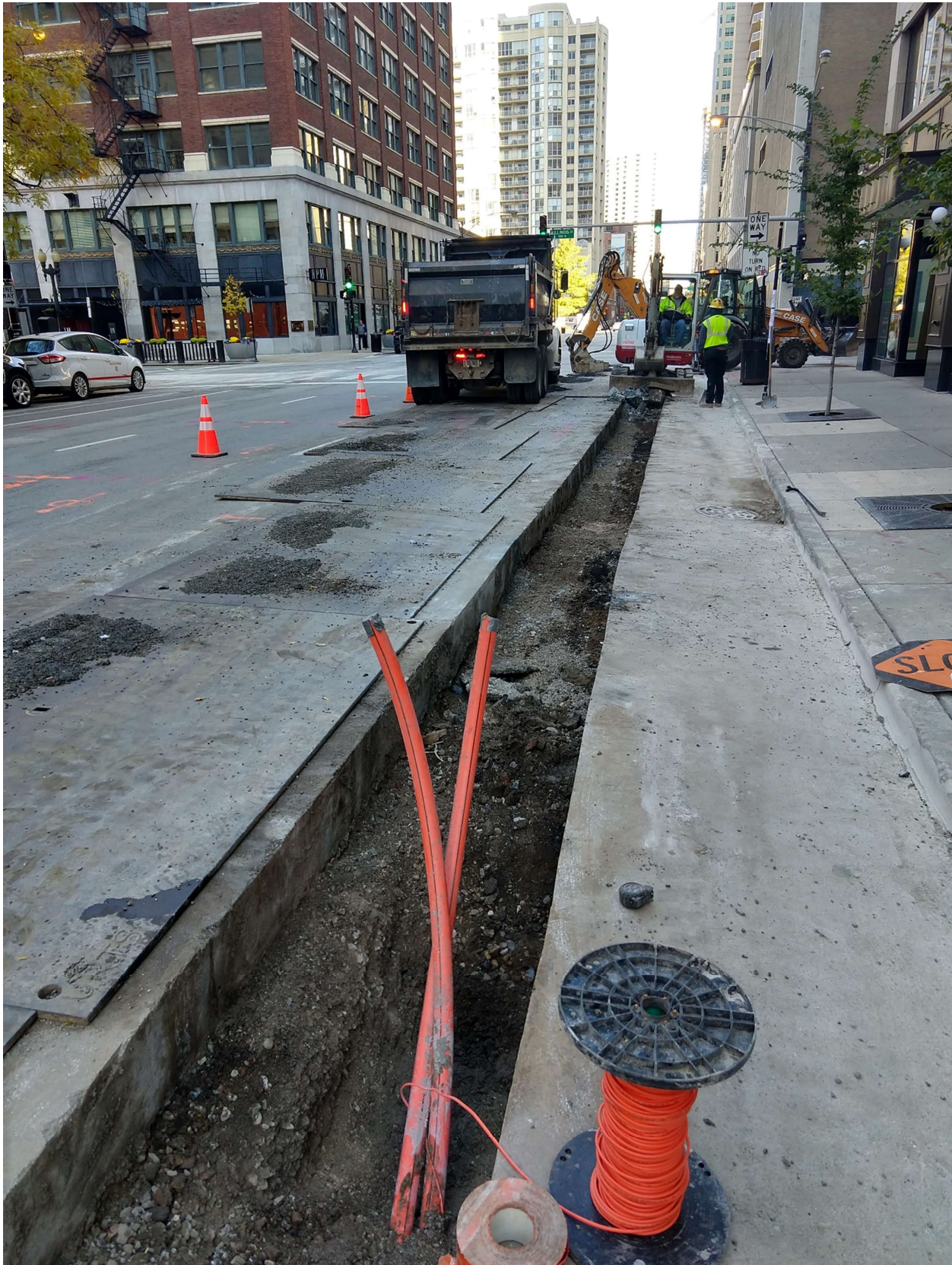
PICTURE 1: VIEW OF THE EXCAVATION AT 440 N. DEARBORN, LOOKING NORTH TOWARDS ILLINOIS ST.
