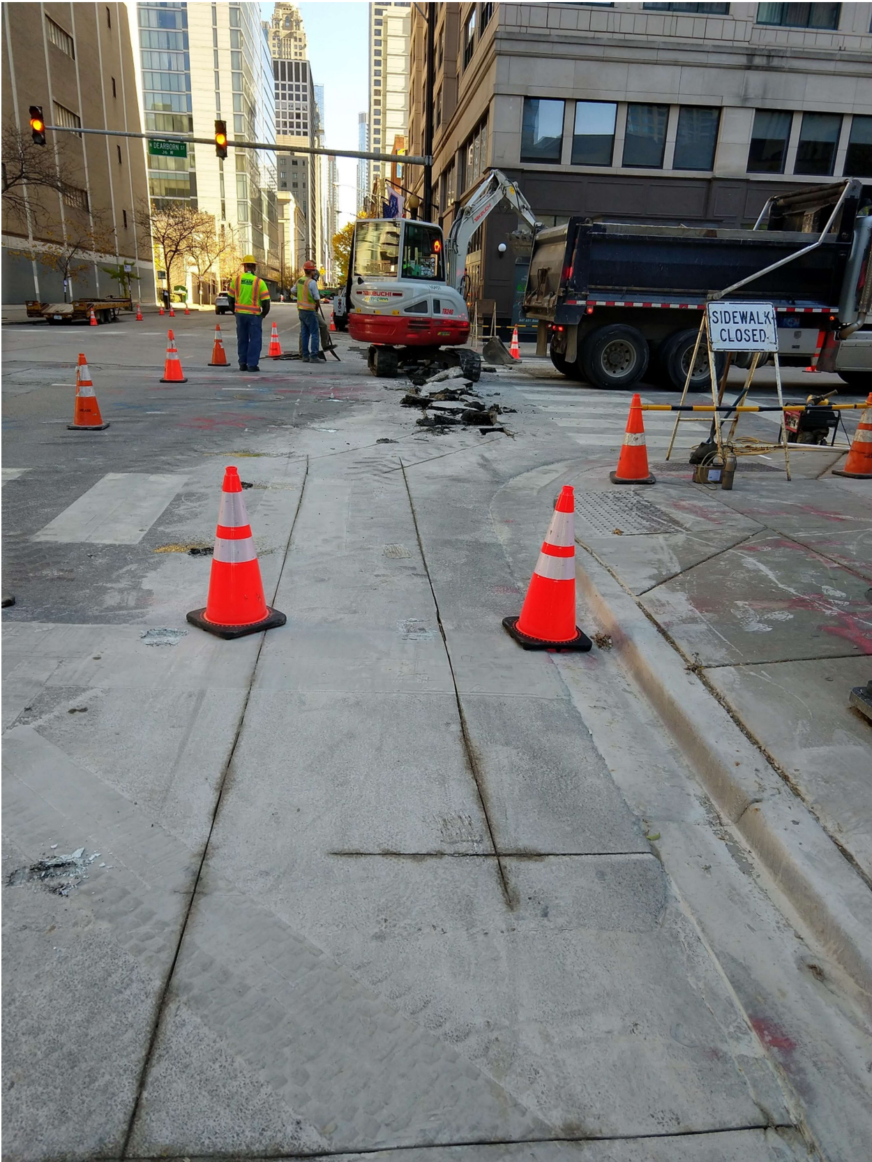
PICTURE 2: VIEW OF THE EXCAVATION AT 40 W. ILLINOIS ST, LOOKING EAST TOWARDS DEARBORN ST.
