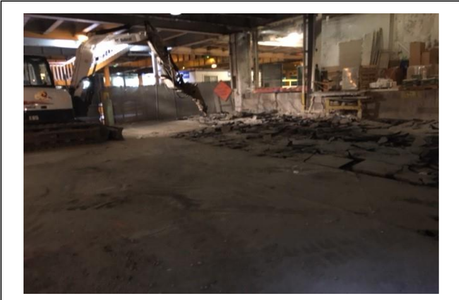
Photo 1: 12/24/2020 - View of Jackhammer and Broken Pavement
