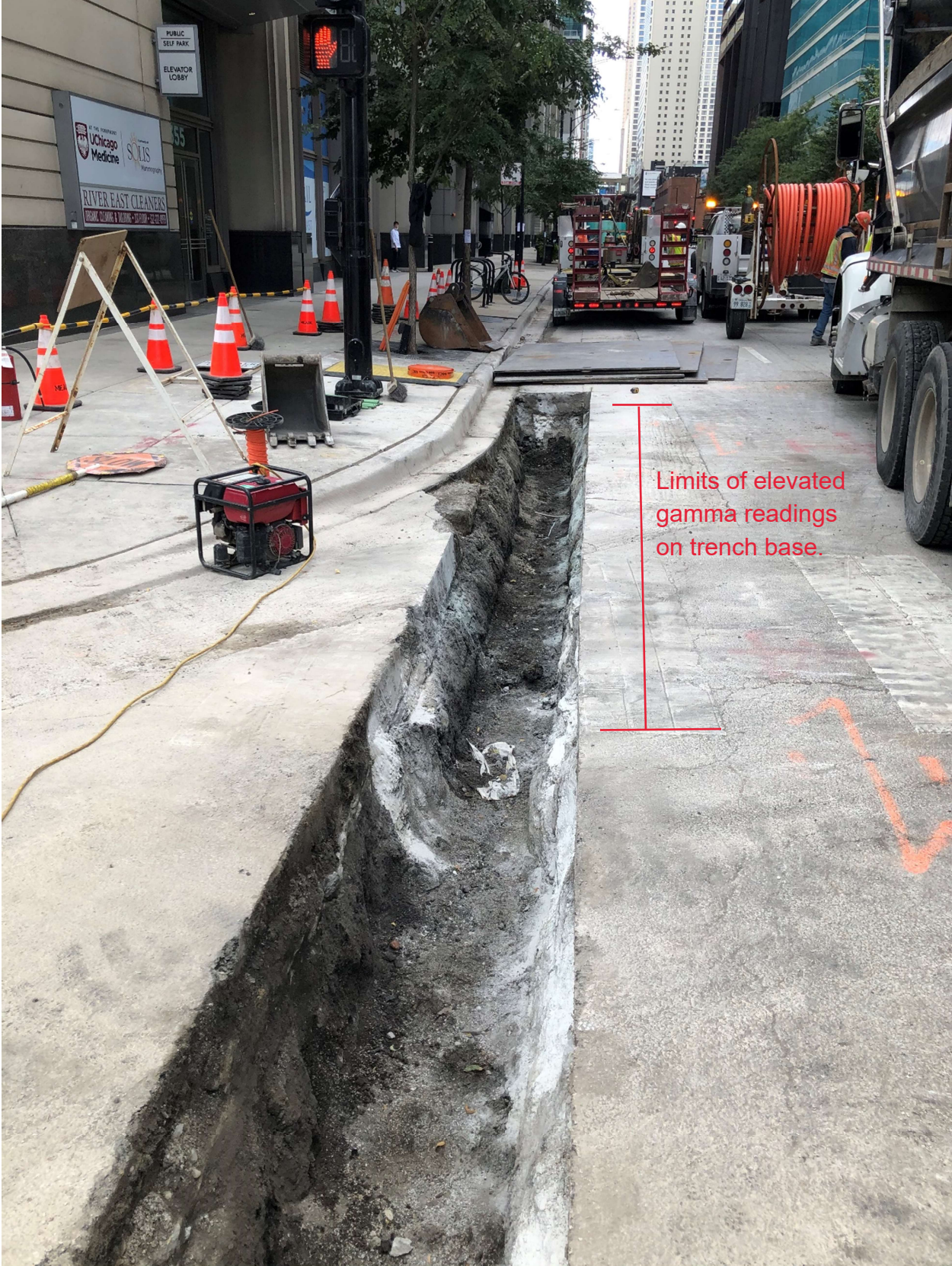
PICTURE 1: VIEW OF THE EXCAVATION AT 353-426 E. GRAND AVE, LOOKING WEST TOWARDS FAIRBANKS AVE.
