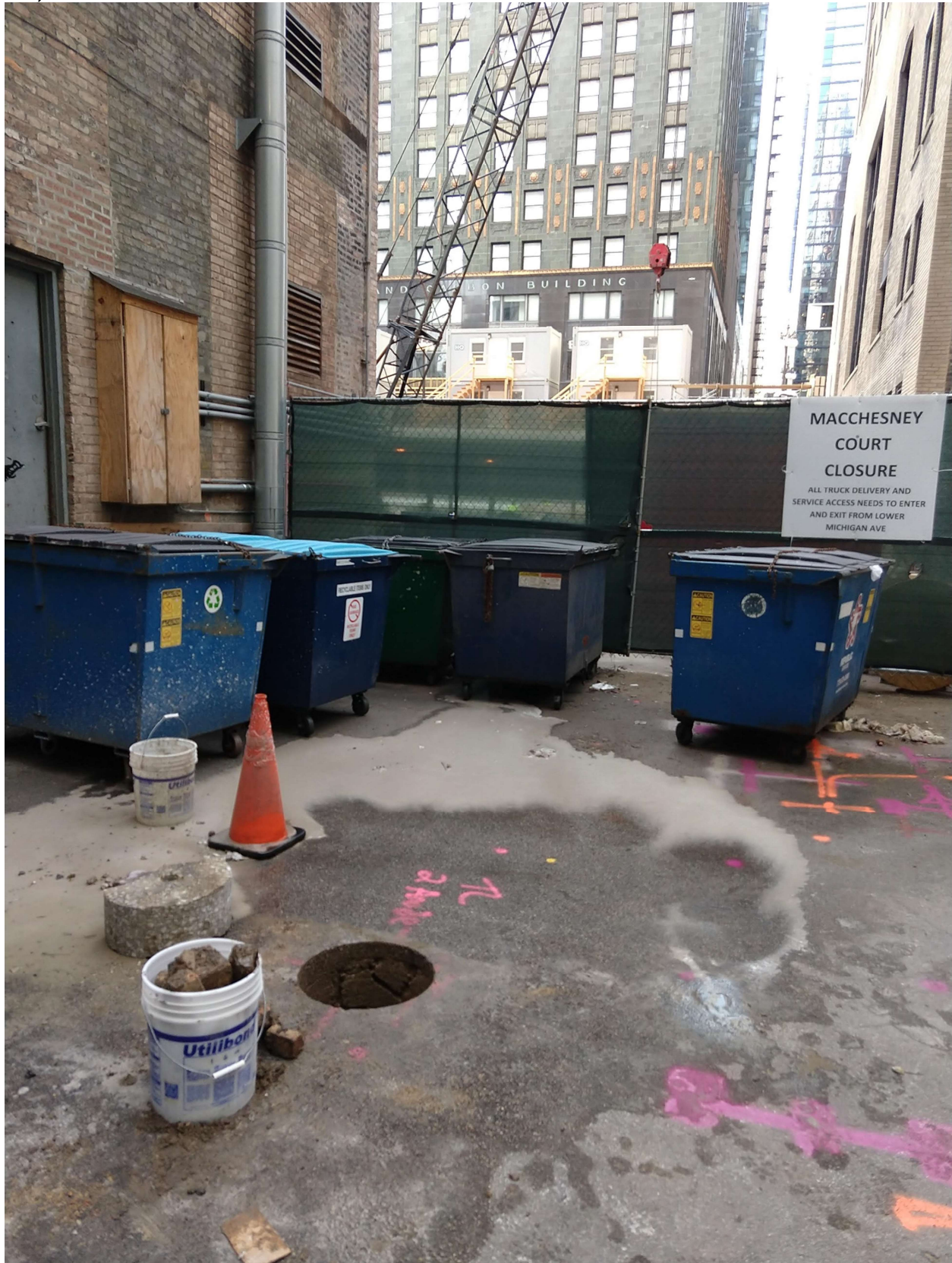
PICTURE 1: VIEW OF THE CORROSION PROTECTION EXCAVATION AT 310 N MAC CHESNEY CT., LOOKING SOUTH TOWARDS E. WACKER PL.
