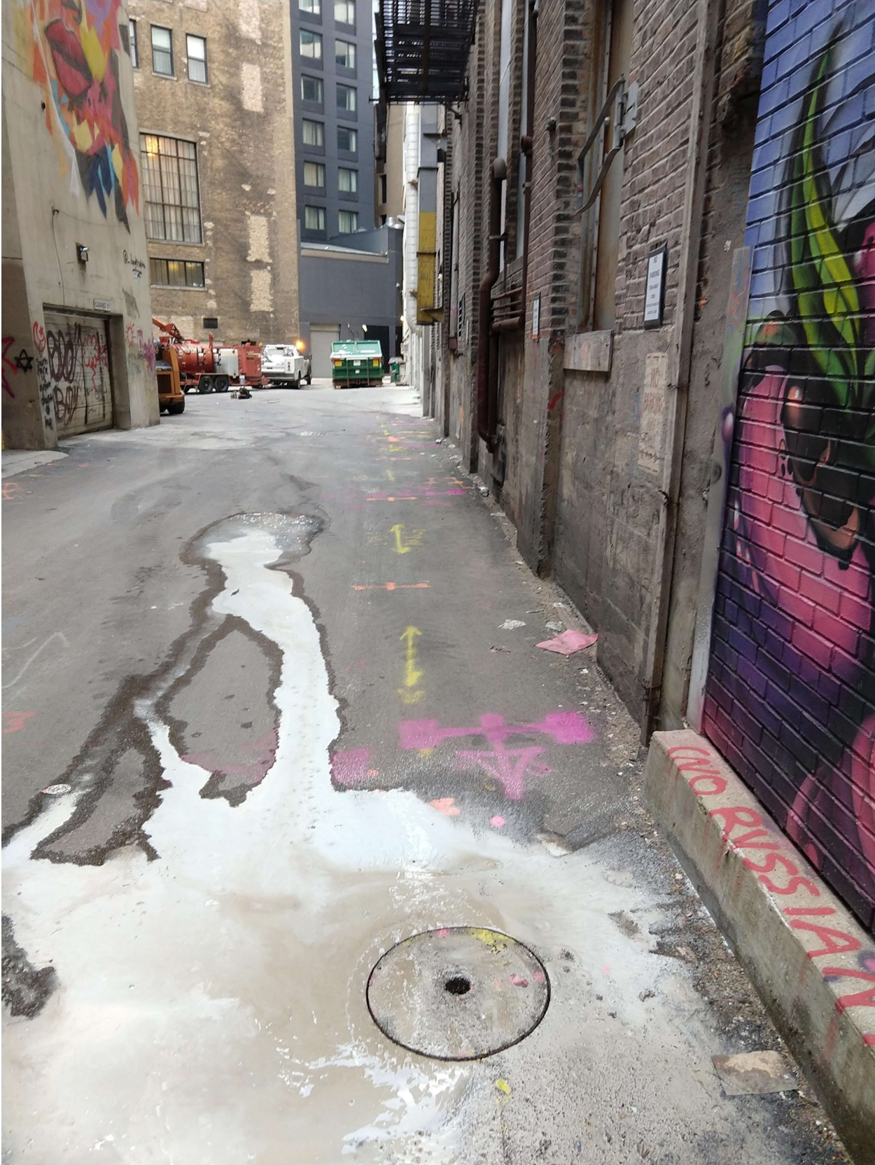
PICTURE 2: VIEW OF THE CORROSION PROTECTION EXCAVATION AT 336 N MAC CHESNEY CT., LOOKING SOUTHEAST TOWARDS E. WACKER PL.
