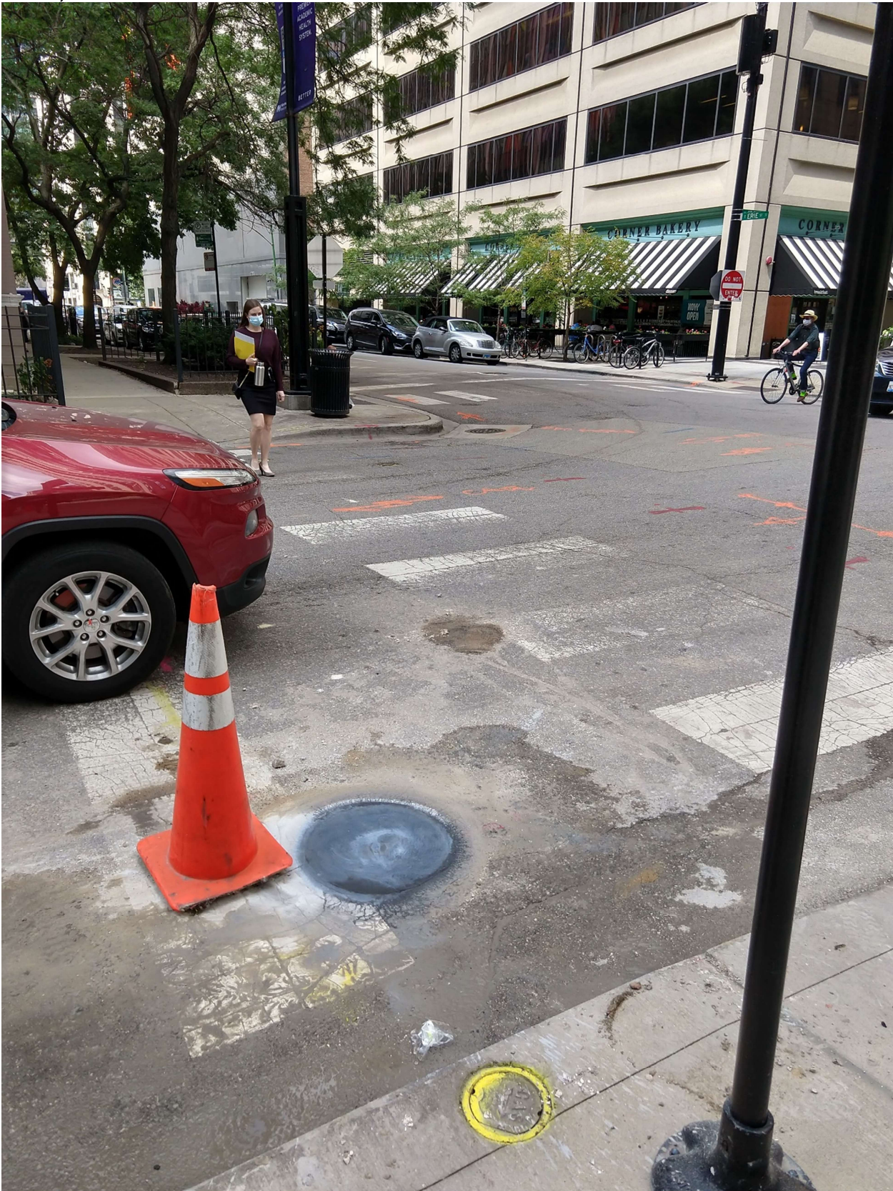
PICTURE 1: VIEW OF THE COMPLETED CORROSION PROTECTION EXCAVATION AT 633 N ST. CLAIR, LOOKING NORTHWEST TOWARDS ERIE ST.
