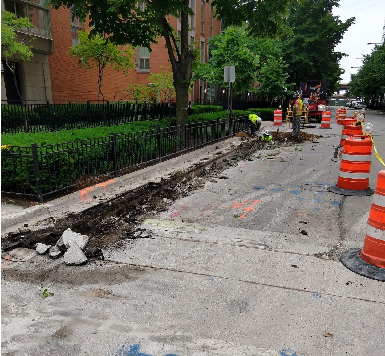
PICTURE 2: VIEW OF THE TRENCH EXCAVATION AT THE INTERSECTION OF MCCLURG CT AND NORTH WATER ST (LOOKING EAST)
