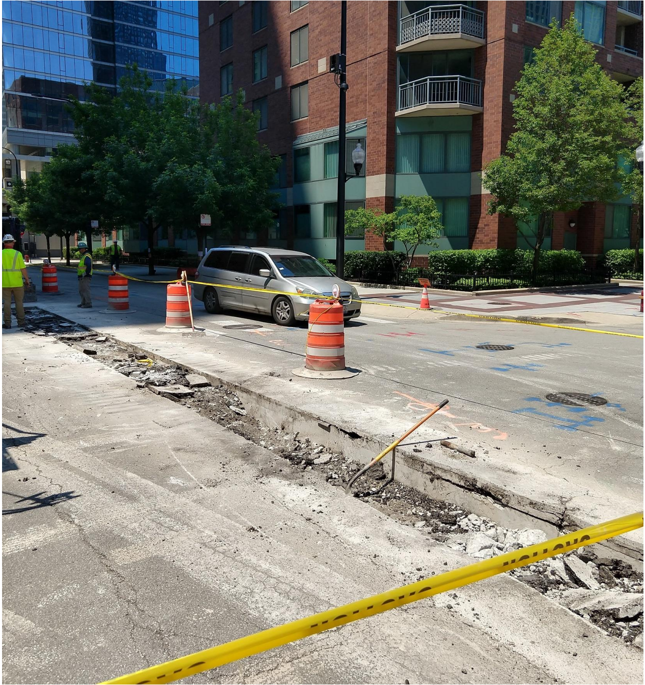
PICTURE 1: VIEW OF THE TRENCH EXCAVATION AT THE INTERSECTION OF MCCLURG CT AND NORTH WATER ST (LOOKING NORTHWEST).
