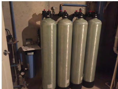
Whole-house filters like the one above have been installed in affected homes.
