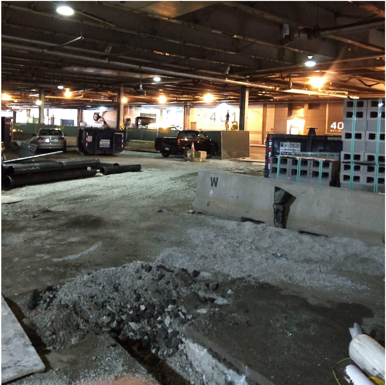
PICTURE 1: VIEW OF THE CORROSION PROTECTION EXCAVATION IN THE LOWER LEVEL OF 435 N. MICHIGAN.
