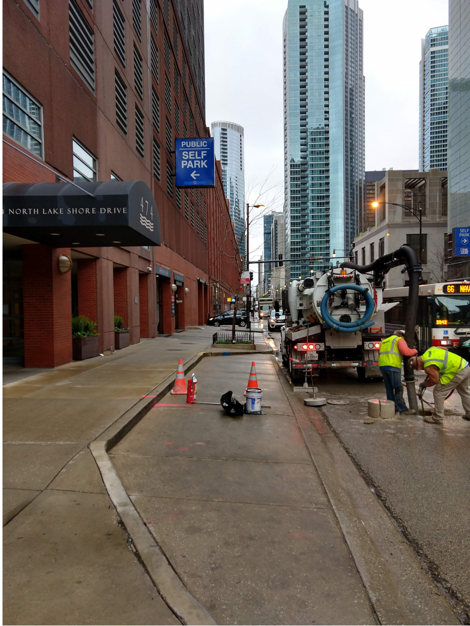
PICTURE 1: VIEW OF THE EAST KEYHOLE OPENING, 1 OF 3, EXCAVATED TO CUT-OFF INACTIVE SERVICE ON AN EXISTING GAS MAIN
