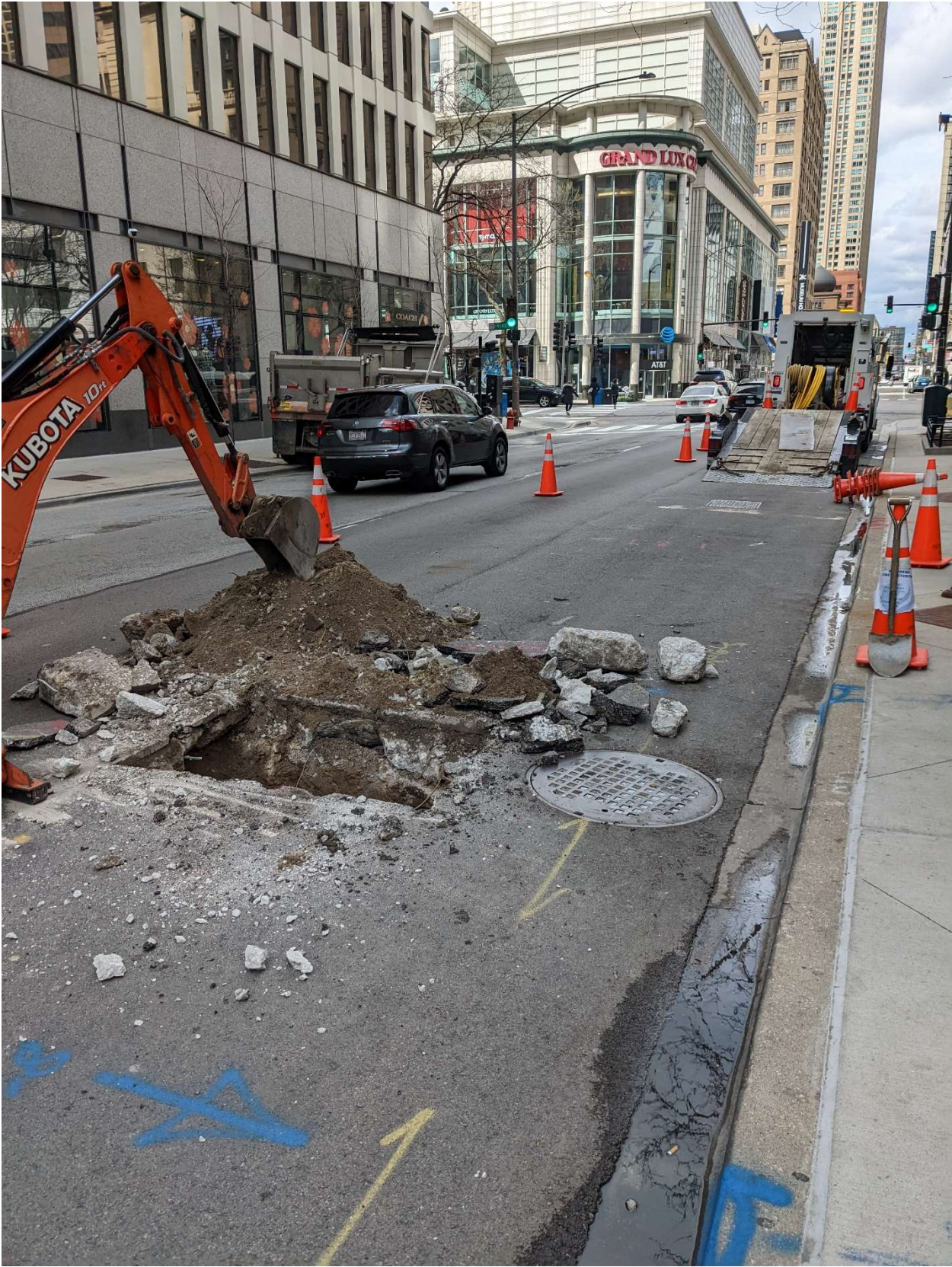
PICTURE 1: VIEW OF THE COMPLETED CORROSION PROTECTION EXCAVATION AT 100-163 E ONTARIO ST.
