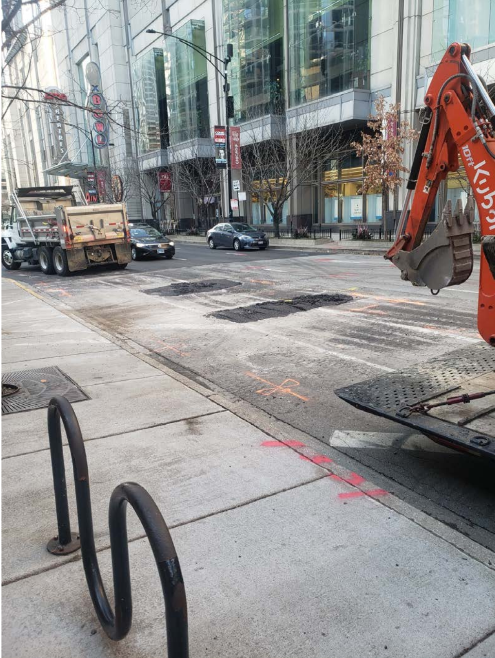
PICTURE 1: VIEW (LOOKING NW) OF THE TWO AREAS OF PAVEMENT REMOVAL AS PAVEMENT REPAIRS ARE BEING COMPLETED.
