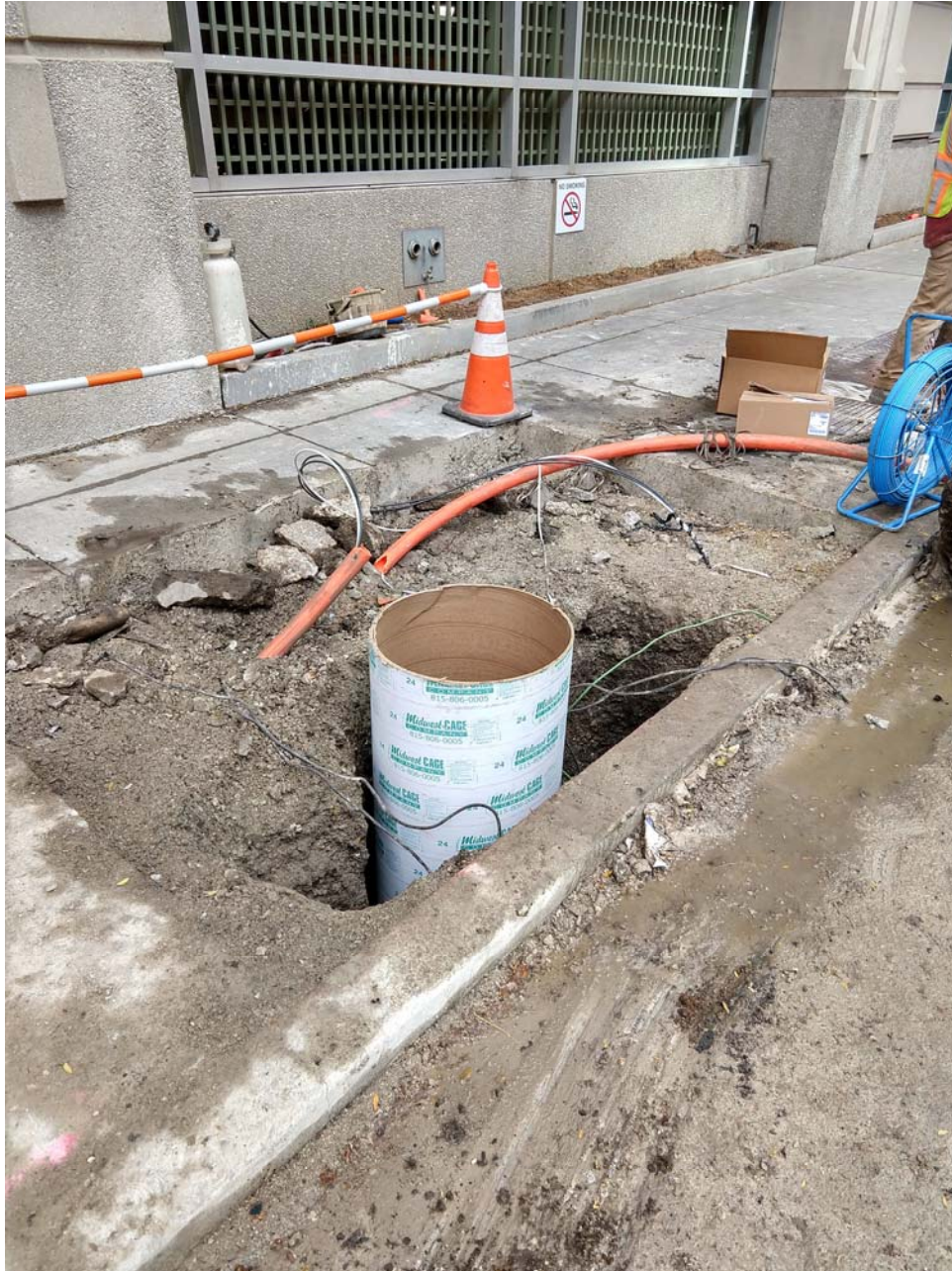
Eastern sidewalk excavation on northern sidewalk of E. Ontario Street after removal of the original foundation with excavation for new utility pole foundation complete.
