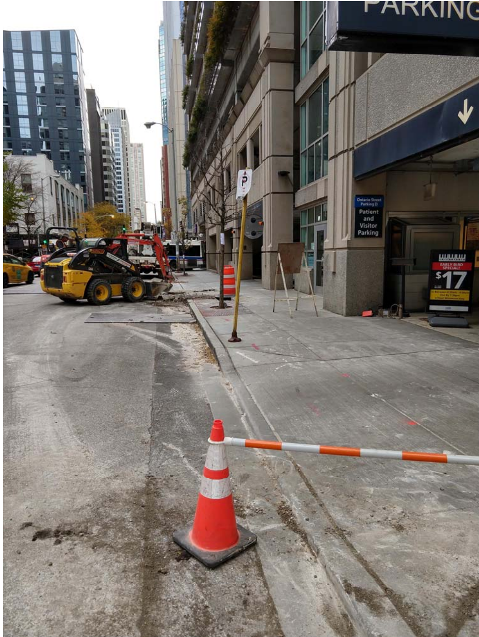
Looking west from the eastern sidewalk excavation at the western sidewalk excavation location and completed trench excavation.
