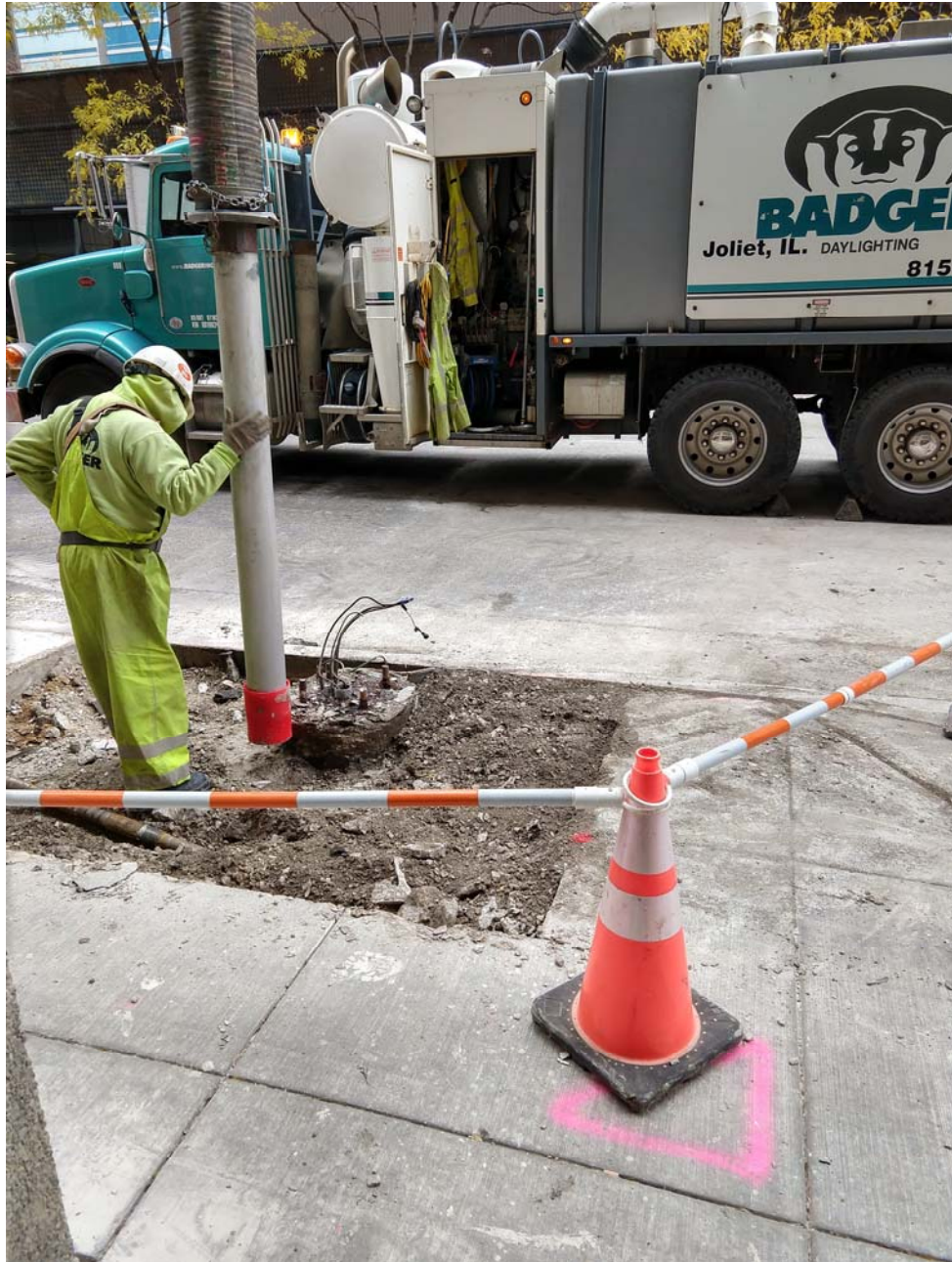
Eastern excavation in northern sidewalk on E. Ontario Street prior to removal of the existing foundation.
