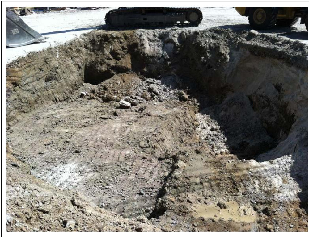
Photo No. 6: South side of excavation with varying bottom depths evident on right side of photograph.
