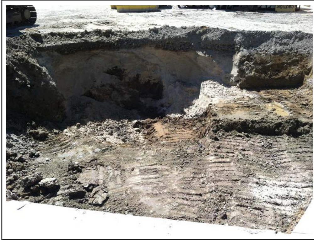
Photo No. 5: West side of excavation in deepest portion with backfill from former UST removal visible.
