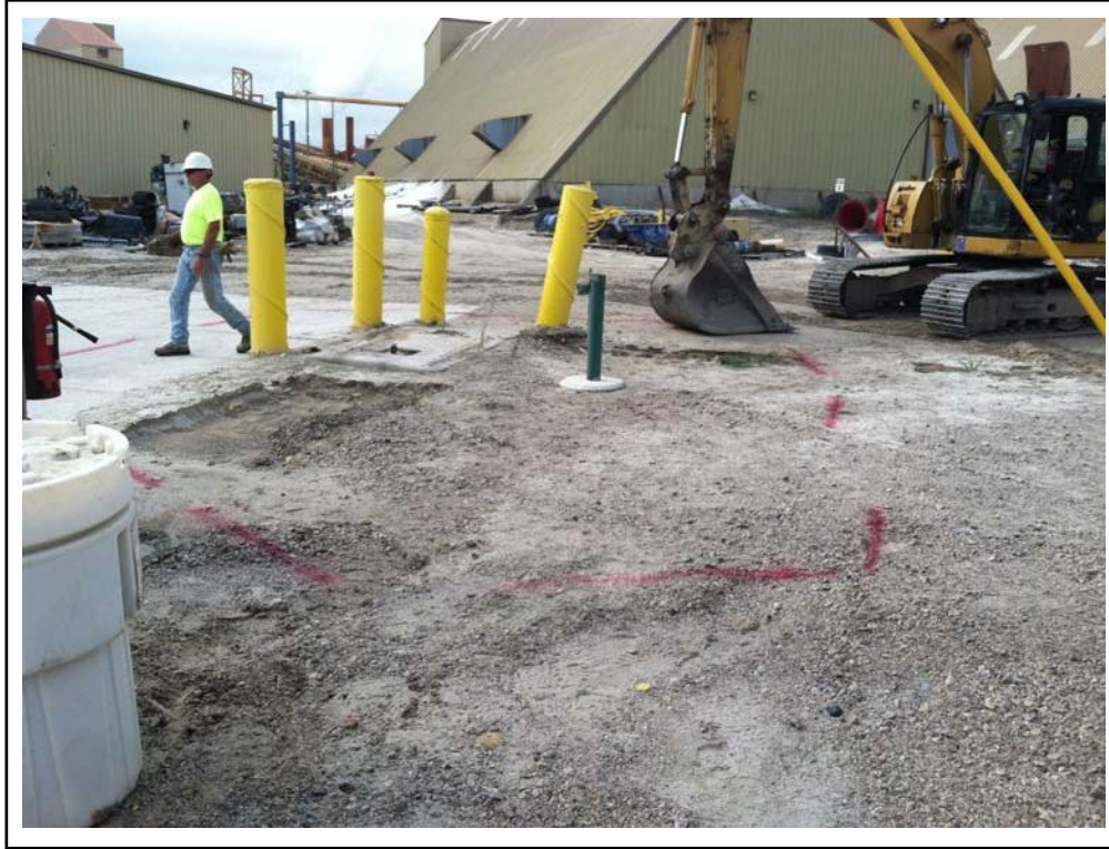
Photo No. 1: AST already moved prior to excavating and monitoring well MW-19 prior to abandonment.
