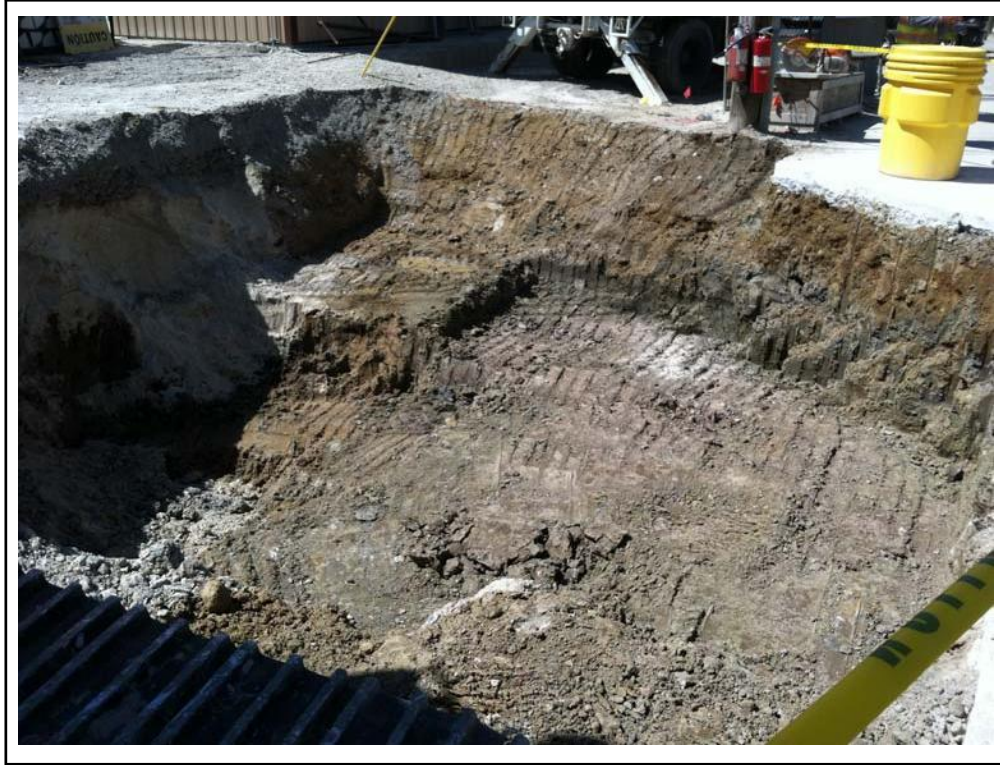
Photo No. 3: Northwest side of excavation with varying bottom depths.
