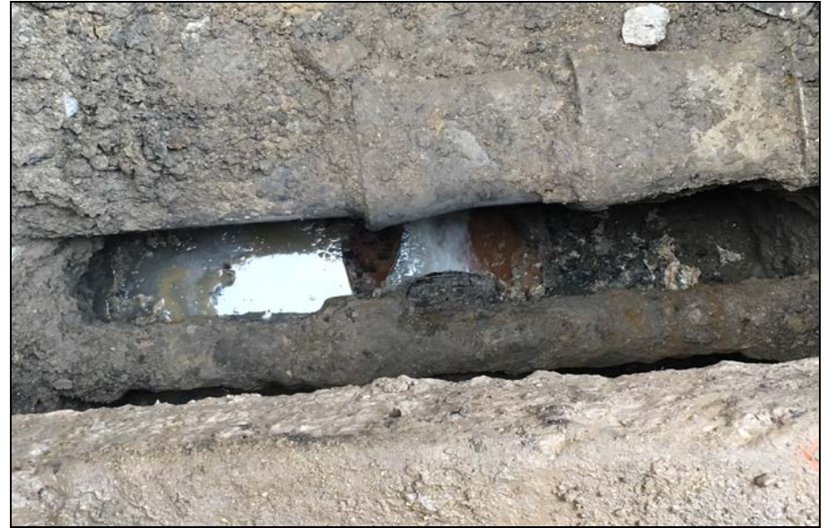
Photo 2: View facing south of sewer line break directly below curb (foreground)
