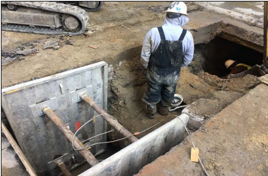
Photo 3: View facing northwest of excavation on Illinois Street (sewer runs underneath 3 foot water main worker is standing on)
