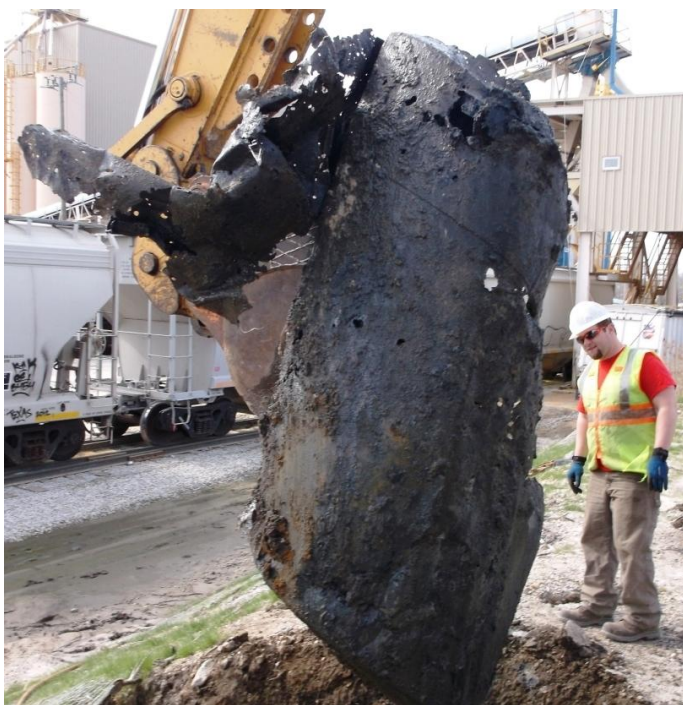
Workers remove a leaky underground storage tank from Illinois Railway property in Wedron. U.S. EPA engineers are looking at several possible sources of well water contamination in the town.
