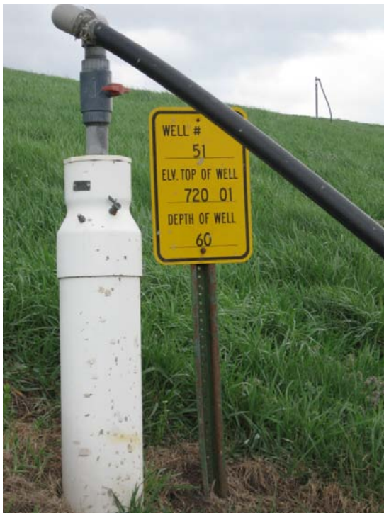
Figure 3 SSL Methane Gas Collection Well
