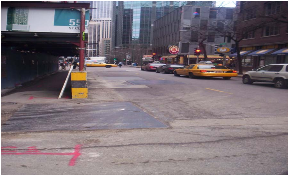
Photo 1: Taken south to north. Shows the locations of the completed test pits and planned trench along St. Clair prior to beginning work.
