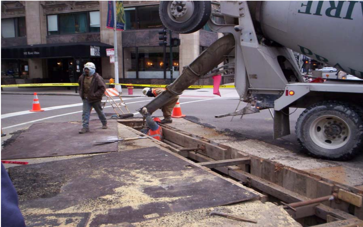
Photo 11: Taken south to north. Shows the pouring of concrete into the trench over the conduit shells.
