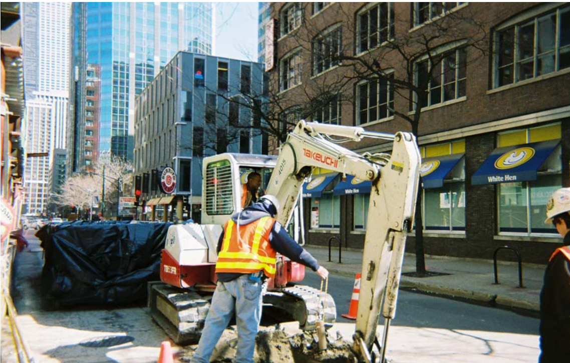
Photo 6: Taken west to east. Shows radiation screening of soil using the "Bucket Survey Method."
