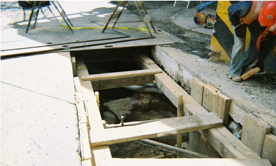
Photo 8: Taken north to south. Shows utilities encountered at the south end of the excavation prior to turning into the alley.
