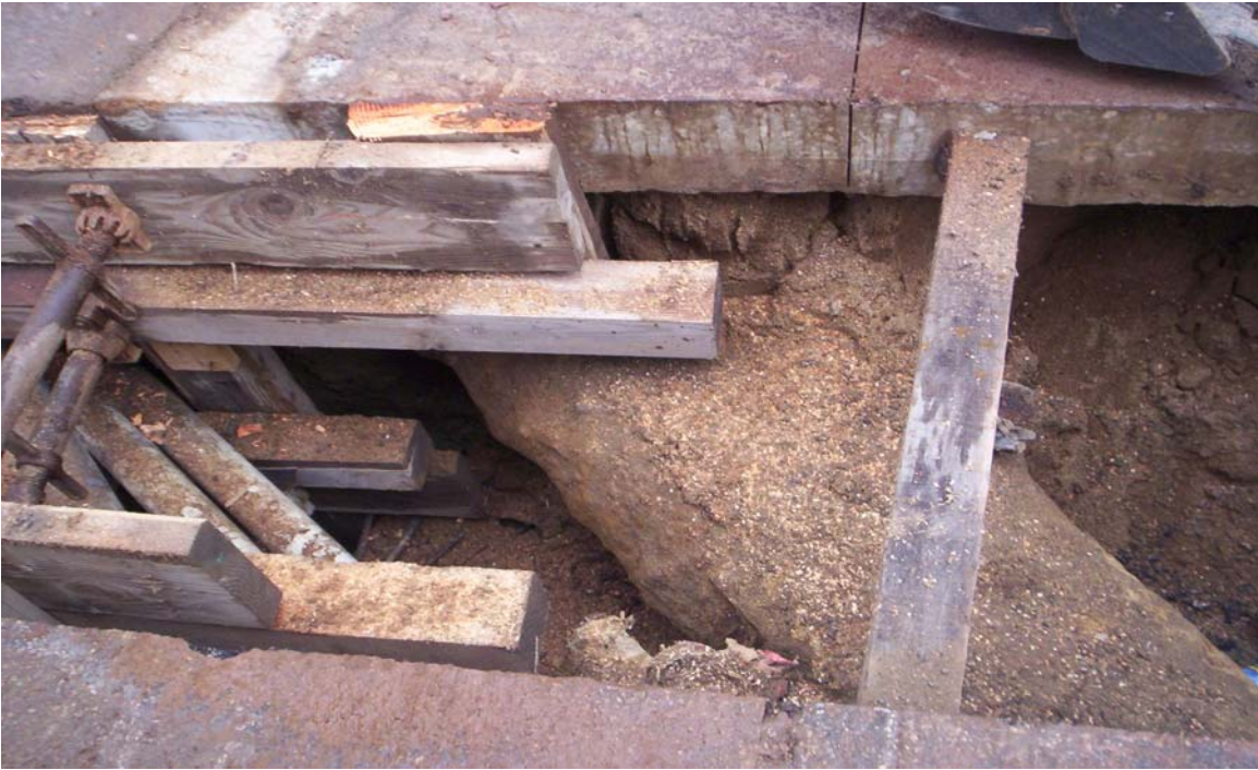
Photo 7: Taken south to north. Shows utilities encountered at the north end of the excavation.
