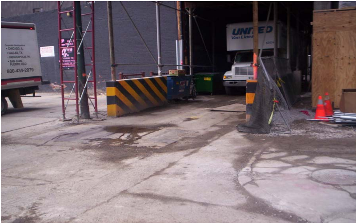
Photo 2: Taken east to west. Shows south end of planned trench along alley prior to beginning work.
