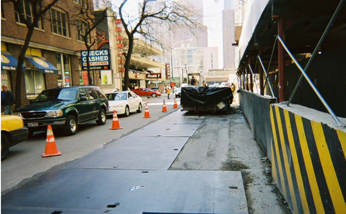
Photo 17: Taken north to south. Shows steel plates placed over the top of the completed trench along St. Clair.
