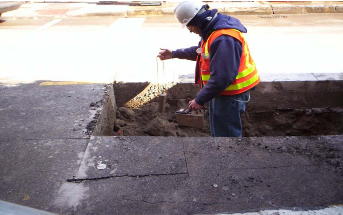
Photo 5: Taken west to east. Shows radiation screening of soil in trench during excavation.
