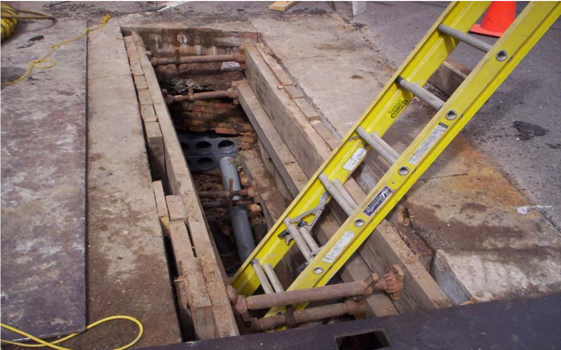
Photo 9: Taken east to west. Shows six lines of conduit shells running into the manhole on north end of excavation.
