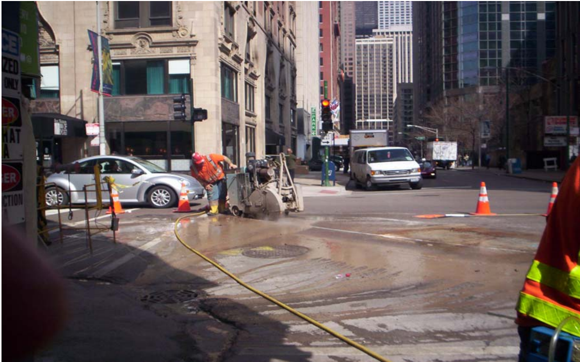
Photo 3: Taken south to north. Shows saw cutting through the pavement at the north end of the trench.
