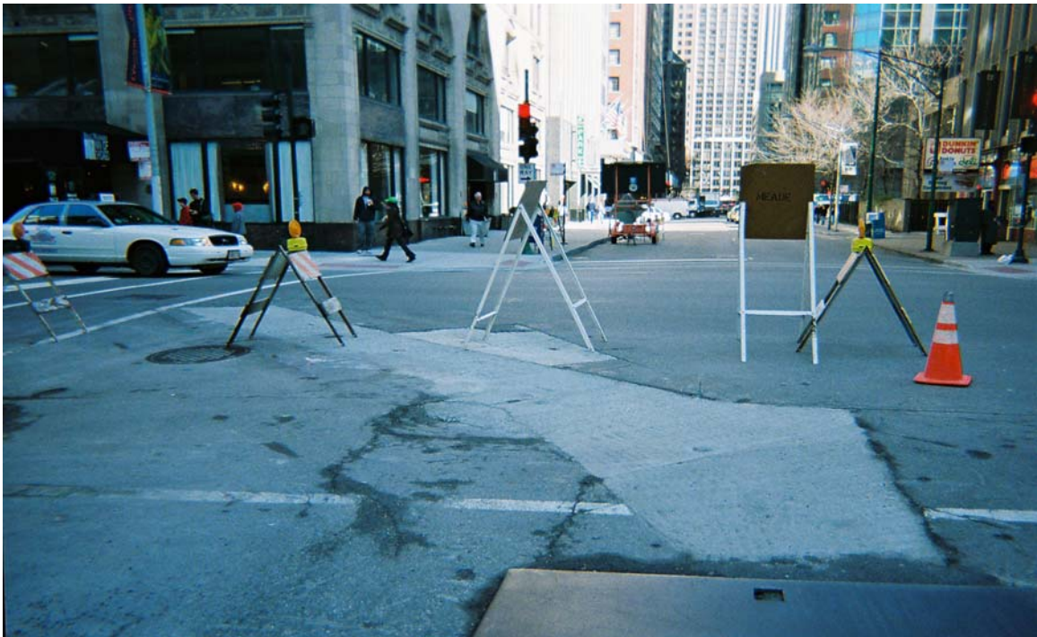
Photo 16: Taken south to north. Shows location of the north end of the trench after it has been backfilled and the concrete poured.
