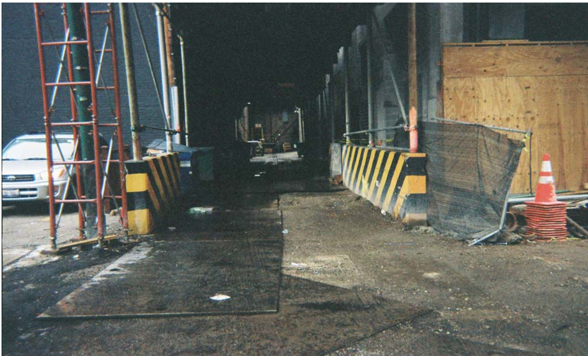
Photo 18: Taken east to west. Shows steel plates over the top of the south end of the completed trench in the alley.
