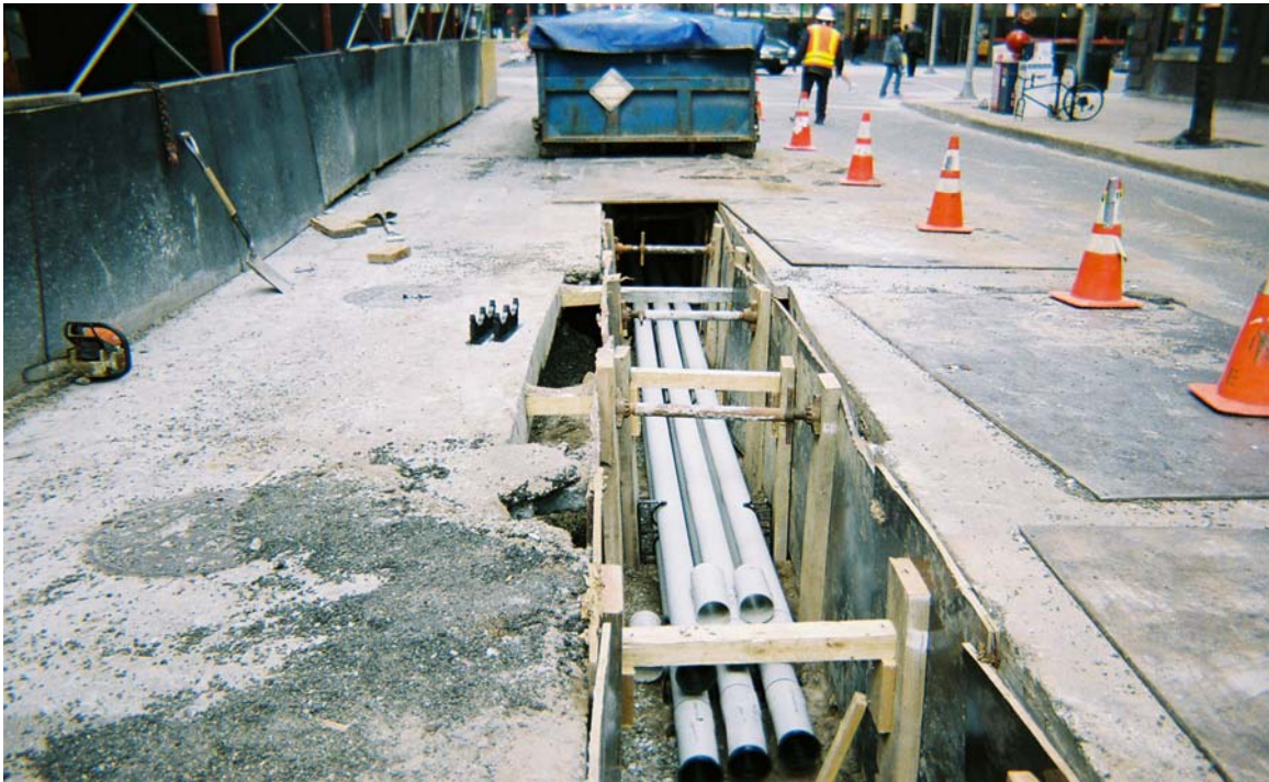
Photo 15: Taken south to north. Shows conduit shells in the trench along St. Clair.
