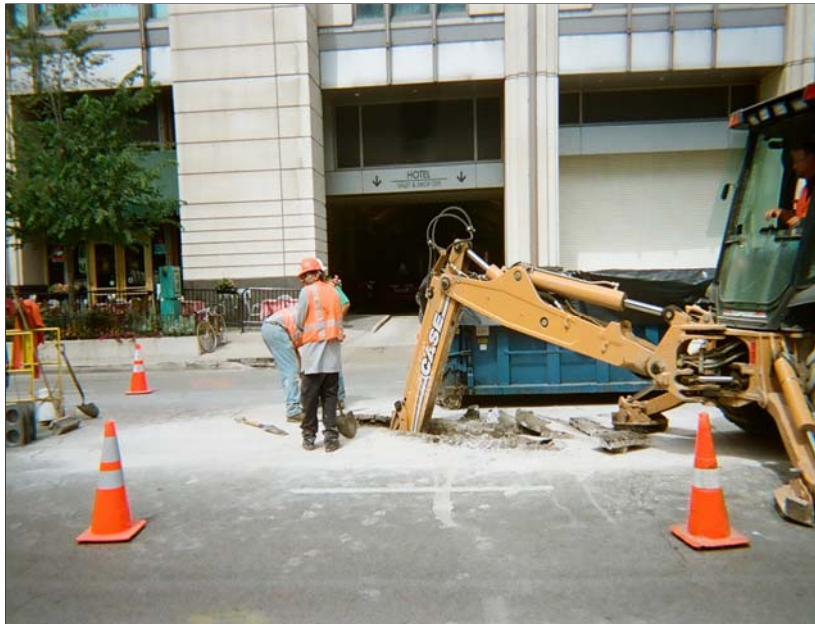
Photo 4: Taken south to north. Beginning of trench excavation using backhoe. Shows narrow width of trench.
