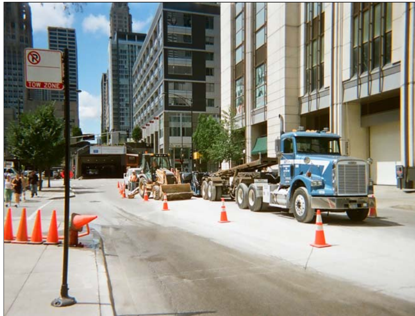
Photo 1: Taken east to west. Shows planned trench run along Illinois Street prior to the beginning of excavation.
