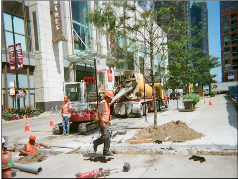
Photo 9: Taken west to east. Completed section of trench running north and south across the sidewalk to the tie-in location.
