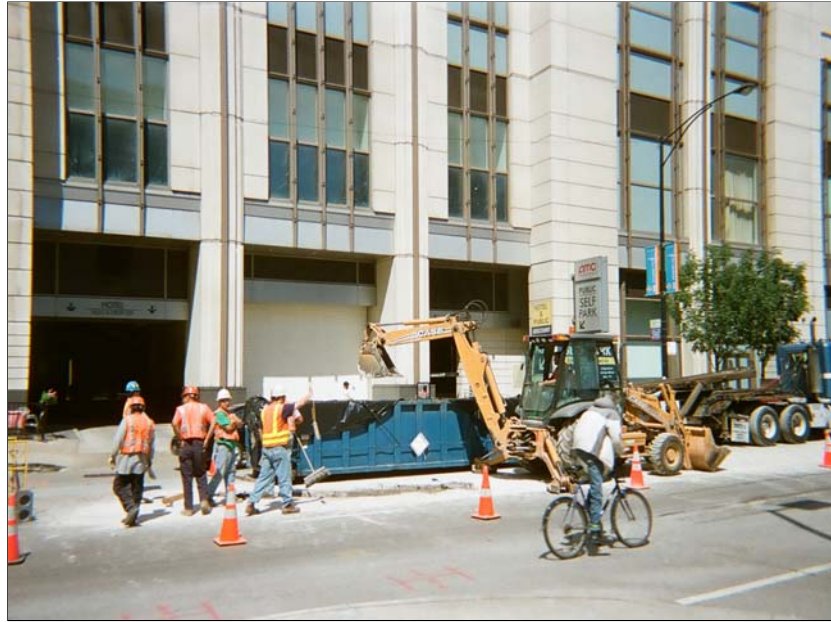
Photo 5: Taken south to north. Screening of trench soils for radiation from the surface during excavation.
